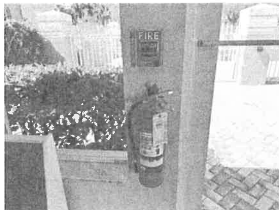
VIEW OF TYPICAL FIRE EXTINGUISHER
