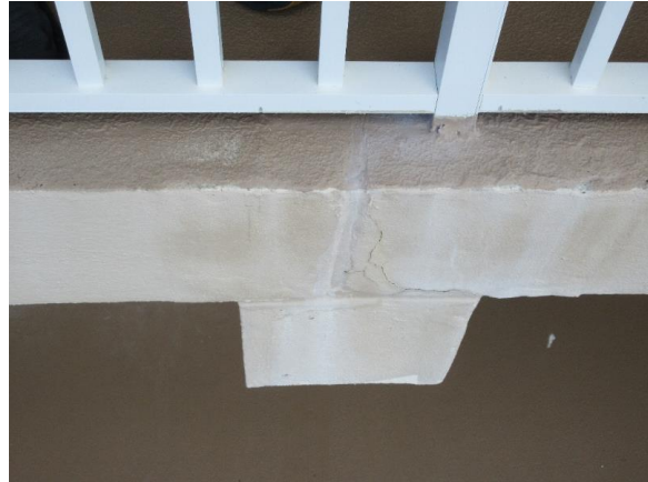
Typical Efflorescence and Crack/Spall at Slab Edge
