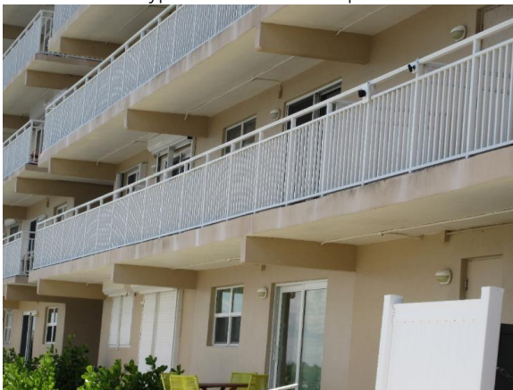
Typical Efflorescence at Slab Edge
