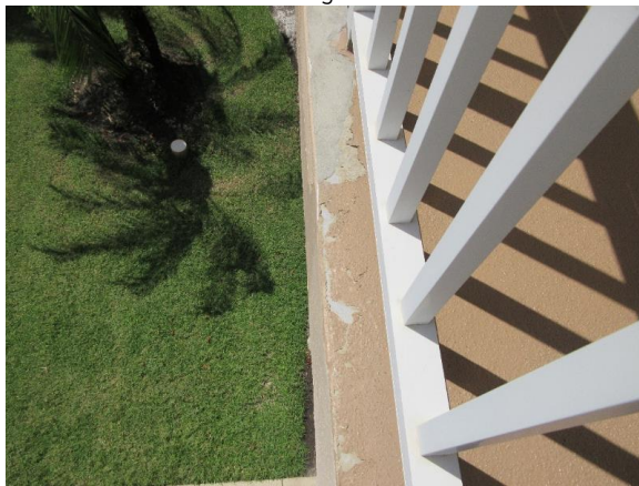
Typical Failed Waterproofing
