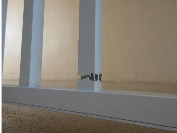
Damage to Railing Pickets
