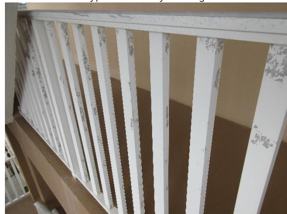
Wear on Railing Coating
