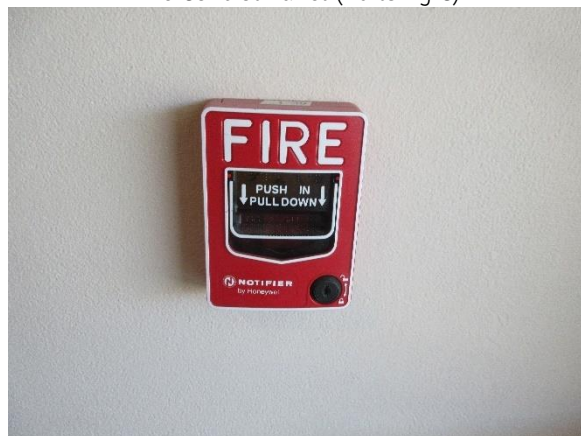
Typical Pull Station
