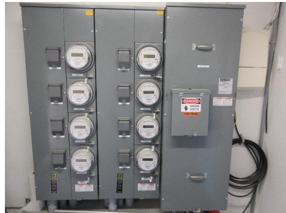
Meter Bank Building C
