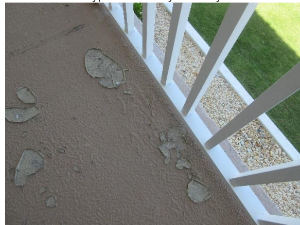
Typical Failed Waterproofing
