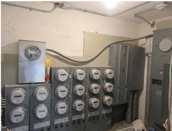
Typical Electrical Meter Bank (Buildings A, B, D & E)
