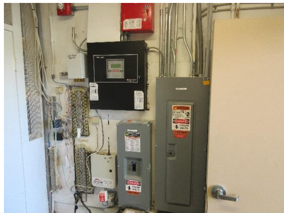
Fire Control Panel (Building C)
