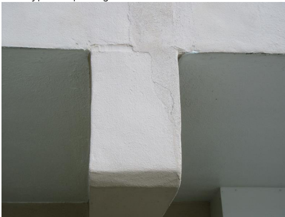
Typical Failed Prev Repair
