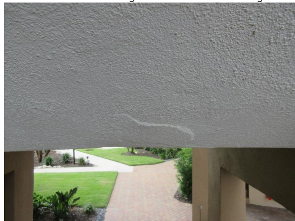
Spalling Concrete at Stairs
