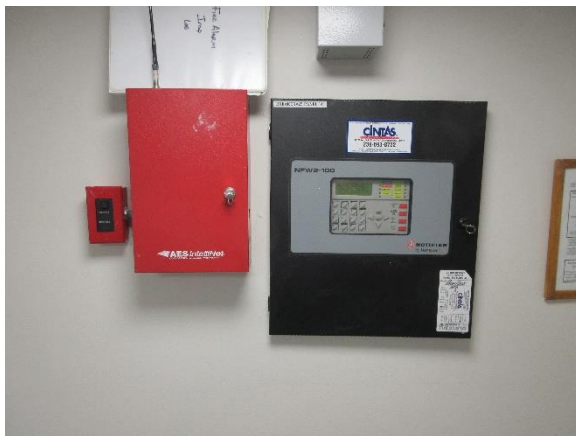
Fire Control Panel (Buildings A, B, D & E)
