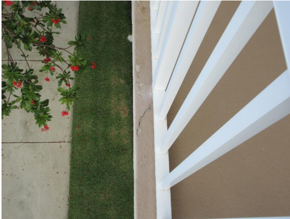
Typical Spalling Concrete at Rail Post Pocket
