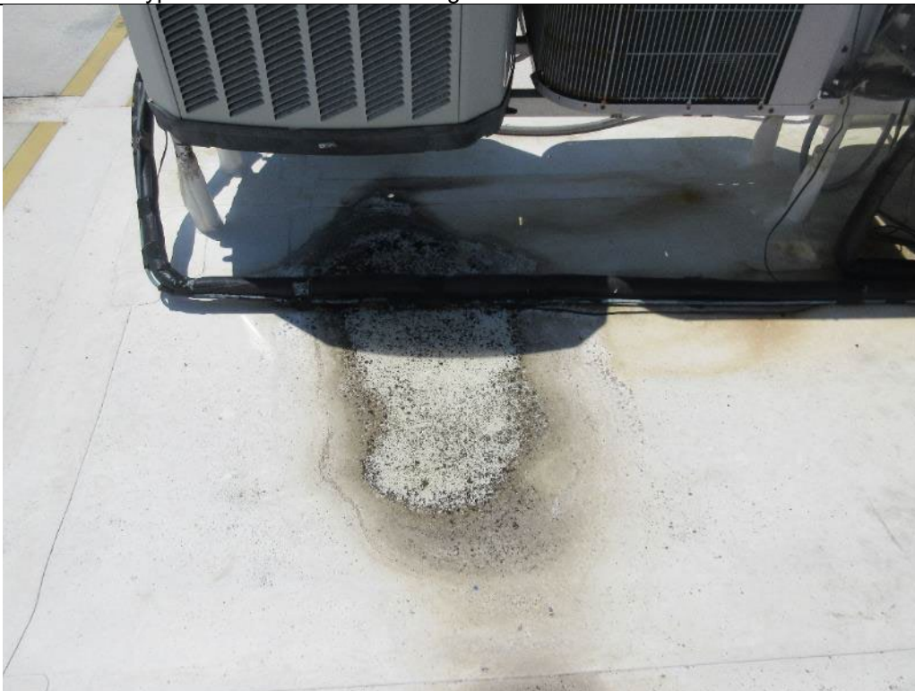
Photo 95. Isolated Ponding at Roof Building E
