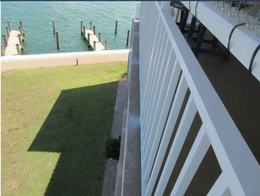
Photo 43. Typical Failed Waterproofing and Efflorescence at Slab Edge C402
