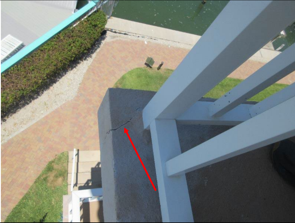
Photo 90. Cracked and Spalled Slab Edge E404
