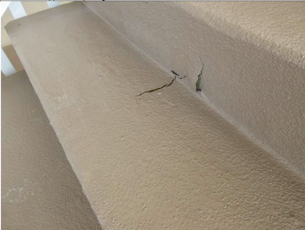
Photo 8. Failed Waterproofing Coating at Stairs
