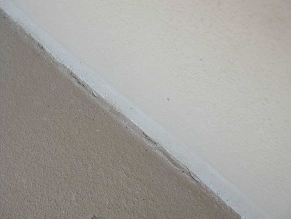
Photo 46. Typical Failed Floor to Wall Transition Sealant and Waterproofing
