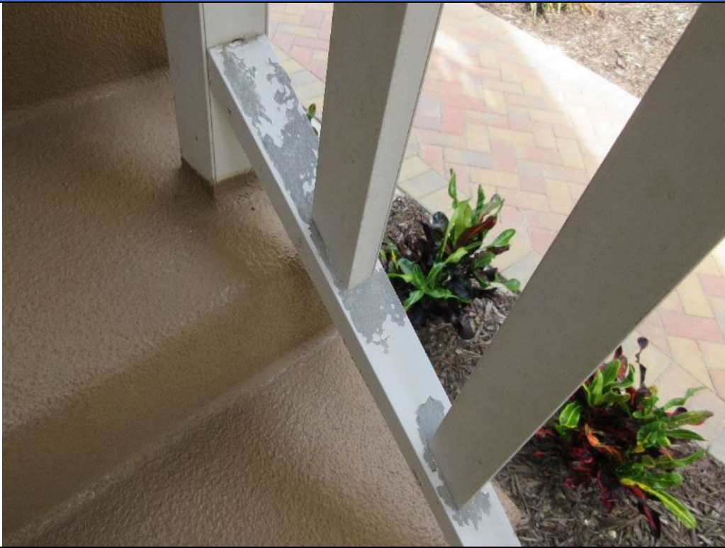
Photo 55. Typical Failed Railing Coating Building D
