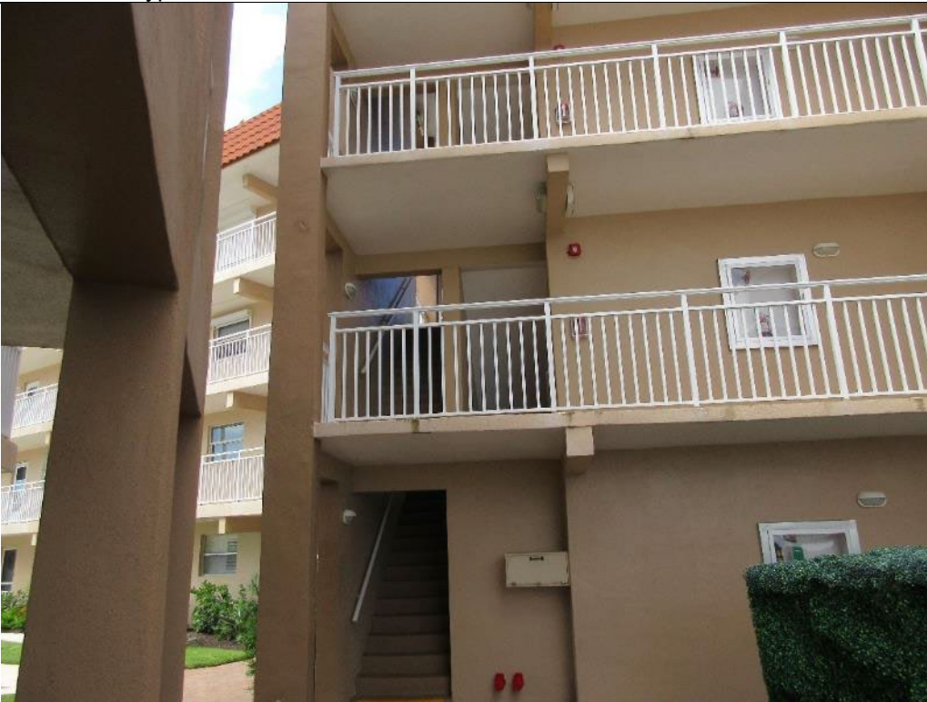
Photo 50. Typical Stairs Building C with Staining and Efflorescence at Slab Edges
