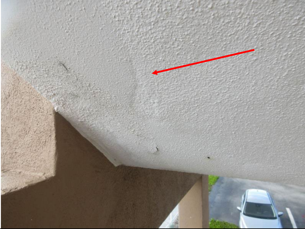
Photo 7. Apparent Spalling Concrete at Stairs
