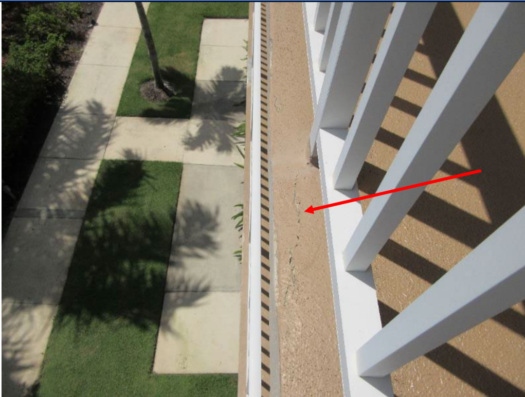
Photo 79. Spalling Concrete and Crack at Slab Edge Near Post Pocket E301
