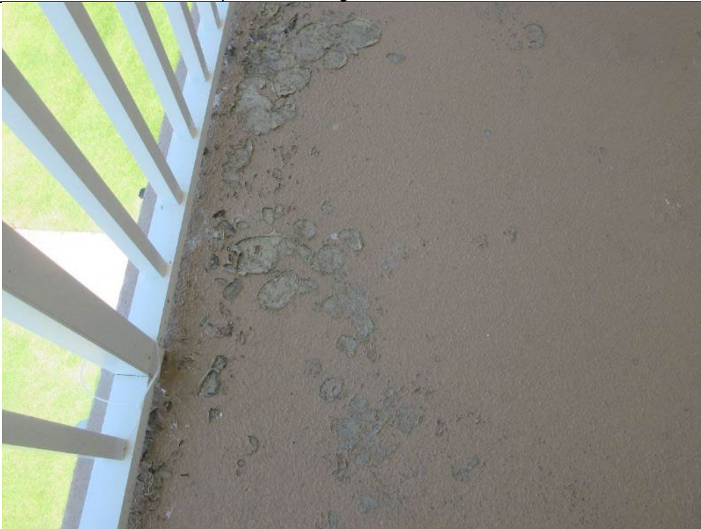
Photo 91. Typical Failed Waterproofing E303
