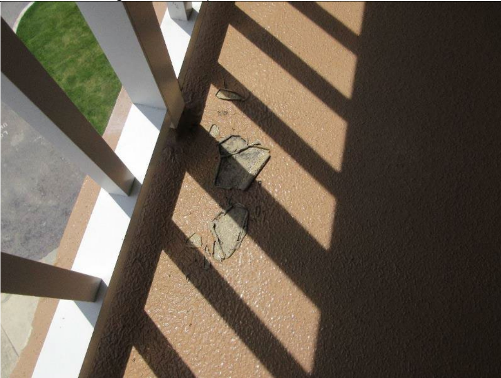
Photo 78. Typical Failed Deck Coating Building E
