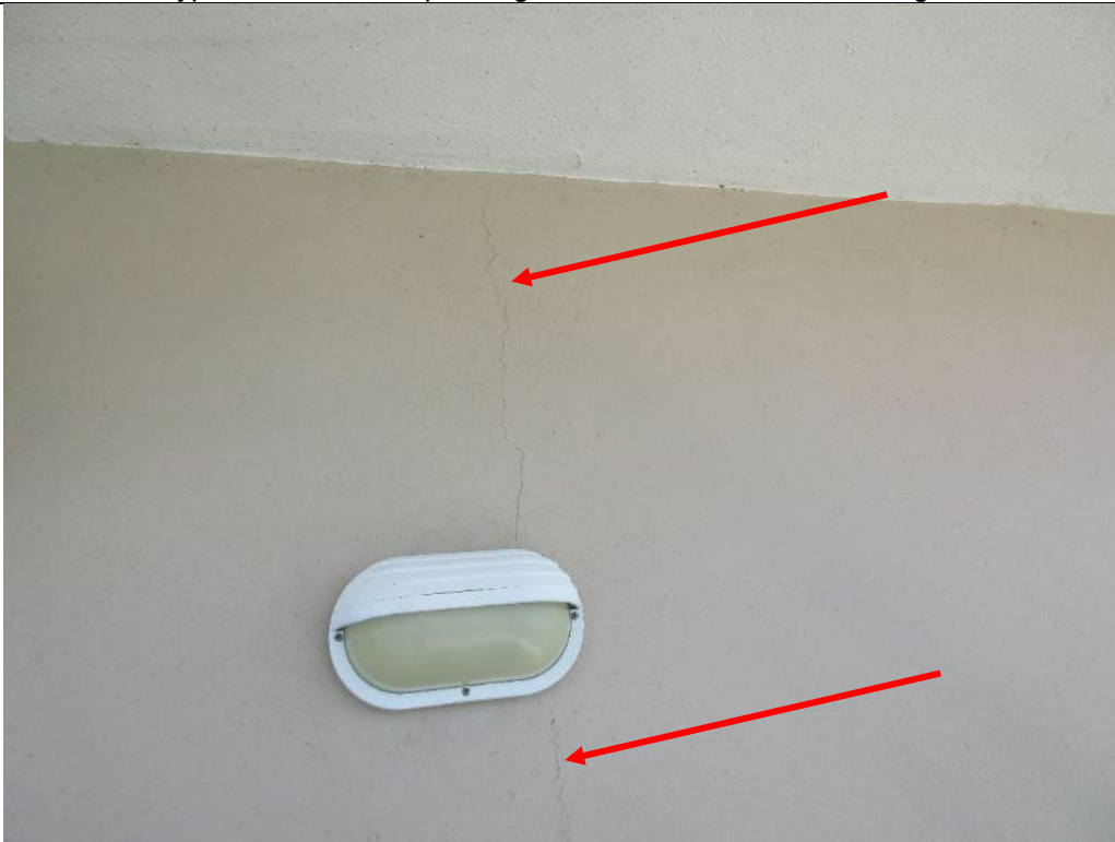
Photo 44. Crack at Stucco Wall C402
