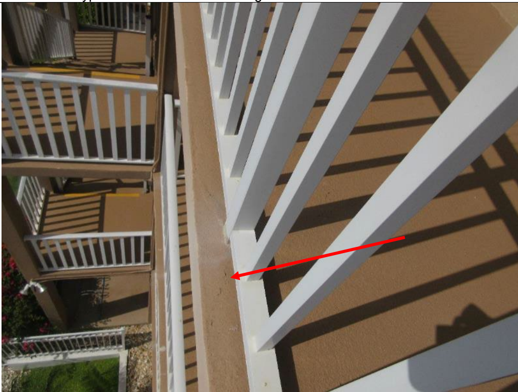
Photo 16. Apparent Concrete Spall at Post Pocket A401
