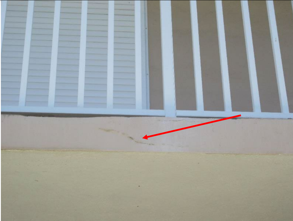
Photo 85. Spalling Concrete and Crack at Slab Edge E202
