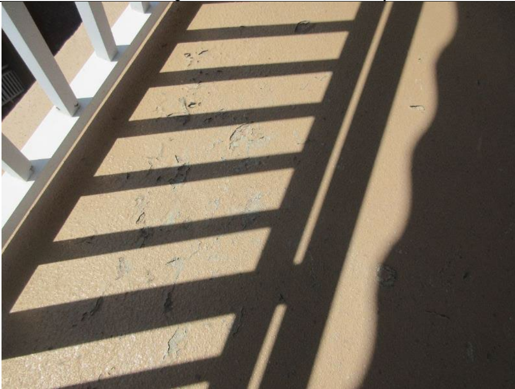
Photo 42. Typical Failed Waterproofing C401
