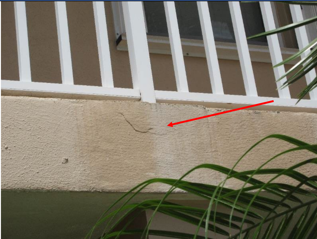
Photo 61. Spall at Slab Edge Railing Post Near D102
