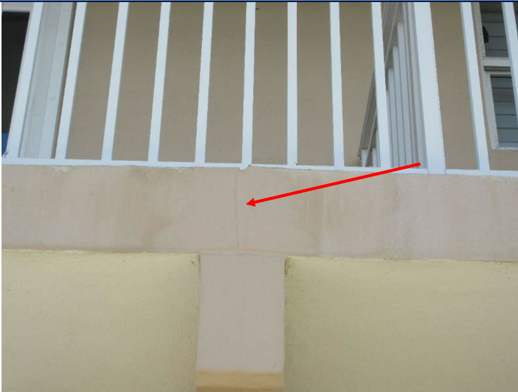
Photo 25. Crack at Slab Edge B201
