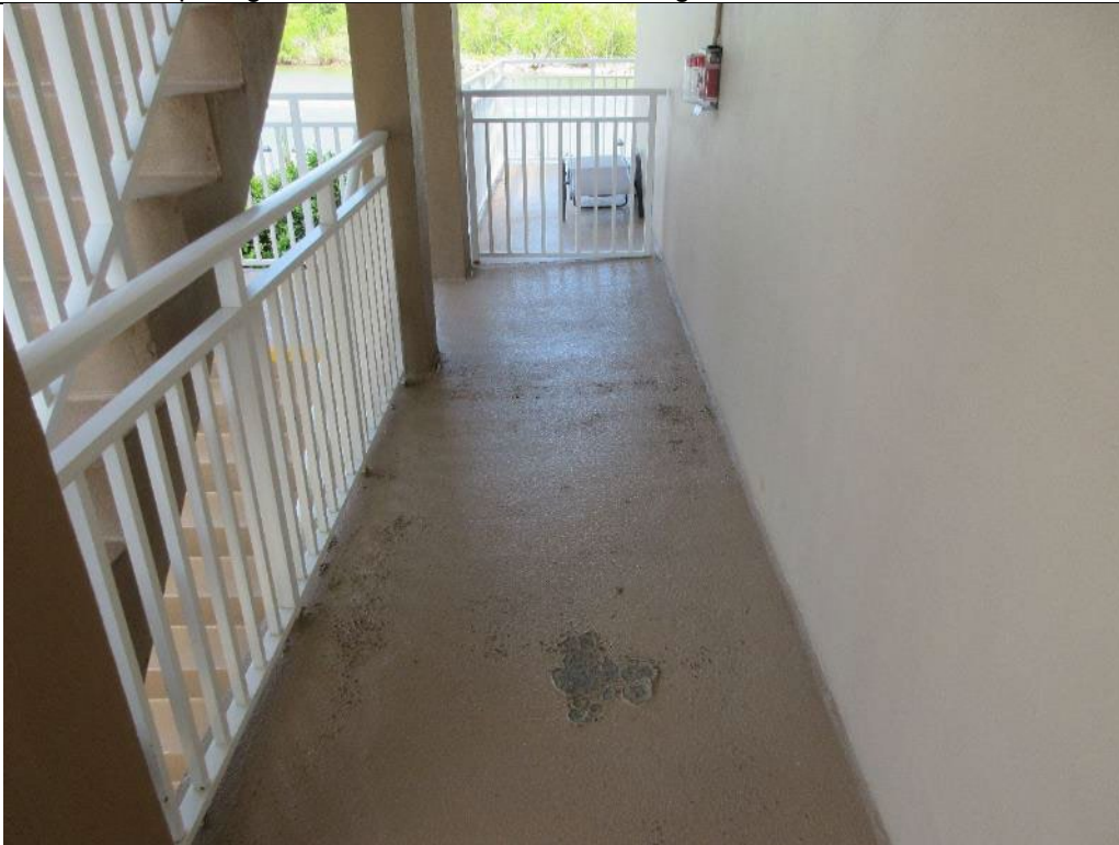
Photo 82. Typical Failed Waterproofing Building E
