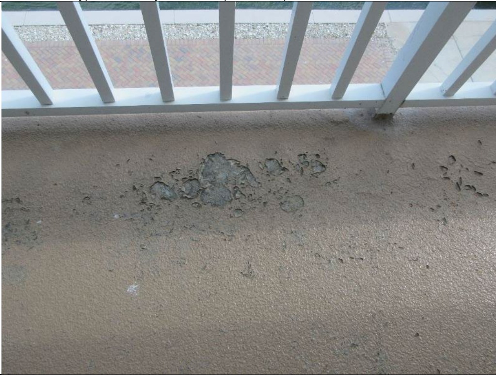
Photo 14. Close-Up Failed Deck Coating A301 (Typical)
