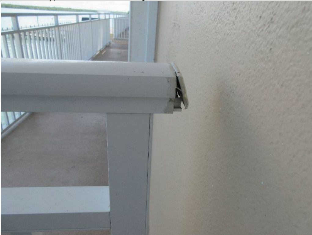
Photo 34. Damaged Rail Top Cap at B302
