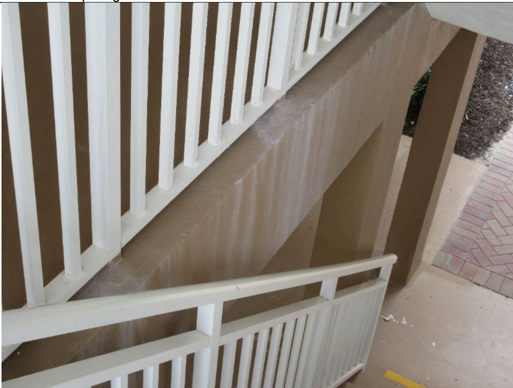
Photo 32. Efflorescence at Slab Edge Near Stairs
