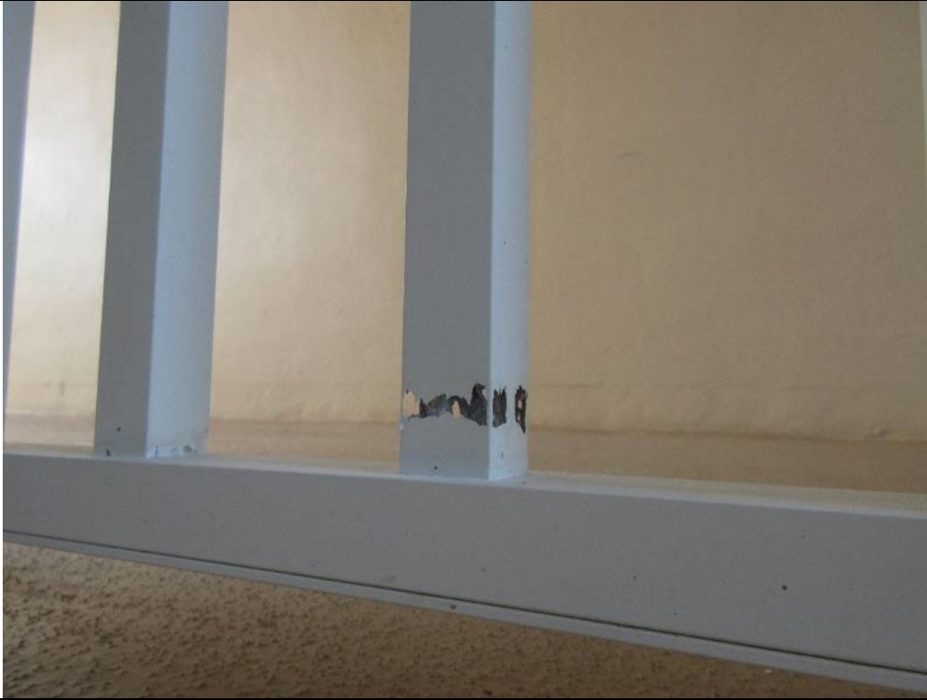
Photo 63. Typical Damaged Railing Picket at Attachment
