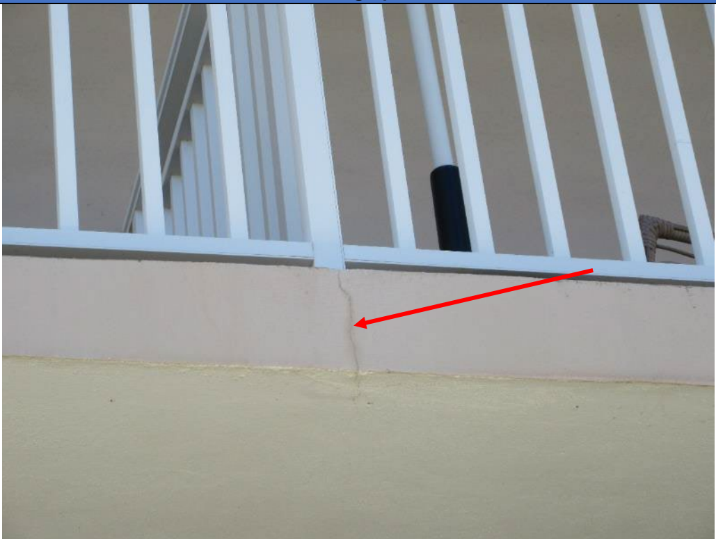
Photo 87. Crack at Slab Edge First Floor Lobby
