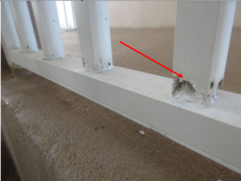
Photo 12. Railing Picket Deterioration at Attachment to Bottom Rail
