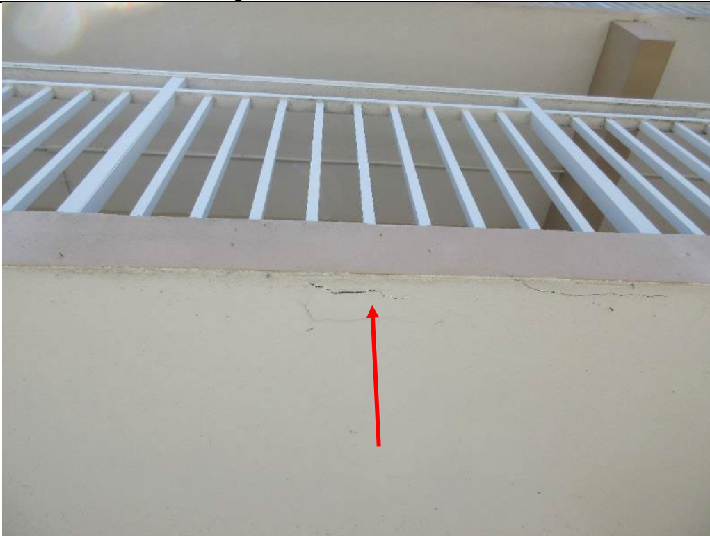
Photo 18. Slab Edge Crack and Spall at A201
