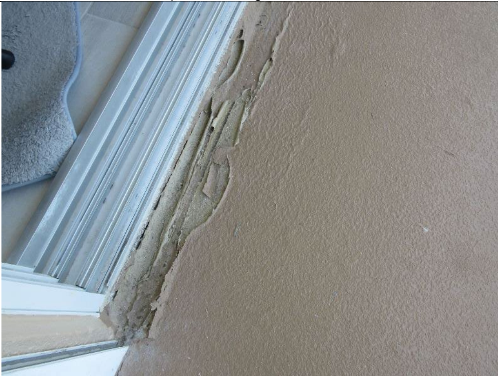
Photo 66. Failed Waterproofing Coating at D302
