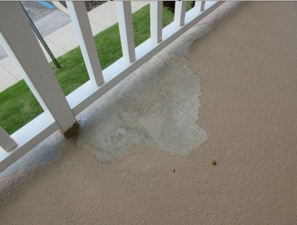
Photo 10. Failed Deck Coating
