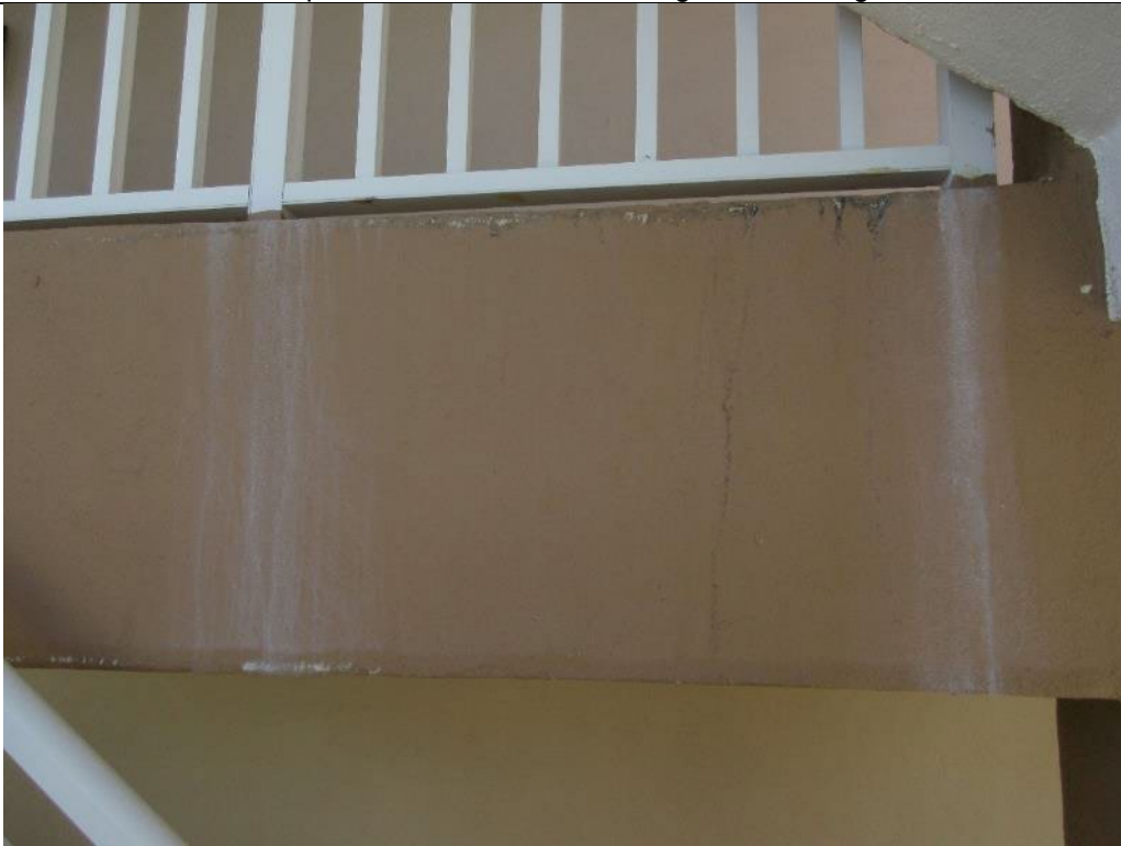
Photo 84. Typical Efflorescence at Railing Post
