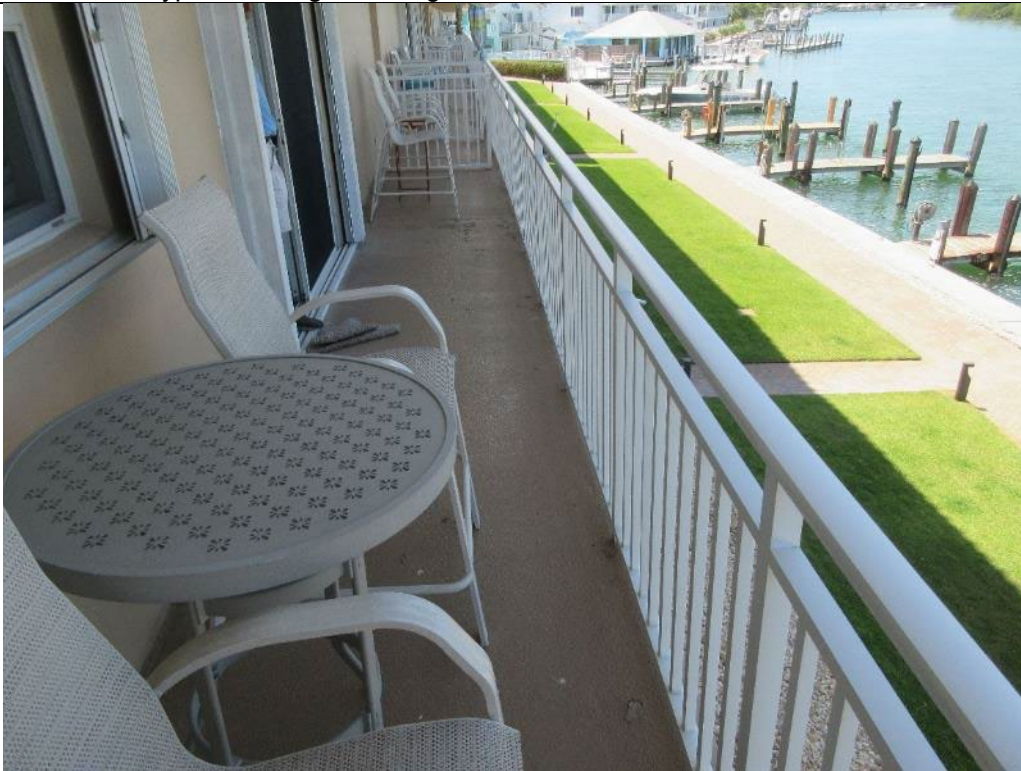
Photo 64. Balcony Overview D202 with Failed Waterproofing Typical
