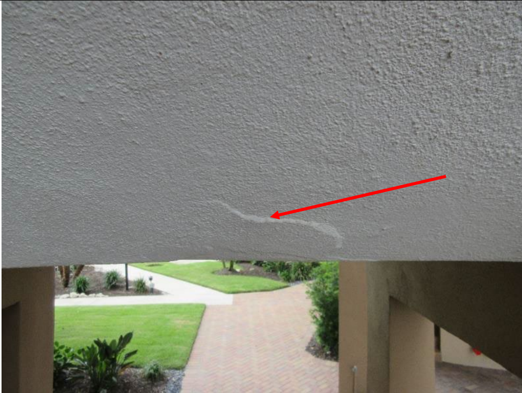
Photo 31. Spalling Concrete at West Stair Level 1
