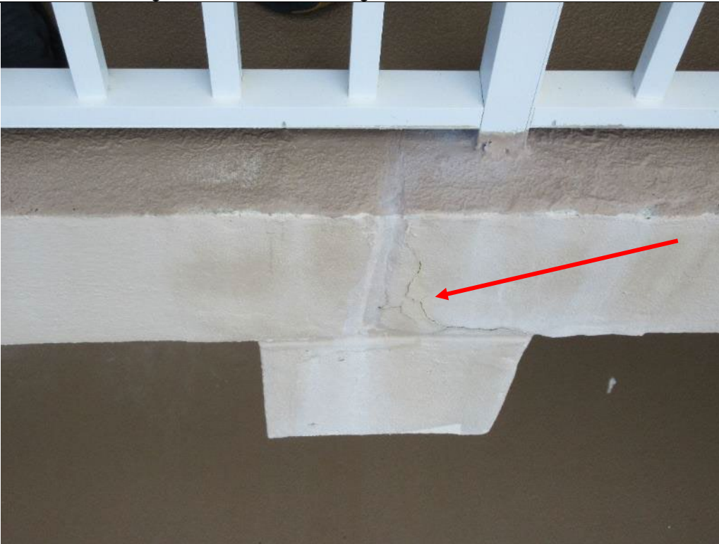
Photo 28. Crack at Slab Edge with Efflorescence near B403
