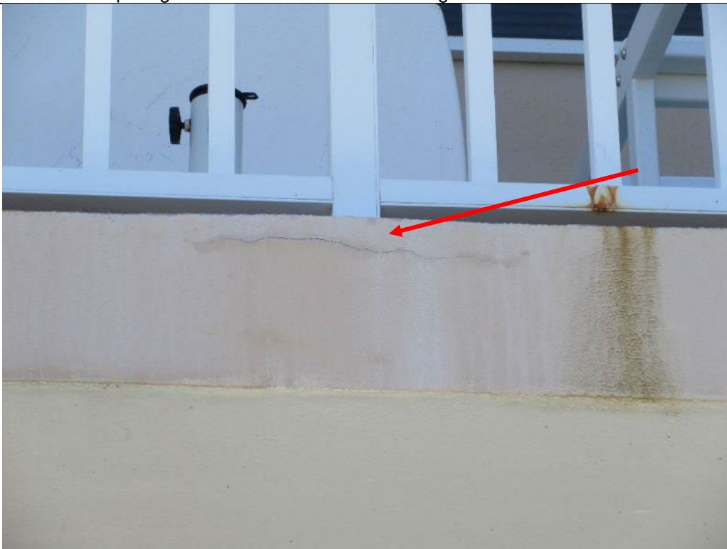
Photo 86. Crack and Spalling Concrete at Slab Edge E203 Corrosion at Railing
