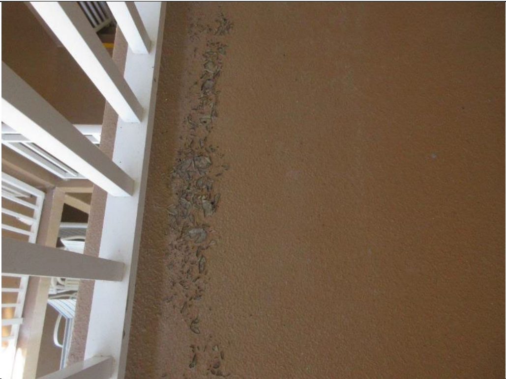
Photo 89. Typical Failed Waterproofing E401
