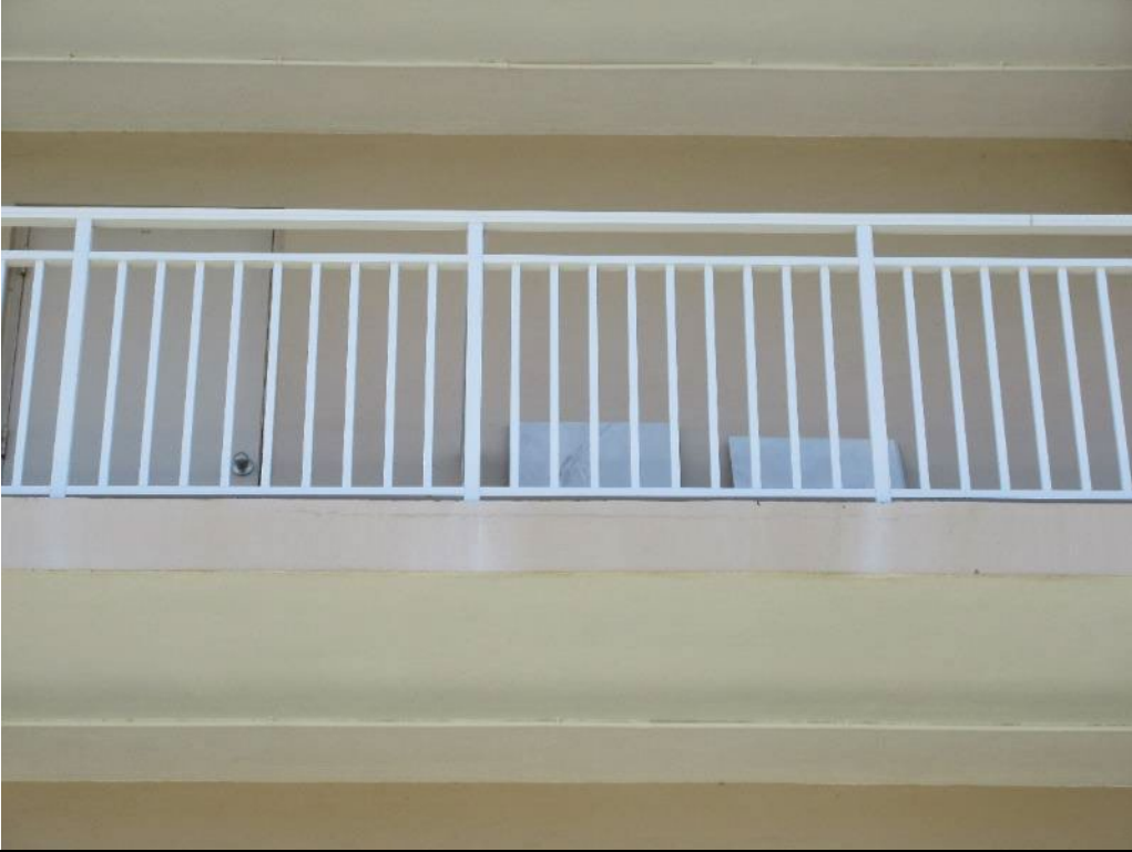
Photo 71. Crack and Spall at Slab Edge at 3 rd Floor Lobby
