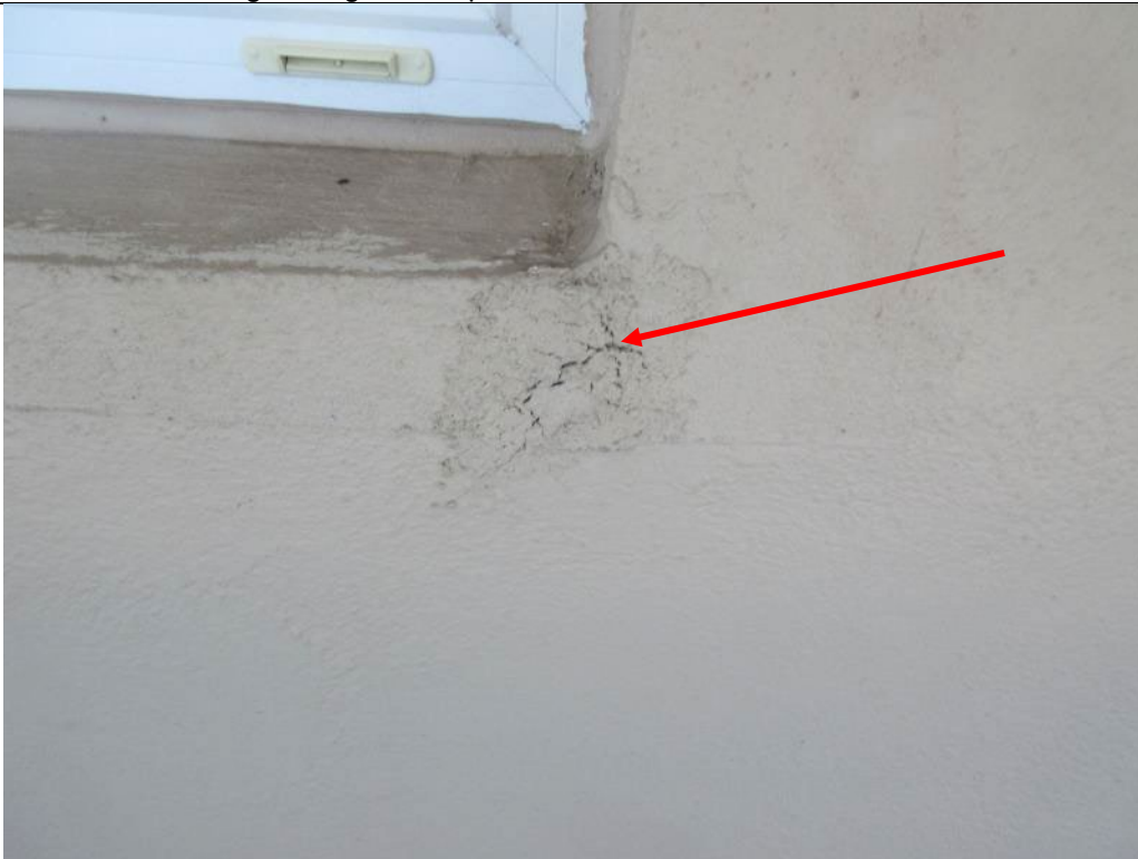
Photo 93. Damaged Windowsill at E303
