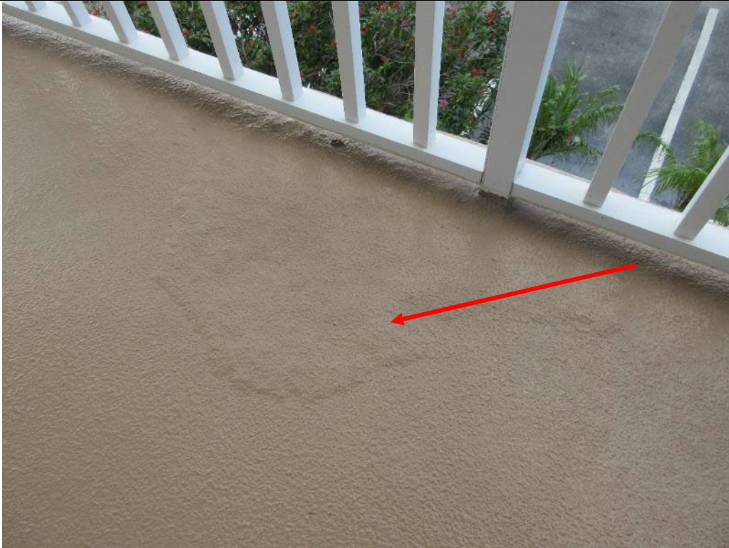
Photo 11. Apparent Spalling Concrete
