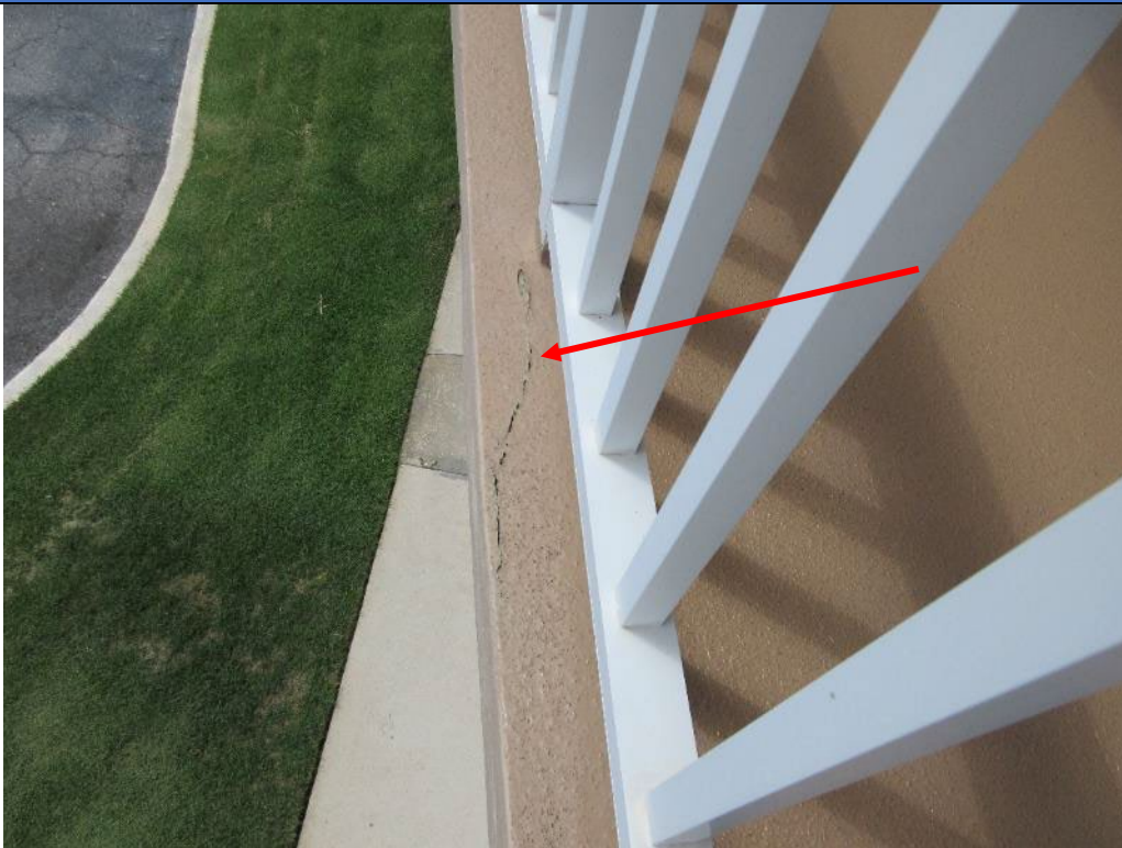
Photo 81. Spalling Concrete and Crack at Slab Edge Near Post Pocket E204
