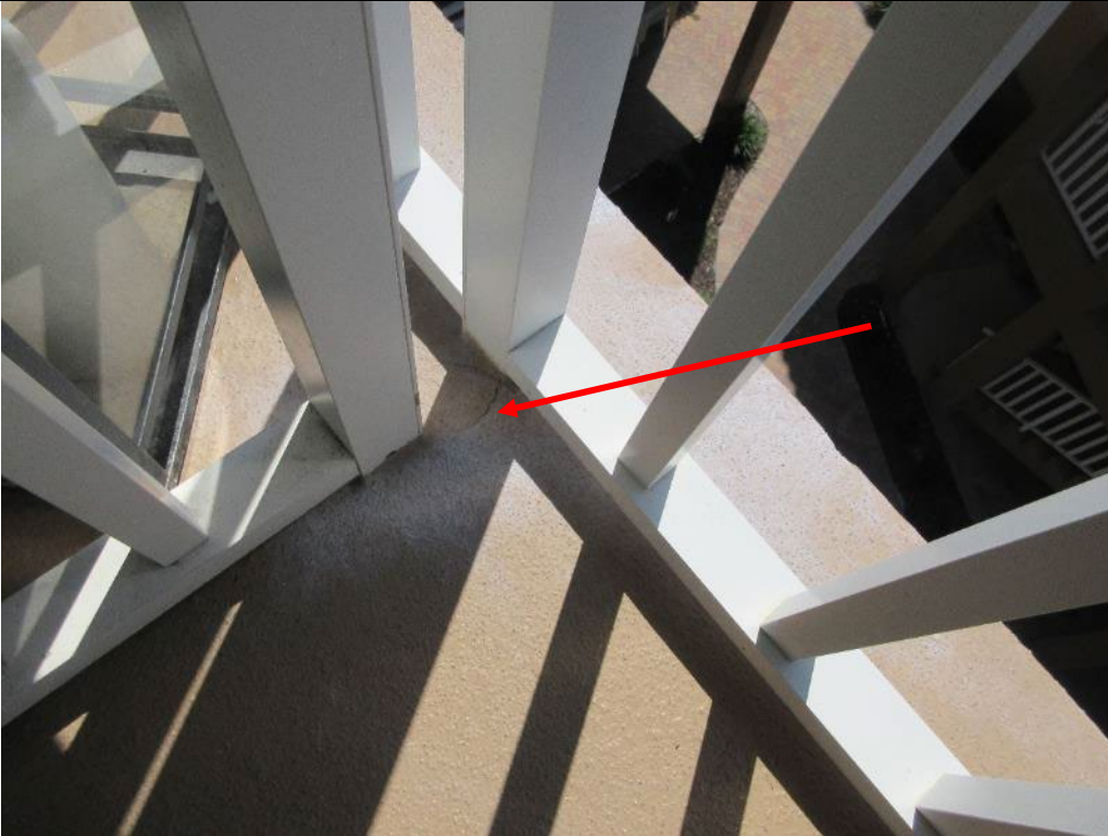
Photo 45. Failed Post Pocket and Waterproofing with Efflorescence C402
