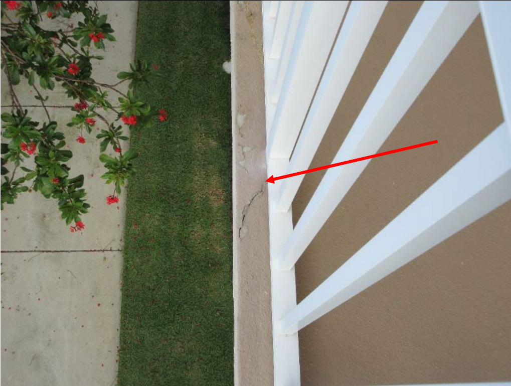
Photo 9. Cracked and Spalling Concrete at Railing Post Pocket and Failed Deck Coating
