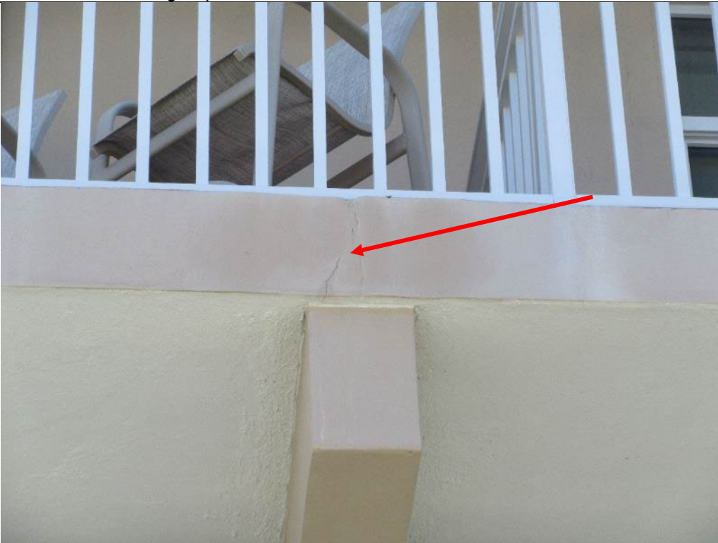
Photo 68. D301 Balcony Slab Edge with Crack at Beam
