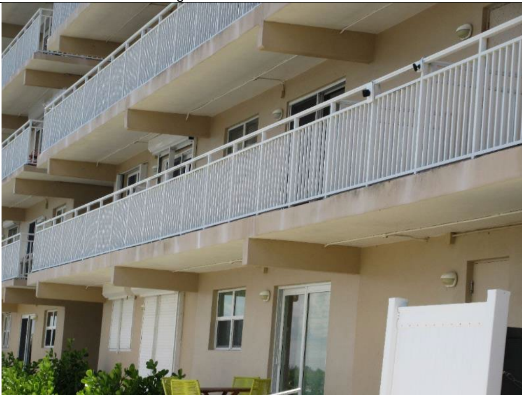
Photo 26. Typical Slab Edge Efflorescence at Unit Balconies Building B
