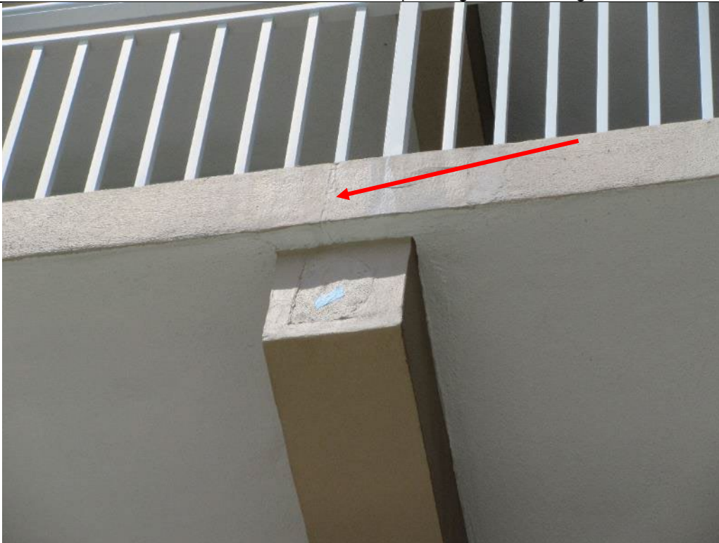
Photo 60. Crack at Slab Edge and Apparent Failed Previous Repair Near D10
