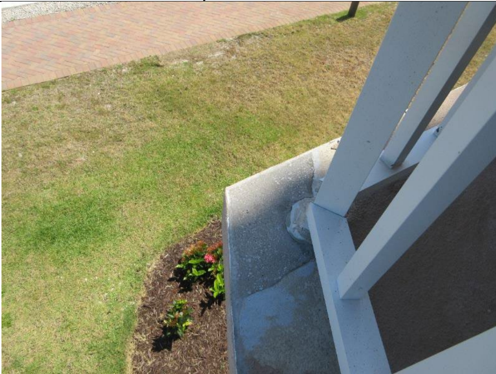
Photo 40. Previous Slab Edge Repair without Waterproofing C201
