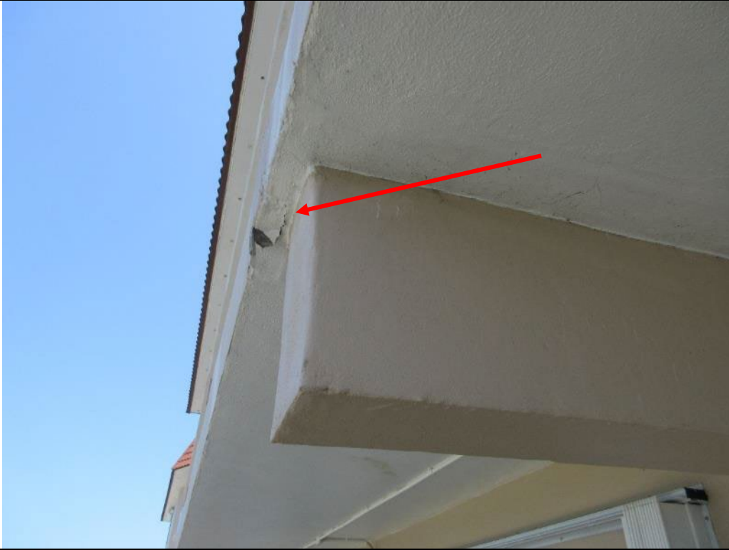
Photo 65. D202 Concrete Spall at Slab Edge at Cantilever Beam
