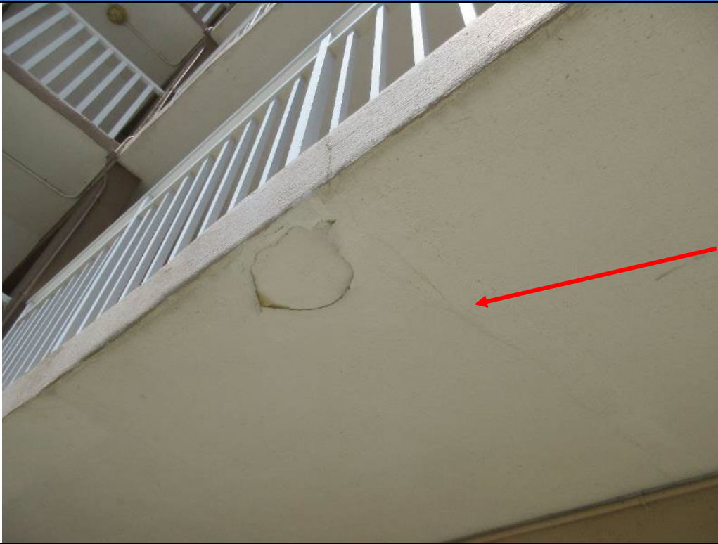
Photo 17. Unit A101 Ceiling with Crack and Delaminated Stucco
