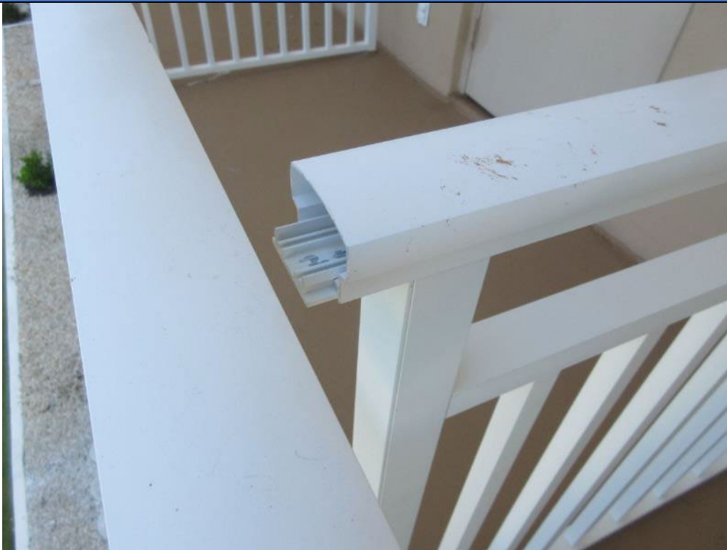
Photo 92. Missing Railing End Cap E303
