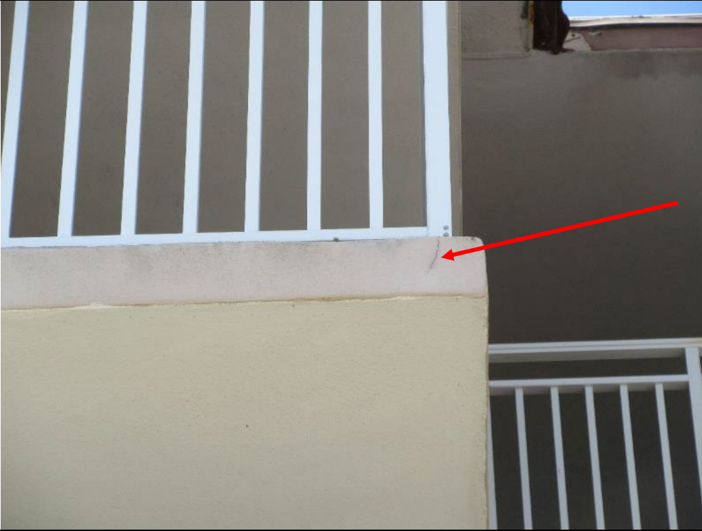
Photo 19. Slab Edge Crack and Spall A304
