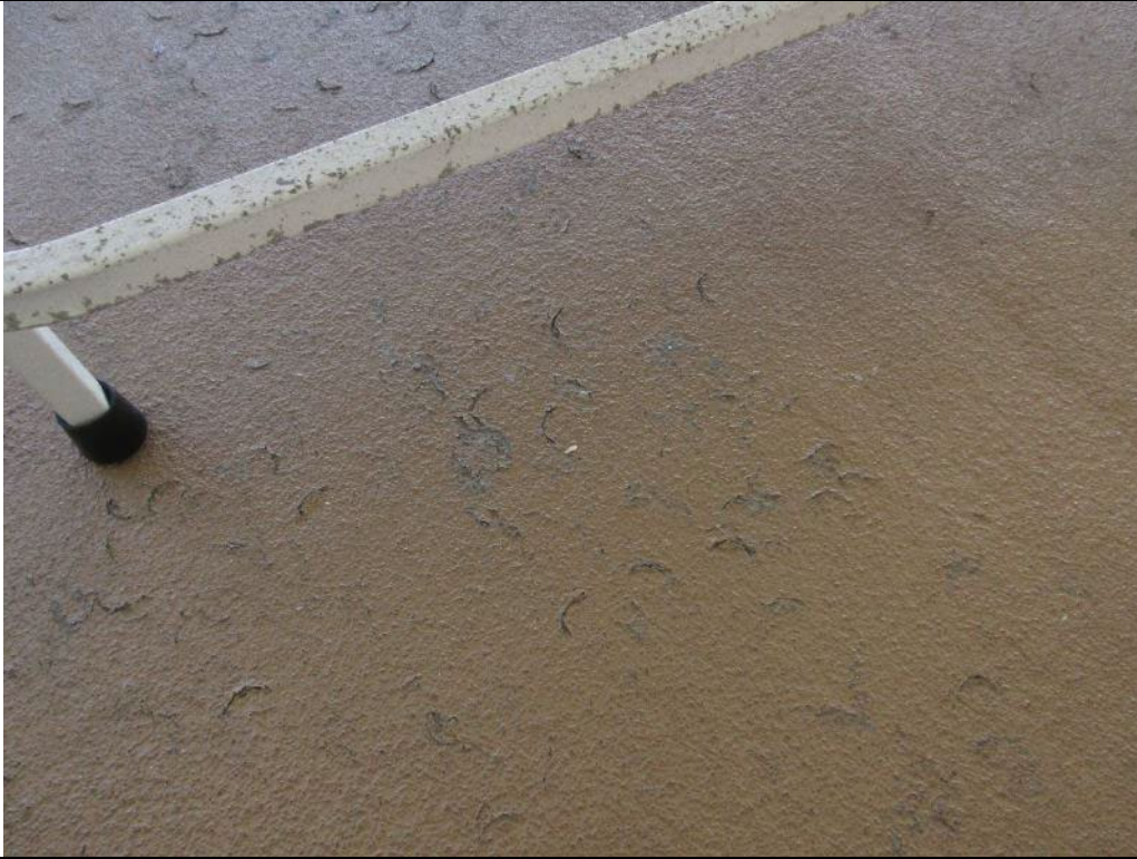
Photo 33. Typical Failed Deck Coating B403
