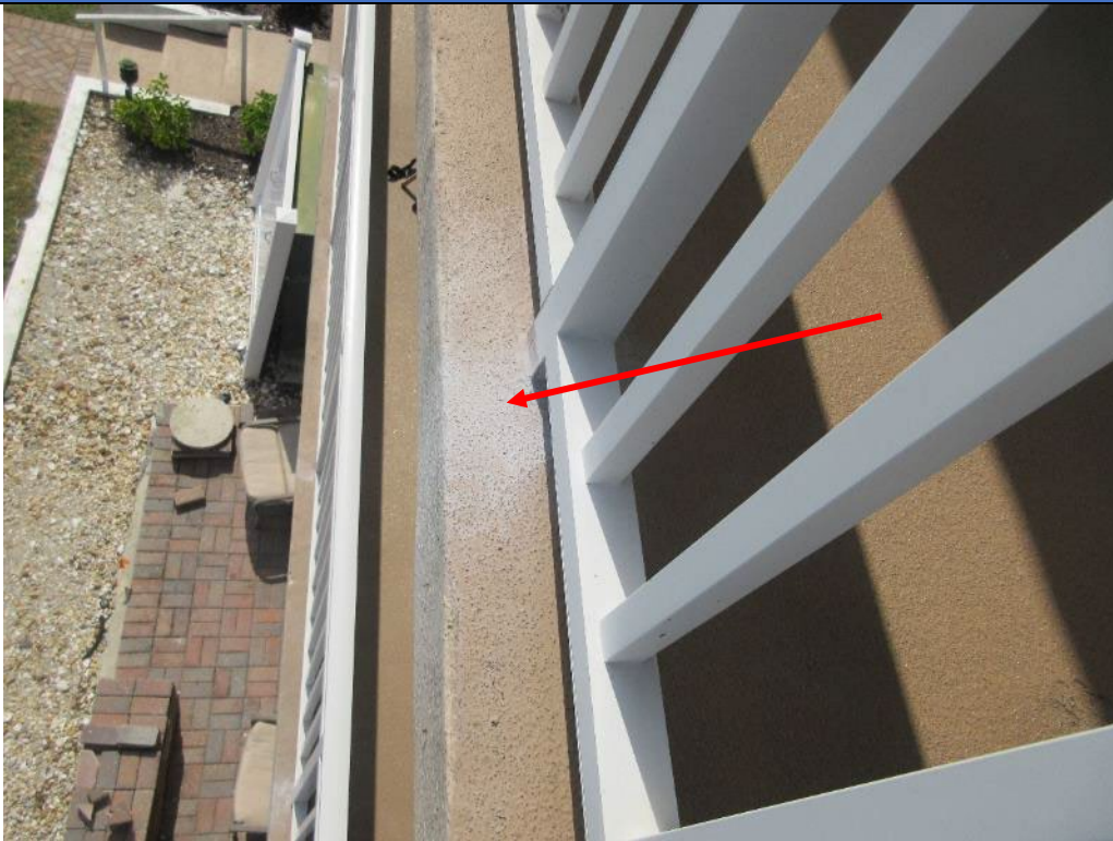
Photo 15. Typical Efflorescence at Railing Post
