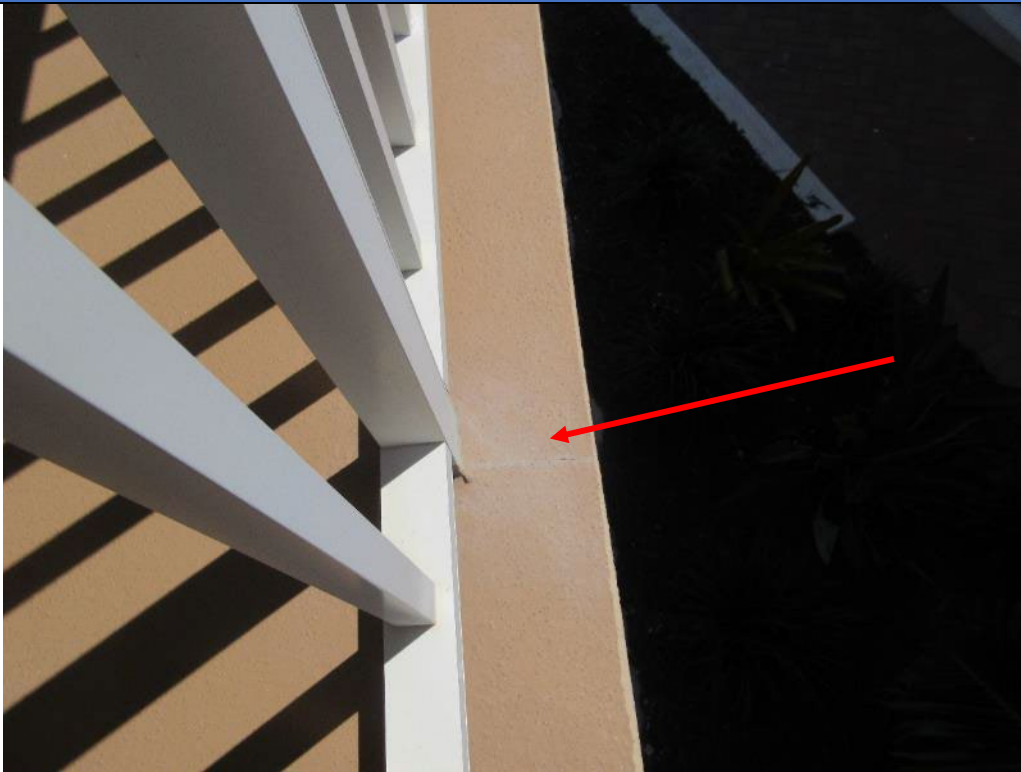
Photo 41. Crack at Slab Edge with Efflorescence C201 Balcony 2
