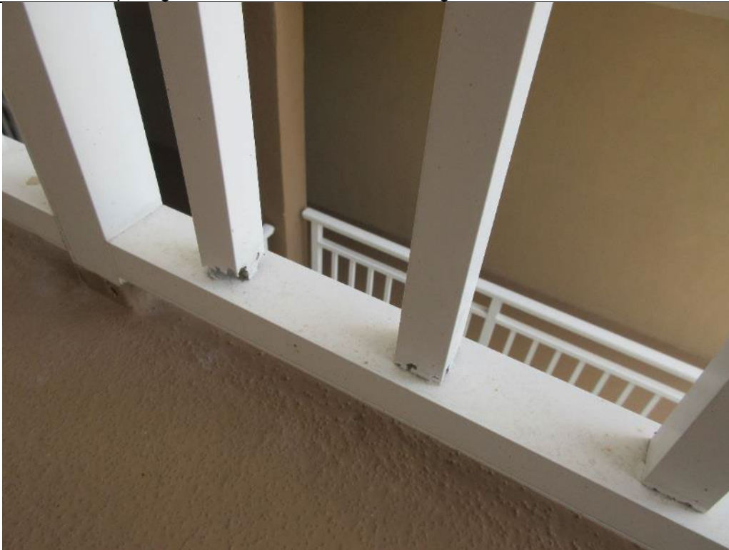
Photo 80. Typical Railing Picket Damage at Attachment Building E
