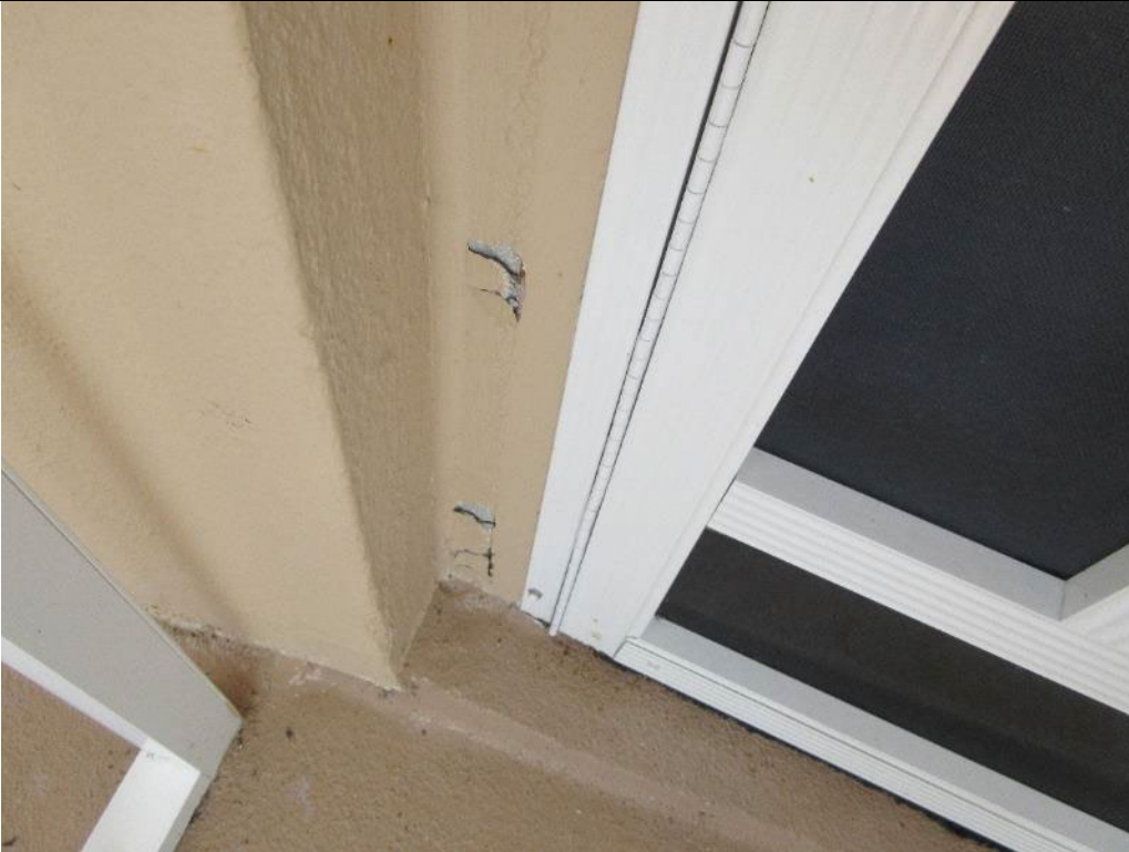
Photo 51. Damaged Stucco and Rusted Stucco Accessories Near C402
