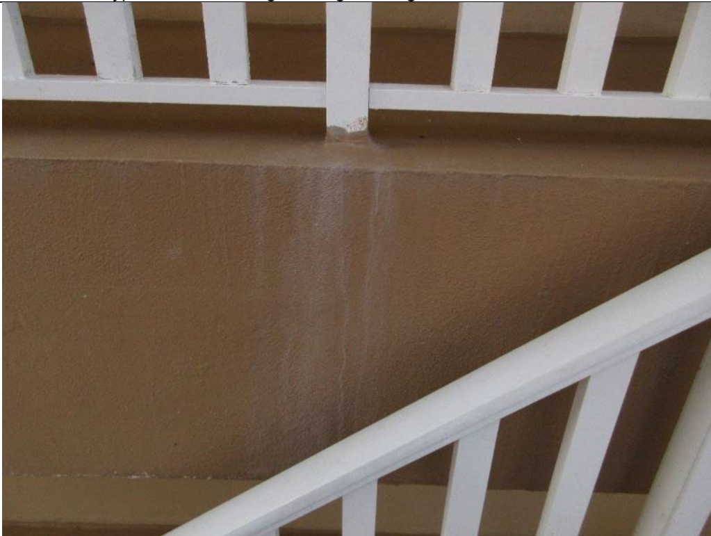
Photo 56. Typical Efflorescence at Slab Edge Railing Post
