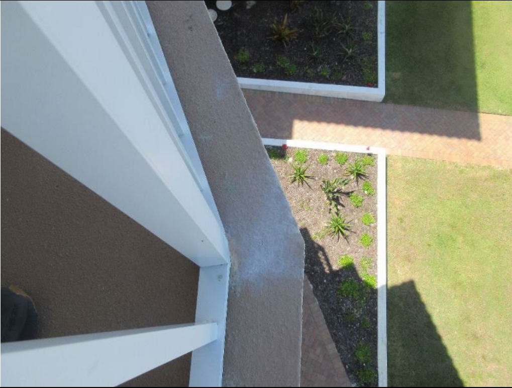
Photo 47. Crack and Apparent Spall at Slab Edge with Efflorescence
