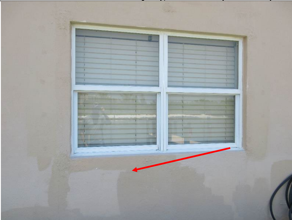
Photo 38. C103 Crack and Damaged Windowsill with Failed Previous Repair
