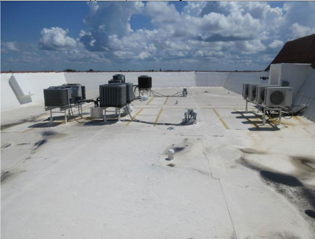
Photo 48. Overview Building C Roof Typical Ponding Areas
