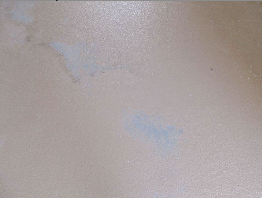
Photo 52. Typical Failed Deck Coating at Walkways
