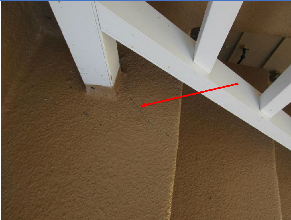
Photo 83. Concrete Spall and Crack at Stair Railing Post Building E East Stair
