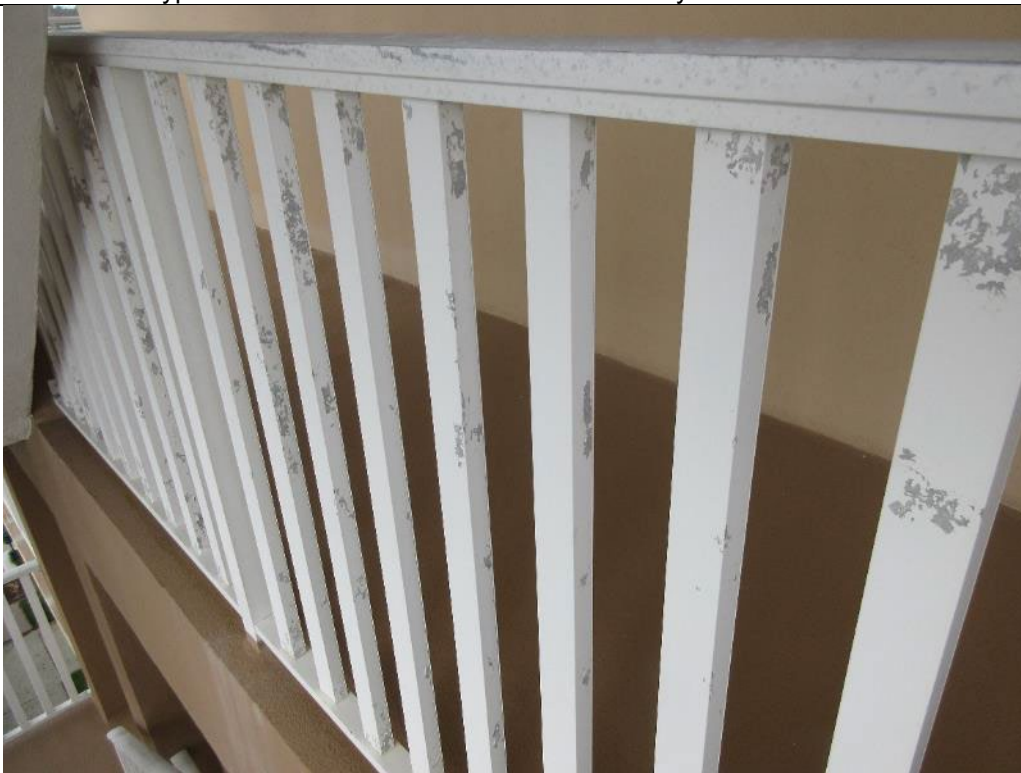
Photo 6. Typical Failed Guard Railing Coating
