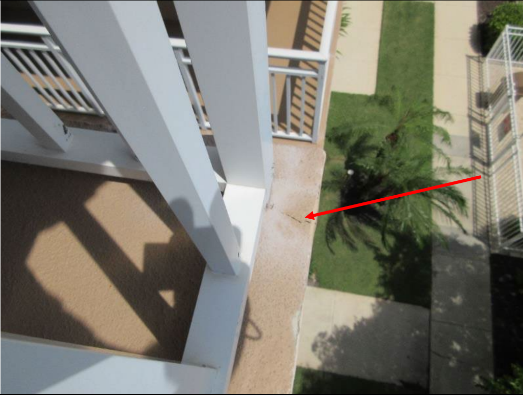
Photo 77. Slab Edge Crack and Spall Near E401
