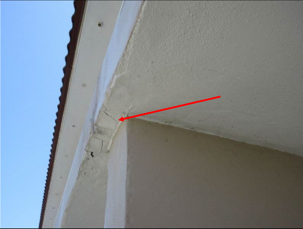
Photo 67. Slab Edge Spall at Cantilever Beam D302
