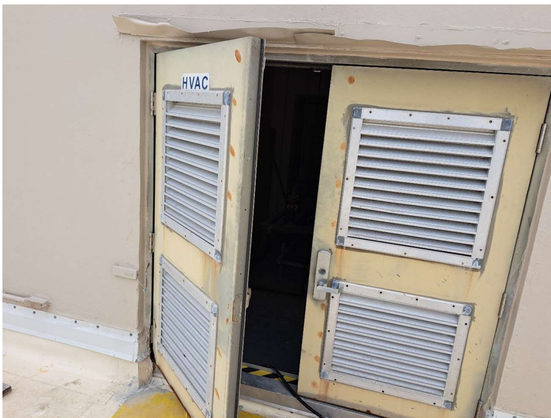
Photo 03 Ref: 2.1.2.1 – Missing / Damaged Exterior Doorway Overhead Flashing (Typical)
