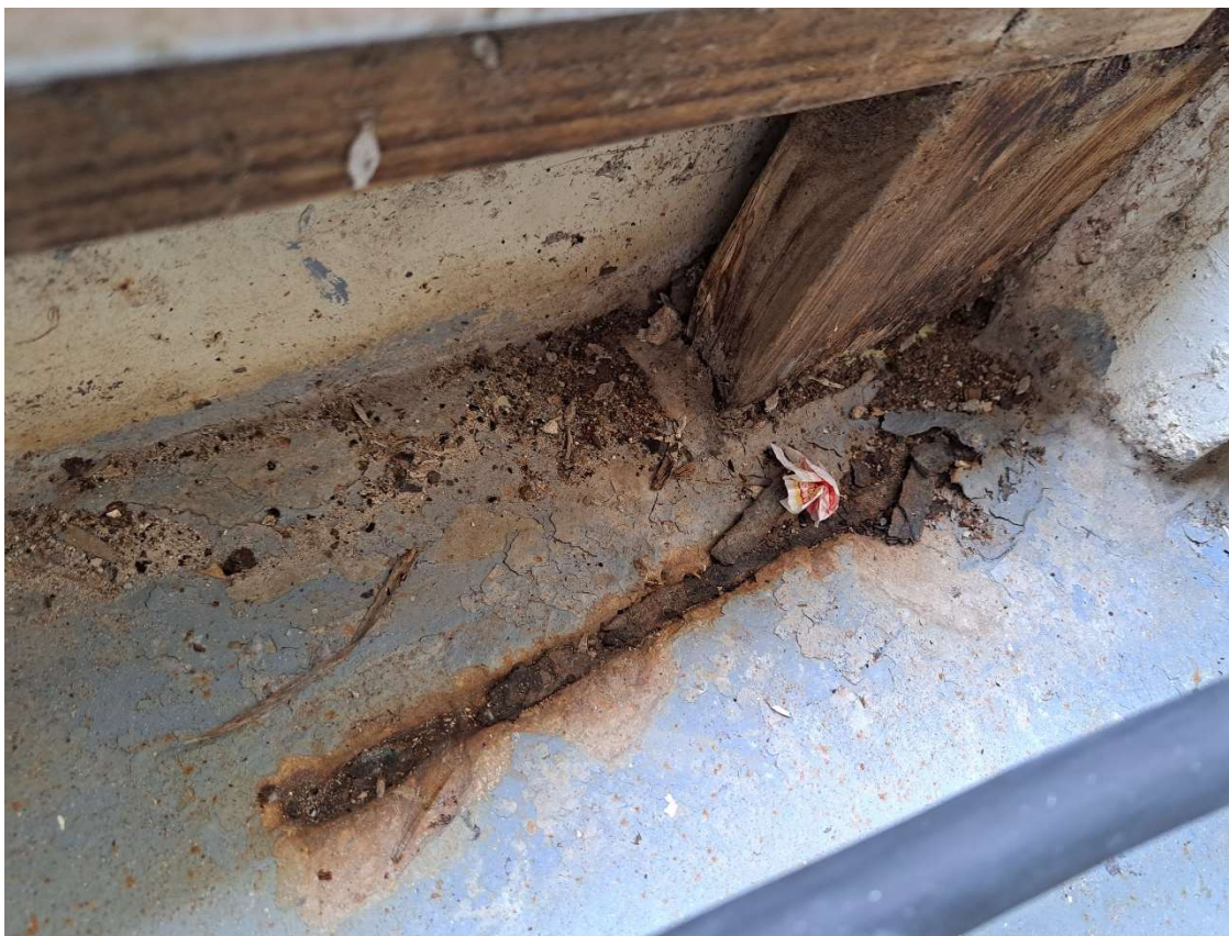
Photo 05 Ref: 2.1.2.1 – Missing / Damaged Exterior Doorway Overhead Flashing (Typical)
