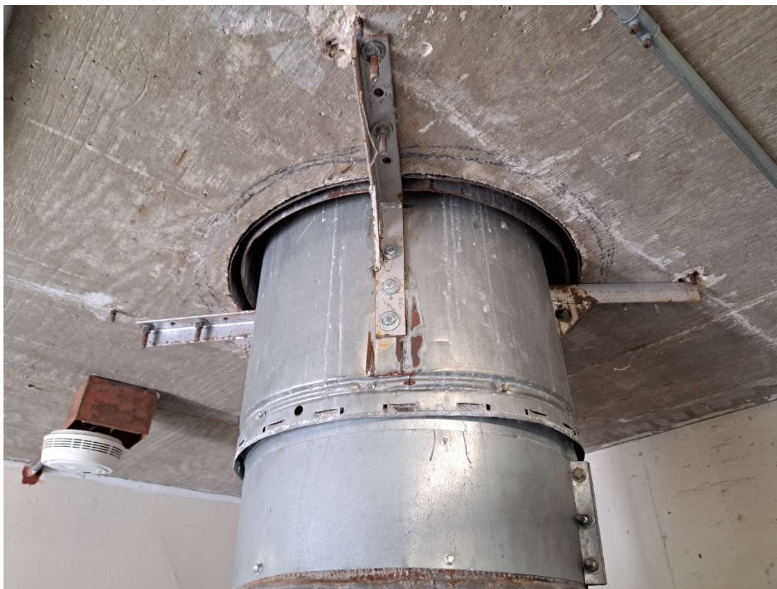
Photo 13 Ref: 2.1.8.1 – Boiler Room Leaking Vent Stack
