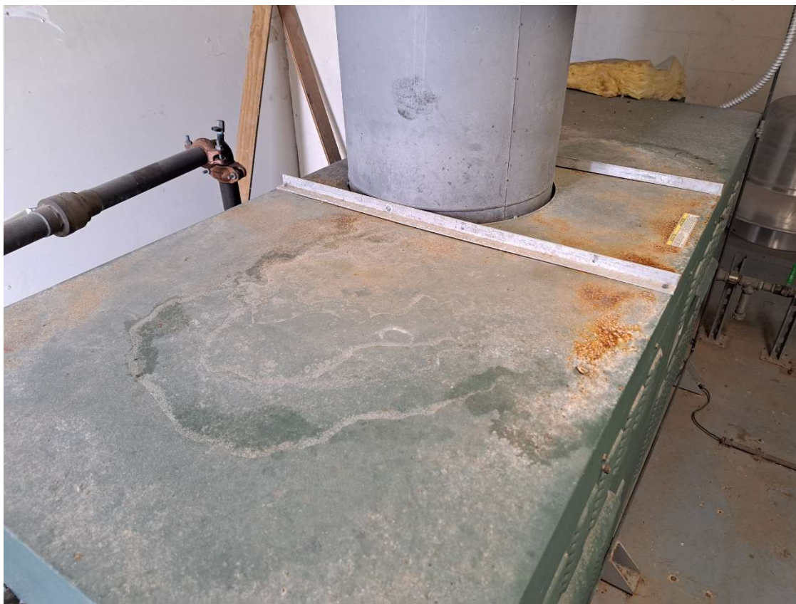
Photo 12 Ref: 2.1.8.1 – Boiler Room Leaking Vent Stack
