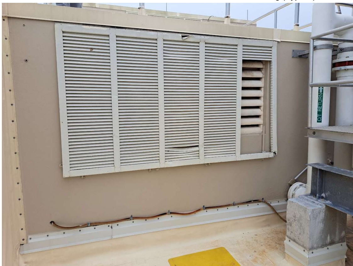
Photo 10 Ref: 2.1.7.1 – Rooftop HVAC Pumphouse Window Covering
