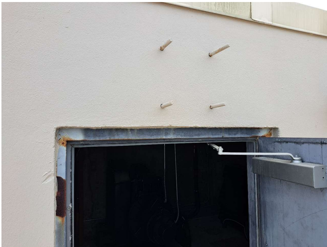
Photo 04 Ref: 2.1.2.1 – Missing / Damaged Exterior Doorway Overhead Flashing (Typical)
