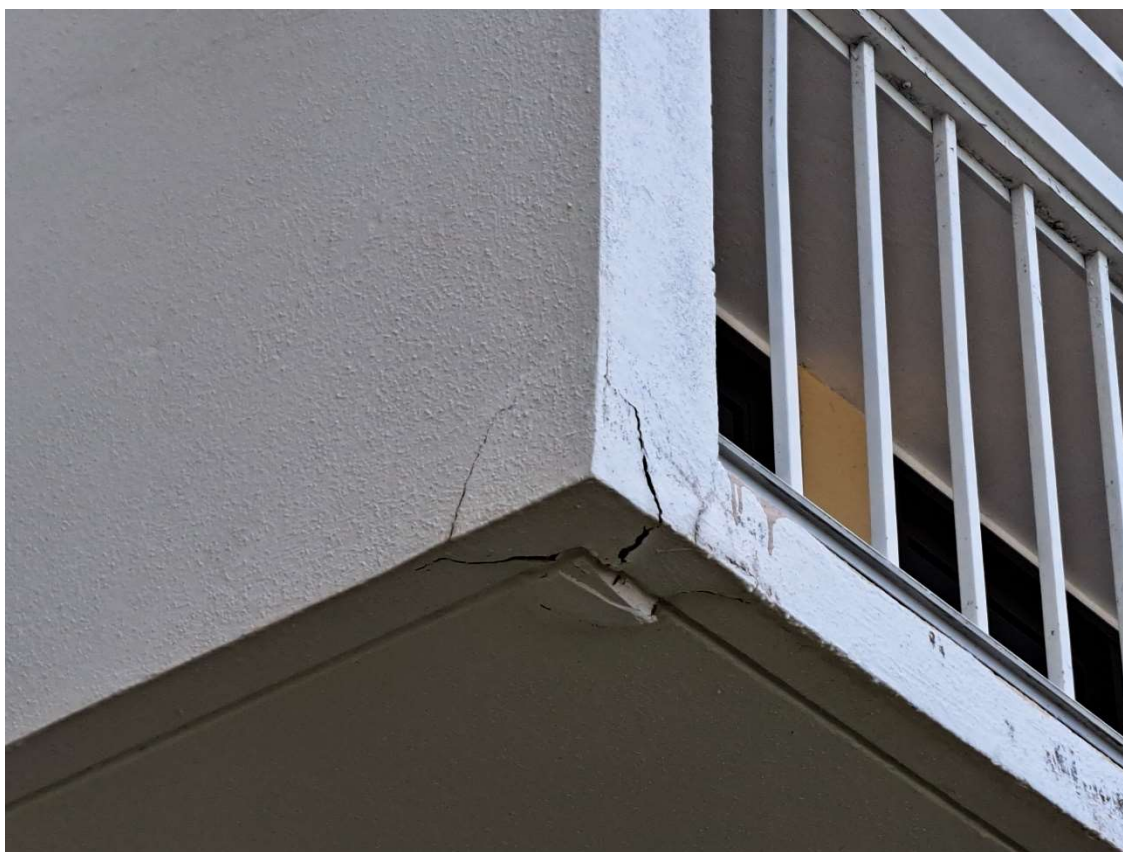
Photo 01 Ref:2.1.1.1 – Slab Corner Cracks/Spalling (Typical)
