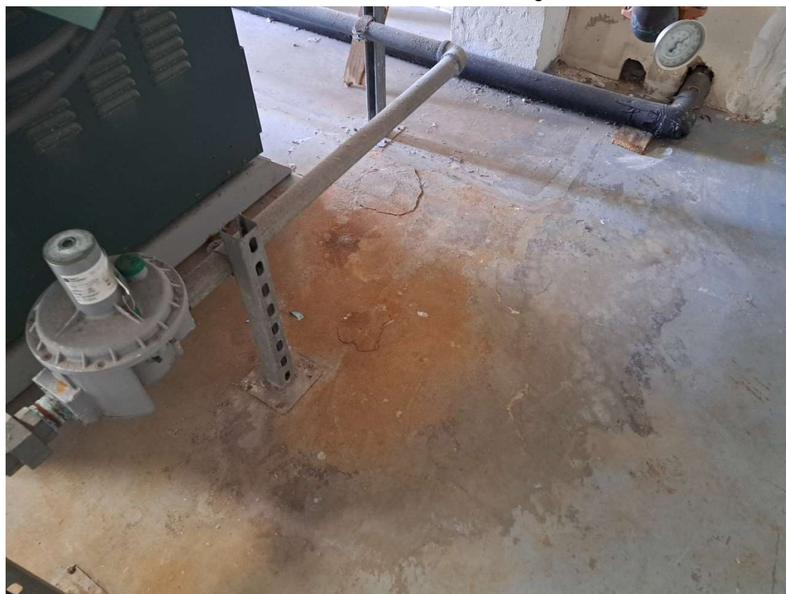
Photo 14 Ref: 2.1.8.1 – Boiler Room Leaking Vent Stack
