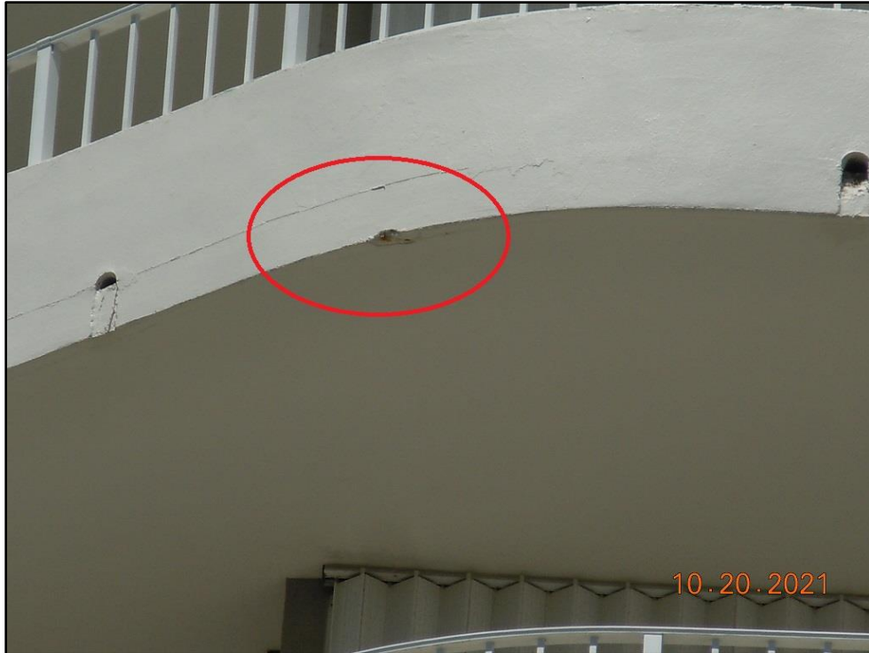
Concrete spalling 9 th floor South elevation
