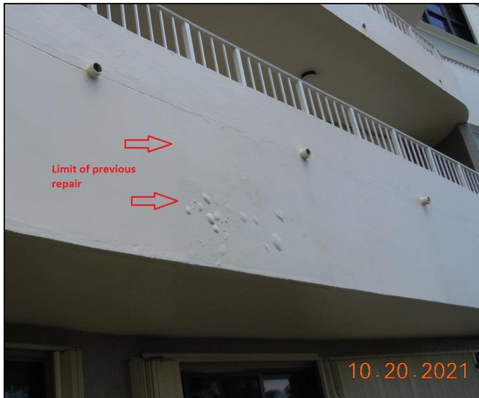
North Elevation, Coating failure near the previous concrete repair
