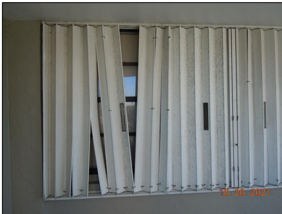
Unit 205, damaged shutters
