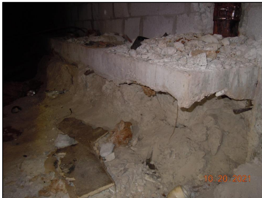
Undermined spread footing
