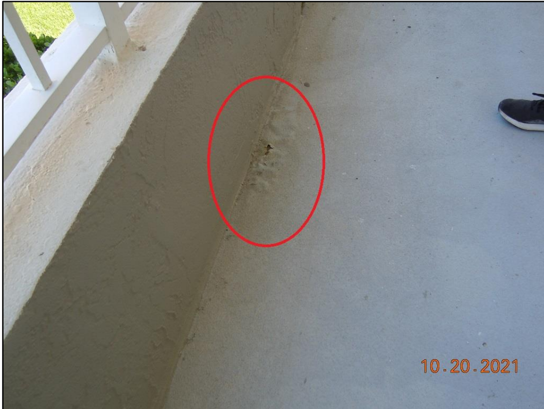
Unit 205 Failed water proofing
