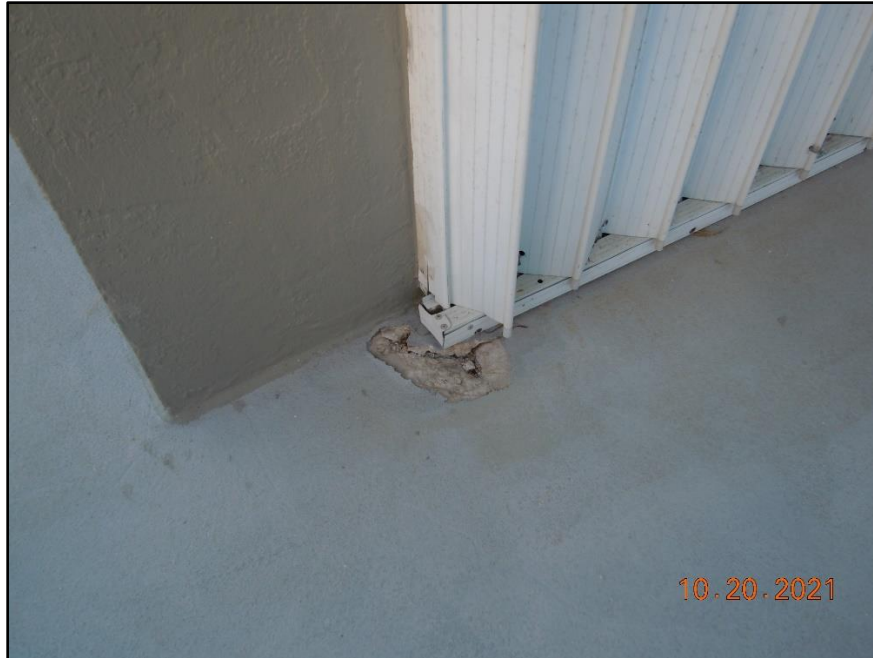
Unit 205 Concrete damage due to damaged shutters
