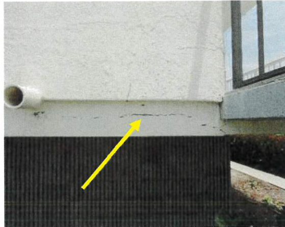
Photo 16: Cracked concrete pad.
