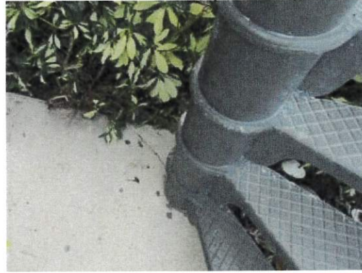
Photo 14: Cracked concrete pad at base of spiral stairs.
