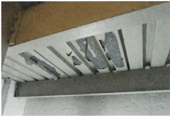
Photo 9: Corrosion of Steel Staircase
