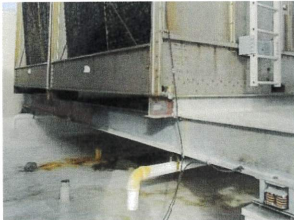
Photo 21: Server corrosion on multiple steel beam.
