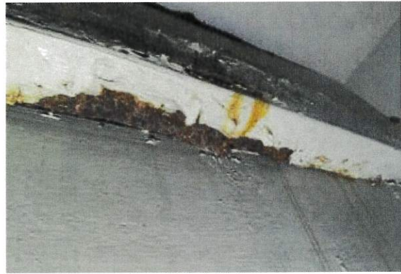
Photo 10: Corrosion of Steel Staircase
