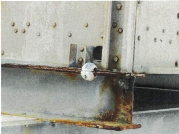
Photo 19: Server corrosion on steel beam.
