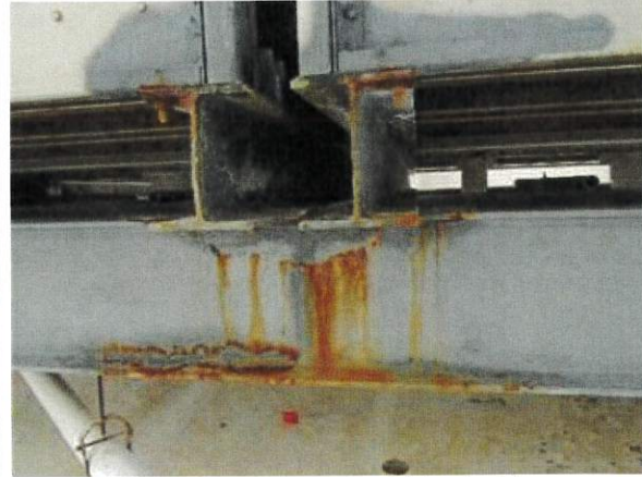
Photo 22: Server corrosion on multiple steel beam.
