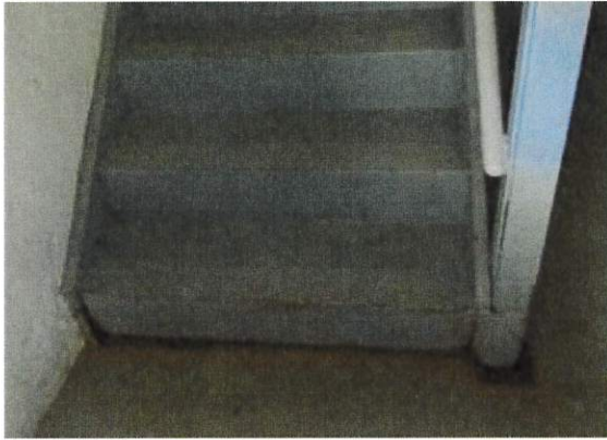
Photo 7: Corrosion of Steel Staircase
