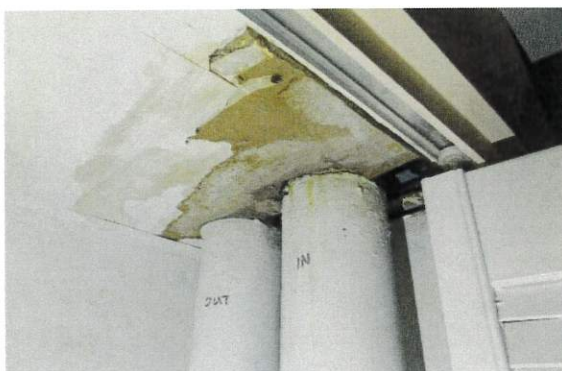
Photo 17: Spalled corrosion / corroded reinforcement to the slab in the HVAC Closet
