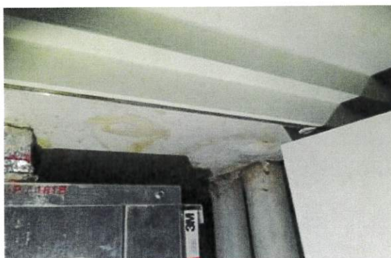
Photo 18: Spalled concrete to the slab in the HVAC Closet
