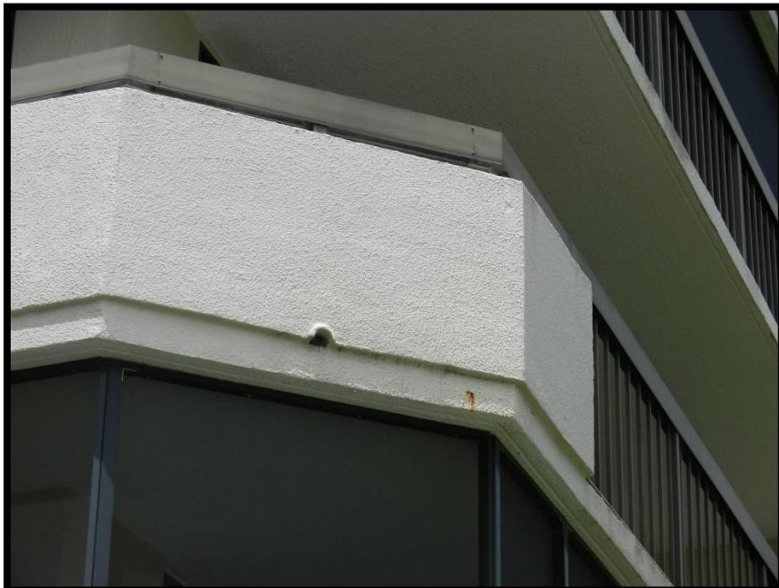
North Elevation Rust Streaking
