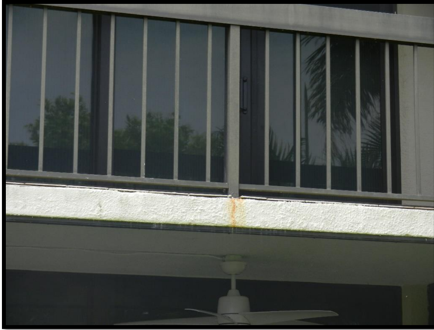
North Elevation Rust Streaking
