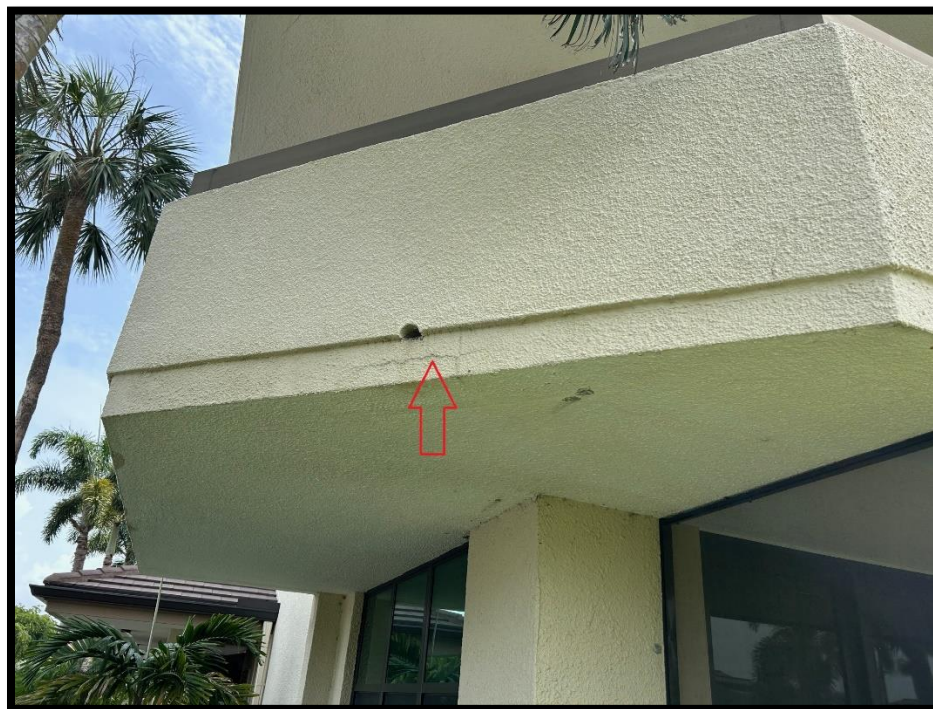
South Elevation Lanai Concrete Spauling
