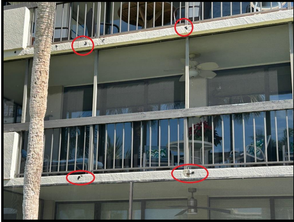
Areas Identified for Repair
