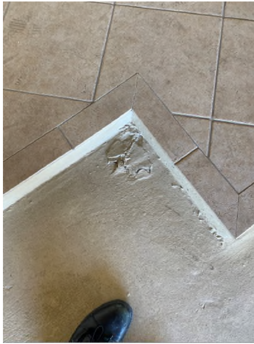
Figure 2: Concrete spall at slab. Common area.
