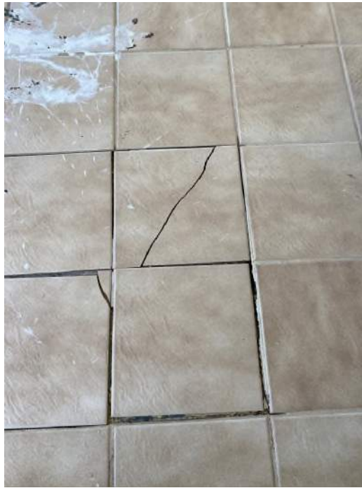
Figure 3: Cracked and delaminated tile at unit 622.
