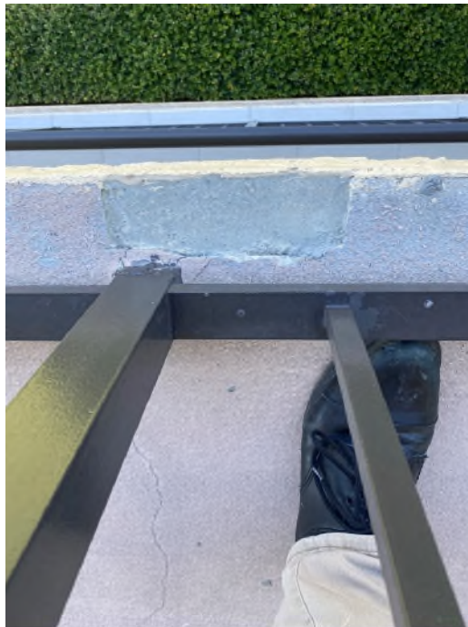
Figure 4: Stucco delamination and hairline crack. Unit 425.
