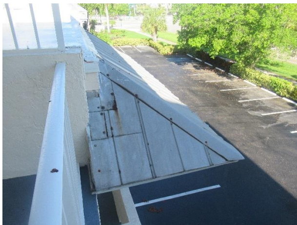
Rust at roof
