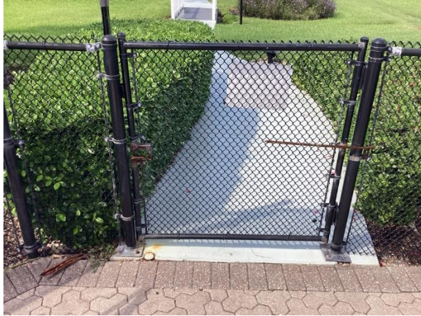
Fence post rust
