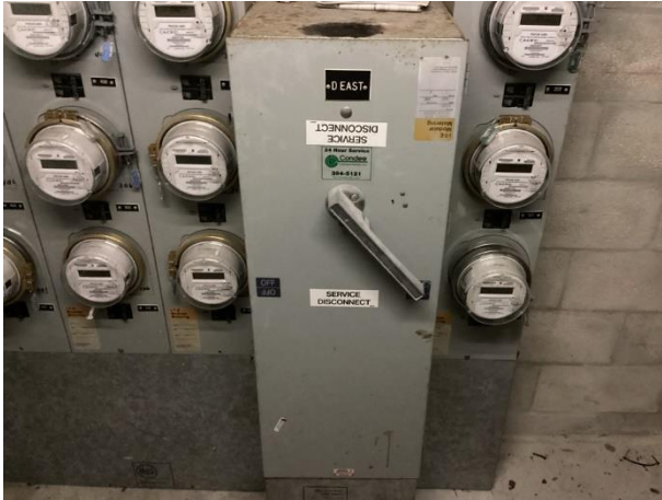
Main panel overview
