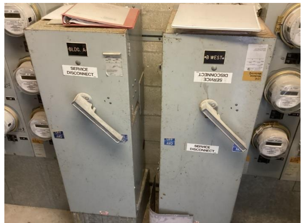
Main panel overview
