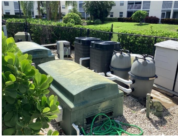
Pool mechanical equipment
