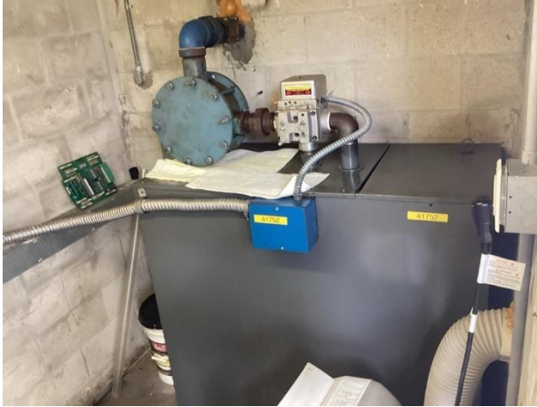
Hydraulic elevator equipment
