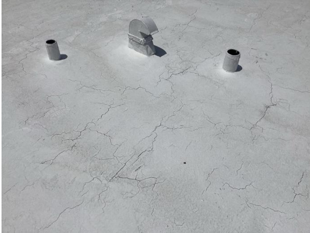
Cracks in membrane
