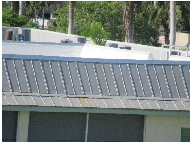
Rust at roof
