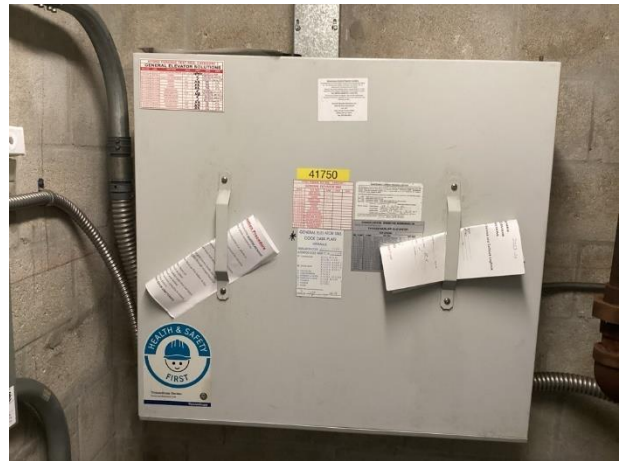
Hydraulic elevator controls
