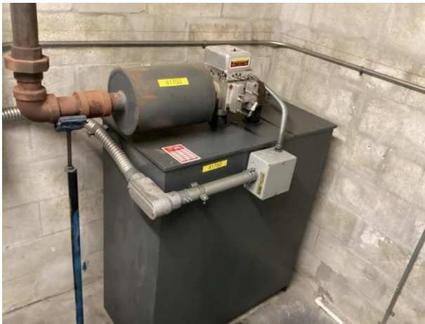
Hydraulic elevator equipment
