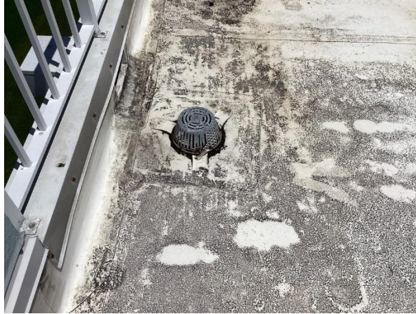
Deterioration at drain cap – Building C
