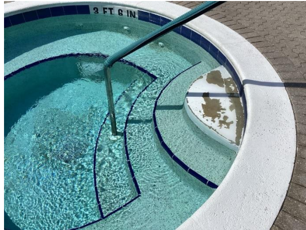
Plaster deterioration at spa
