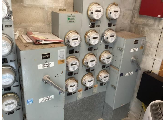
Main panel overview
