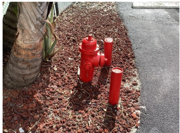
Fire hydrant overview
