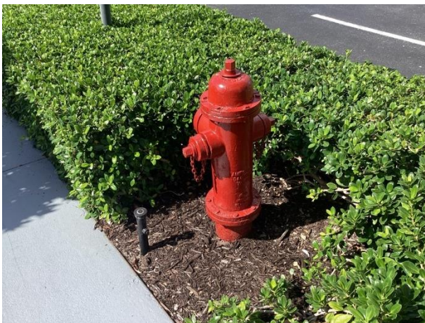
Fire hydrant overview
