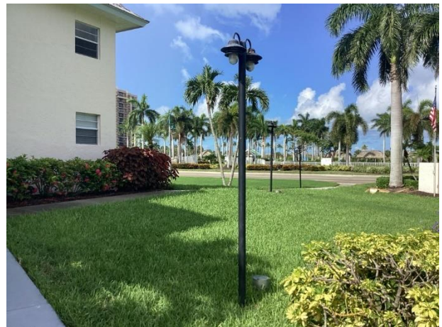
Light pole and fixtures
