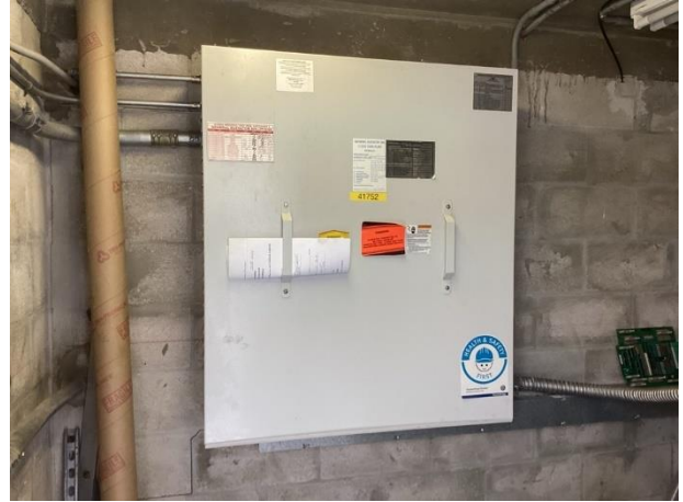
Hydraulic elevator controls
