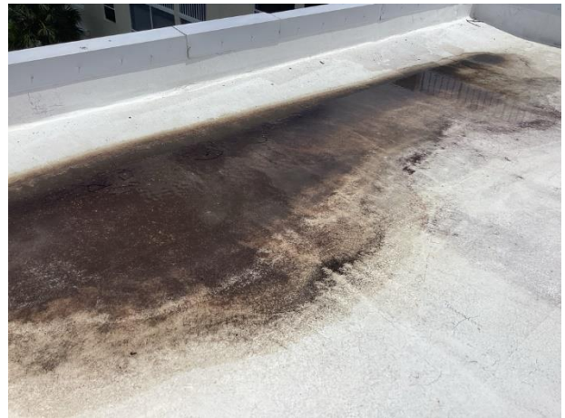
Evidence of standing water
