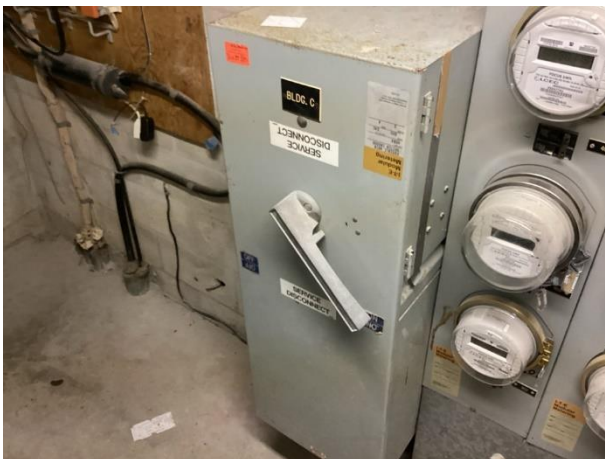
Main panel overview
