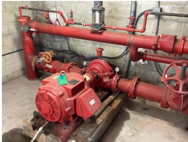
Fire suppression pump
