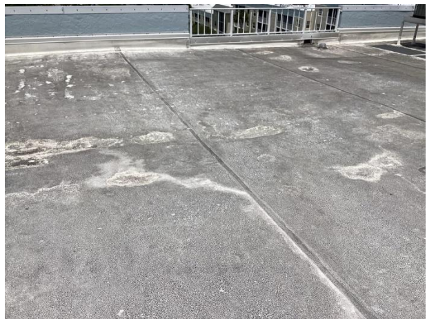
Roof deterioration – Building C
