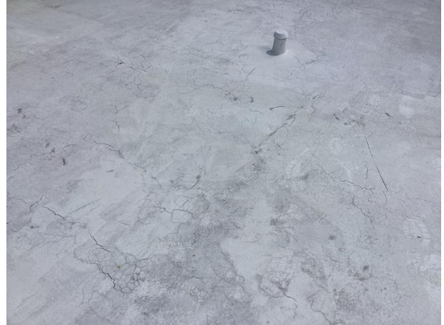
Cracks in membrane
