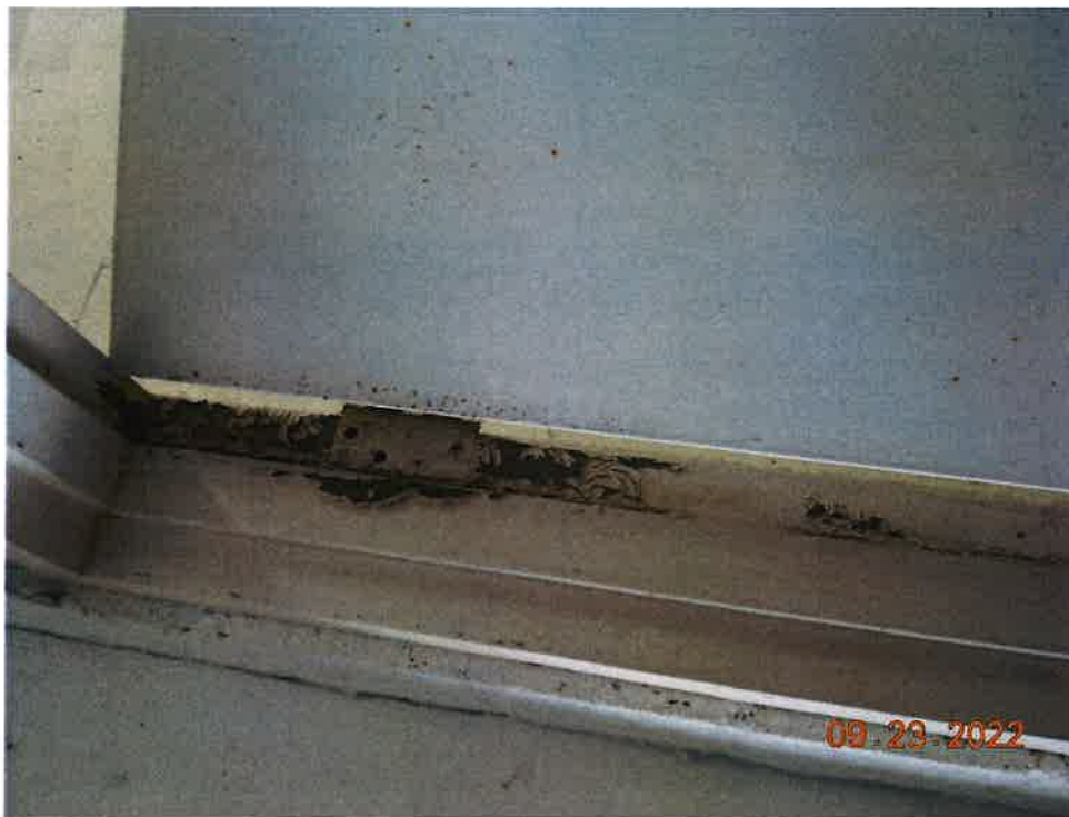
Furnace Roof Pass Door
