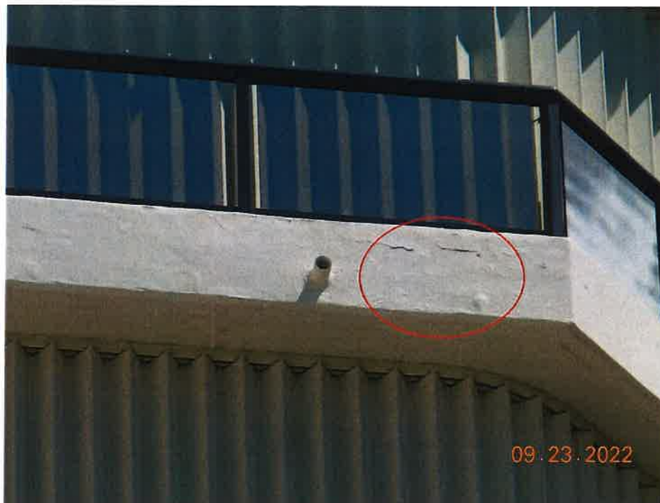
#4 Paint Blistering / Cracking
