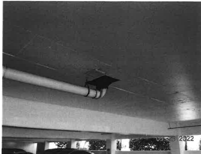
Rusted Rood Drains and Hangers
