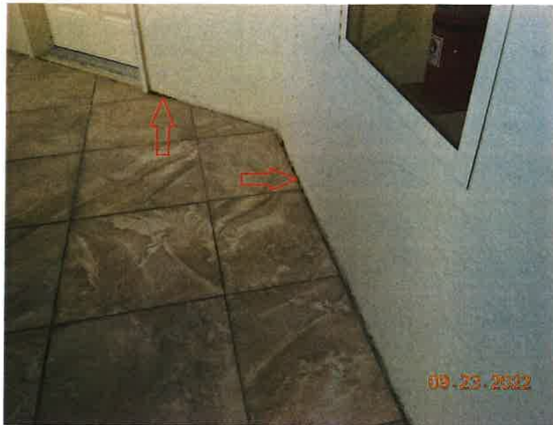
First Floor Moisture Damage
