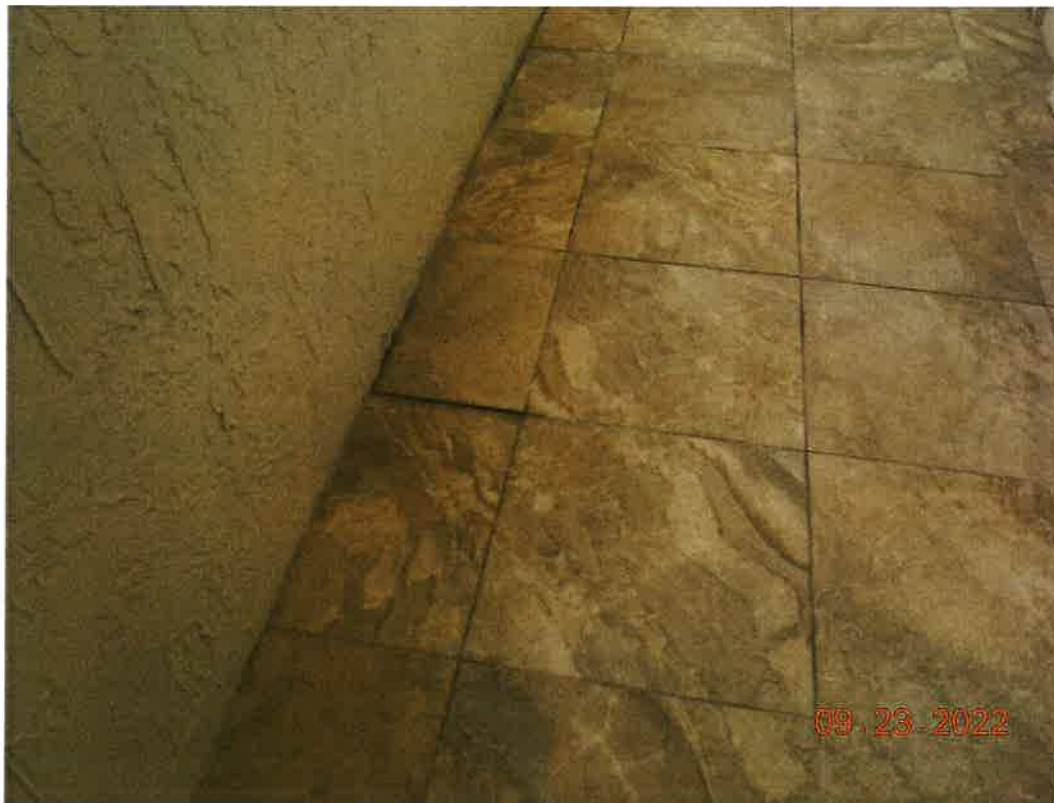
Delaminating Tile, 4 th Floor South
