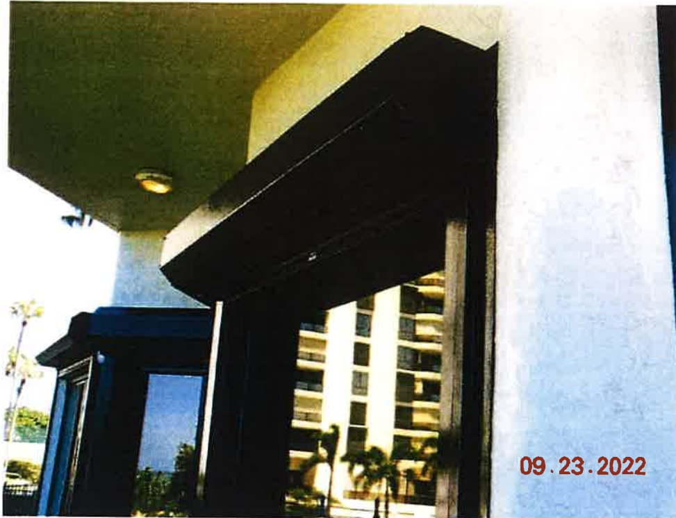
Storm Shutters at Ground Level
