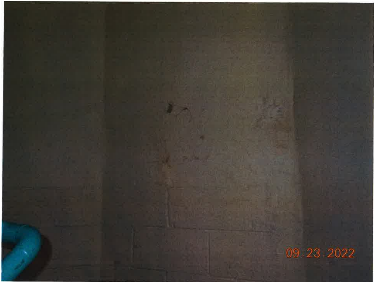
Moisture Infiltration Between Floors 12 and 13 both Stairwells
