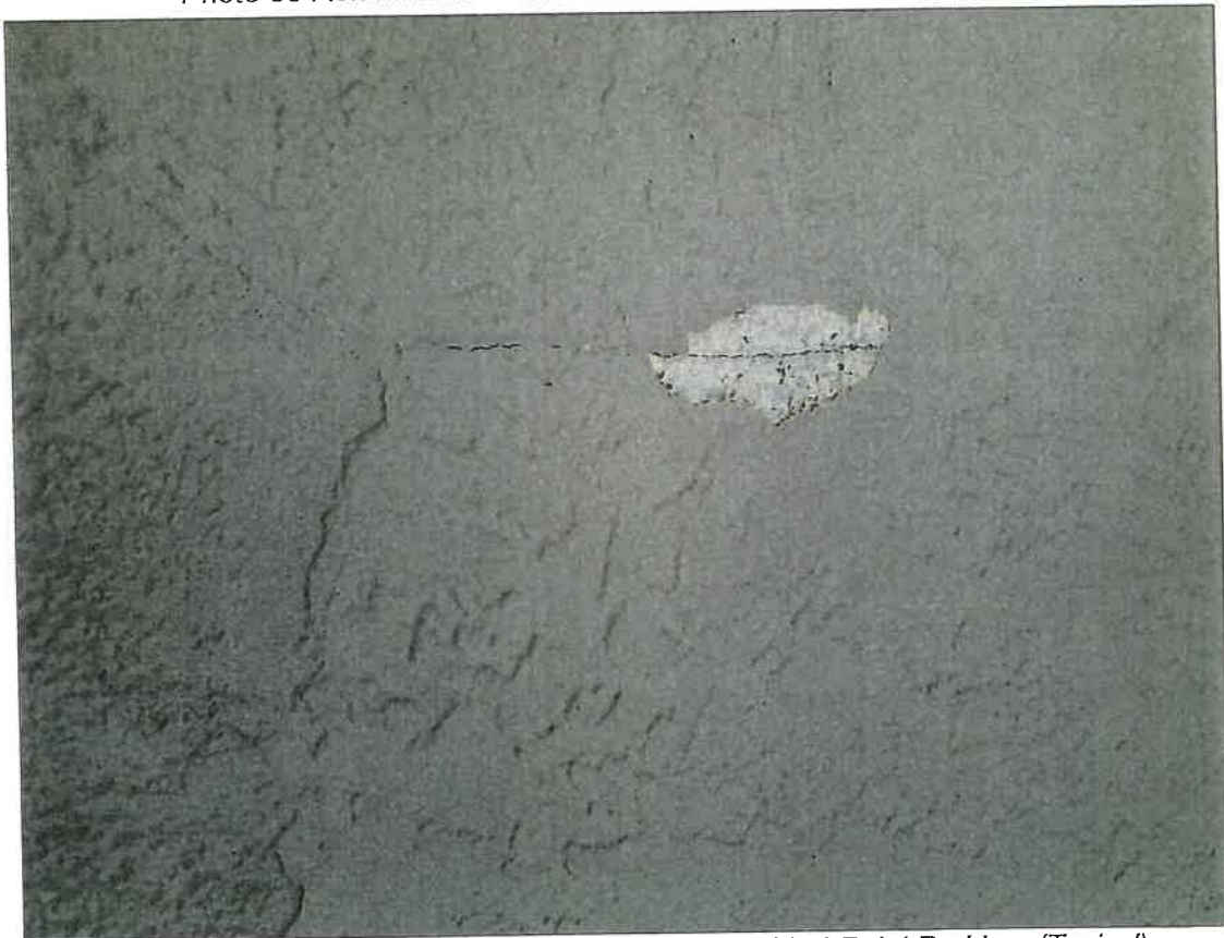
Photo 34 Ref: 2.2.7.2 – Stair Tower Moisture-Behind-Paint Problem (Typical)
