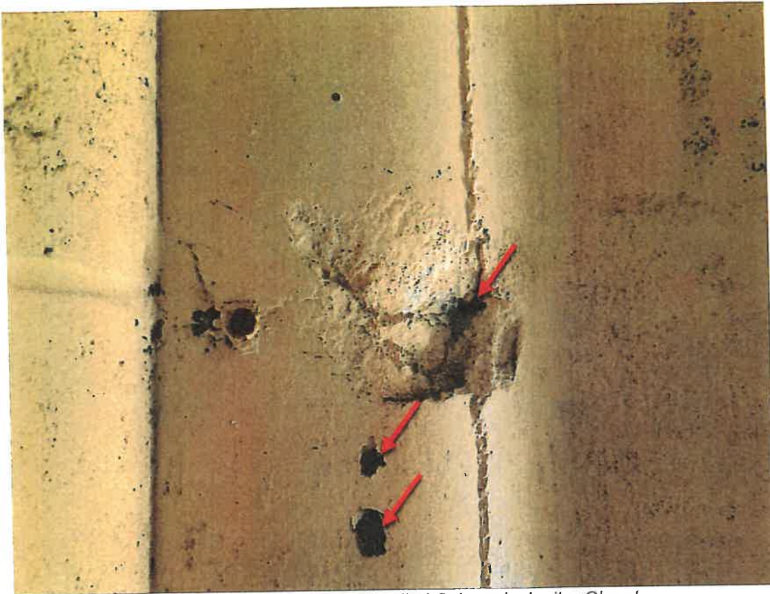
Photo 03 Ref: 2.1.1.1 – Spalled Column in Janitor Closet
