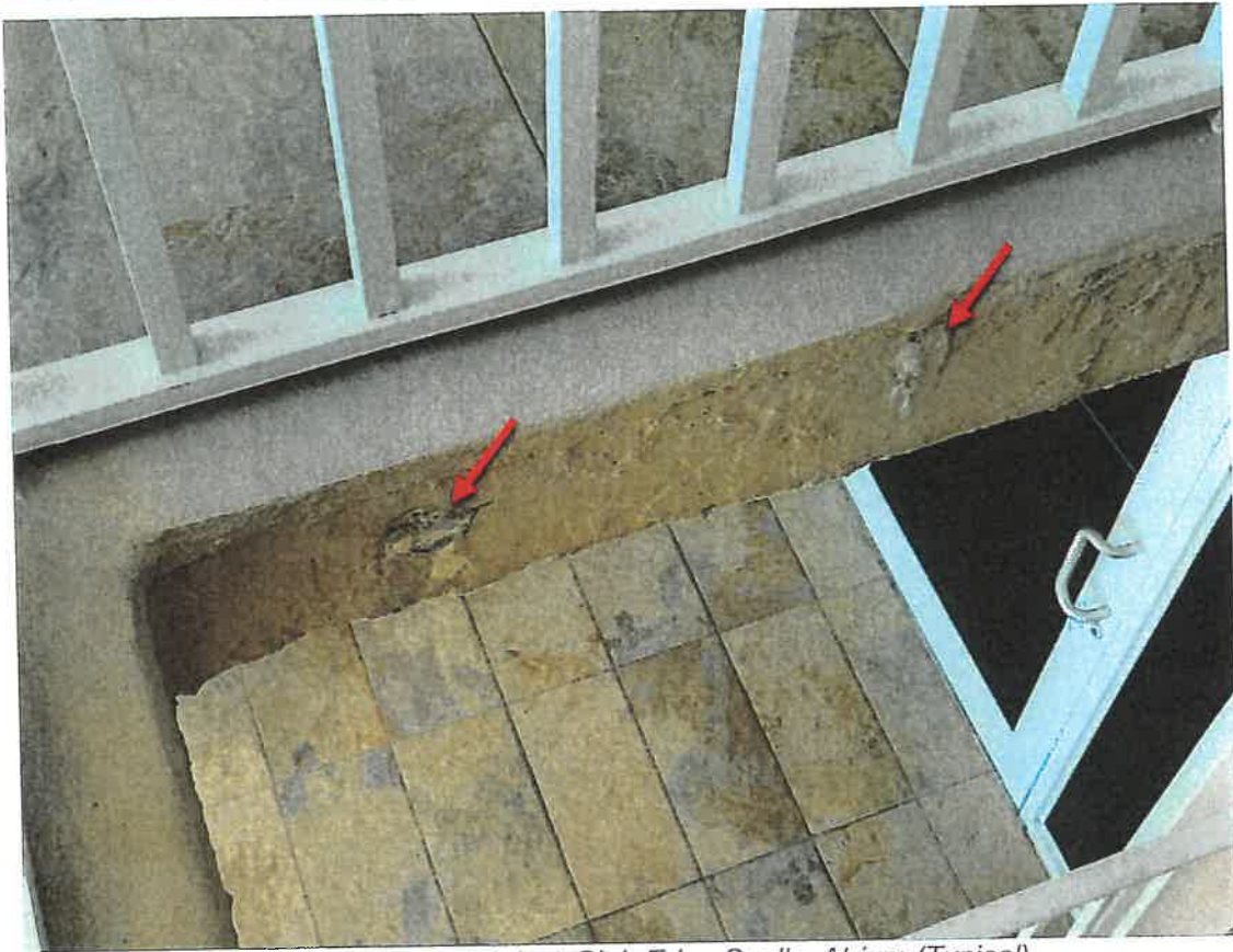
Photo 09 Ref: 2.1.4.1 – Slab Edge Spalls, Atrium (Typical)
