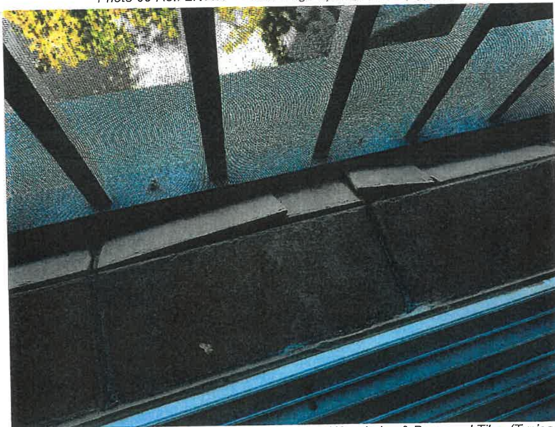
Photo 10 Ref: 2.2.1.1 – Blocked Screen Enclosure Weepholes & Damaged Tiles (Typical)
