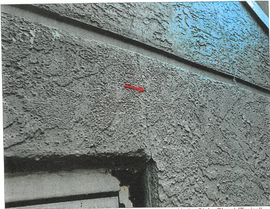
Photo 19 Ref: 2.2.5.1 – Cracks in Door Header Area, Under-Stairs Closet (Typical)
