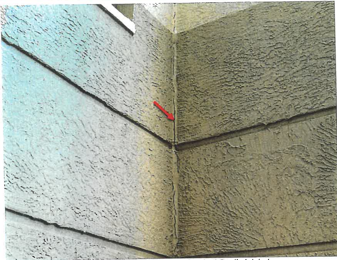
Photo 13 Ref: 2.2.3.1 – Cracked Caulk Joint at
