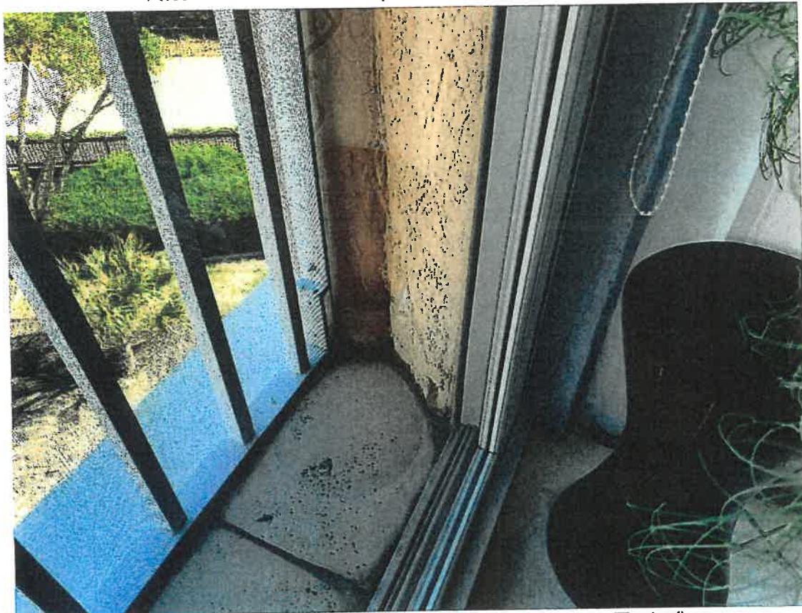
Photo 04 Ref: 2.1.2.1 – Spalled Lanai Column Base (Typical)
