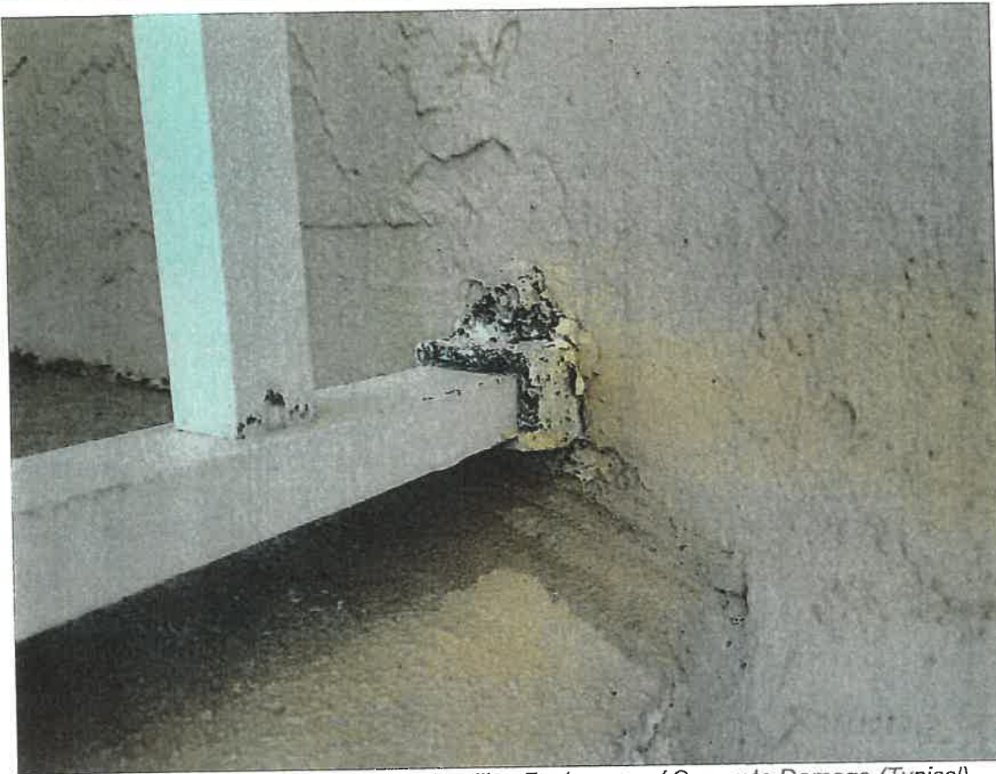
Photo 07 Ref: 2.1.3.1 – Corroded Railing Fasteners w/ Concrete Damage (Typical)
