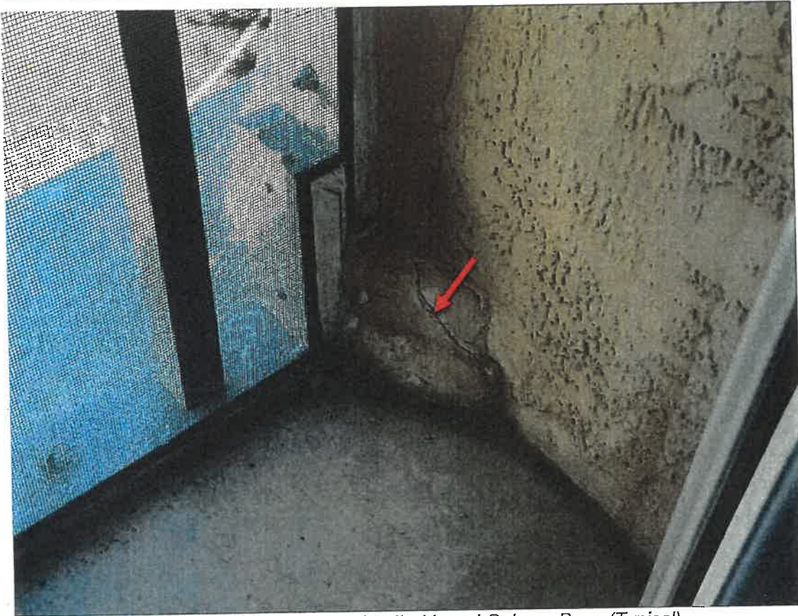
Photo 05 Ref: 2.1.2.1 – Spalled Lanai Column Base (Typical)
