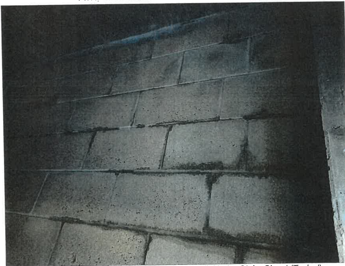
Photo 18 Ref: 2.2.5.1 – Moisture on Wall, Under-Stairs Closet (Typical)
