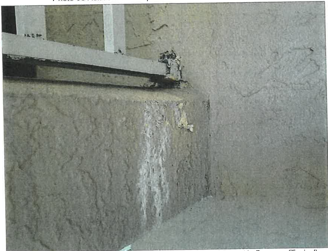
Photo 06 Ref: 2.1.3.1 – Corroded Railing Fasteners w/ Concrete Damage (Typical)
