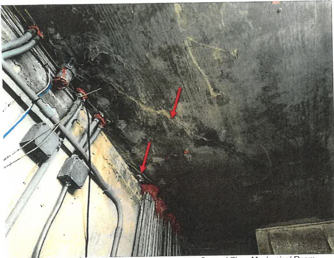
Photo 21 Ref: 2.2.5.1 – Crack Efflorescence, Ground Floor Mechanical Room
