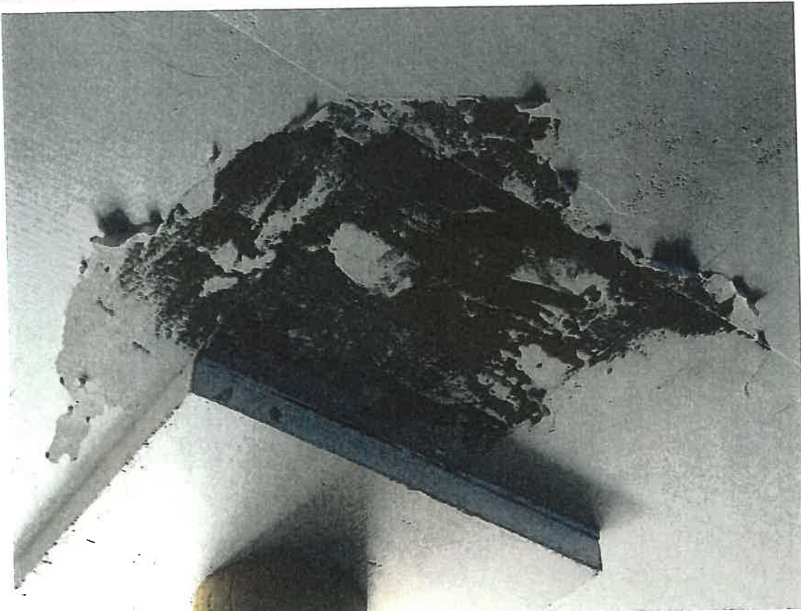
Photo 27 Ref: 2.2.6.1 – Moisture Coming Through Garage Ceiling (Typical)
