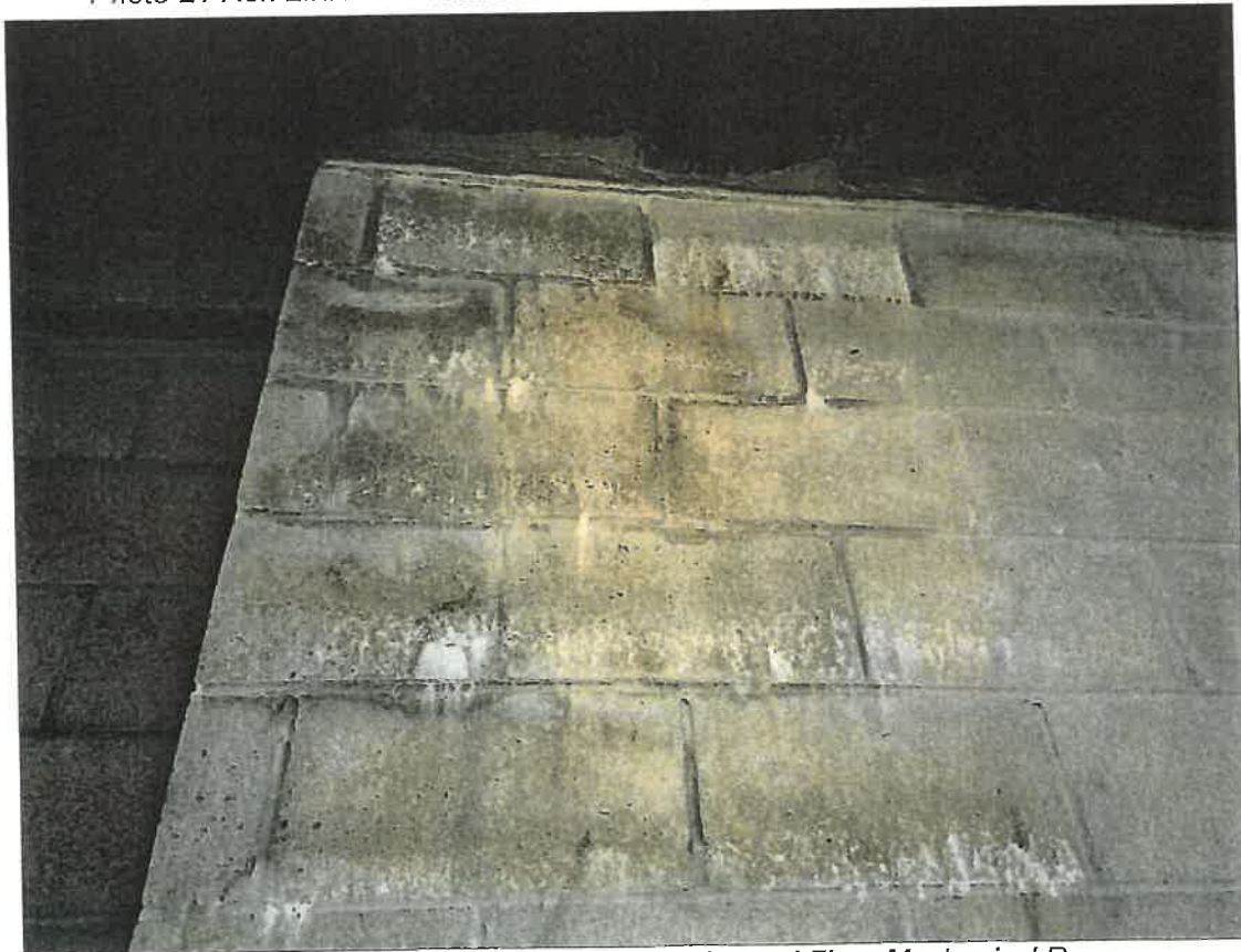
Photo 22 Ref: 2.2.5.1 – Wall Moisture, Ground Floor Mechanical Room
