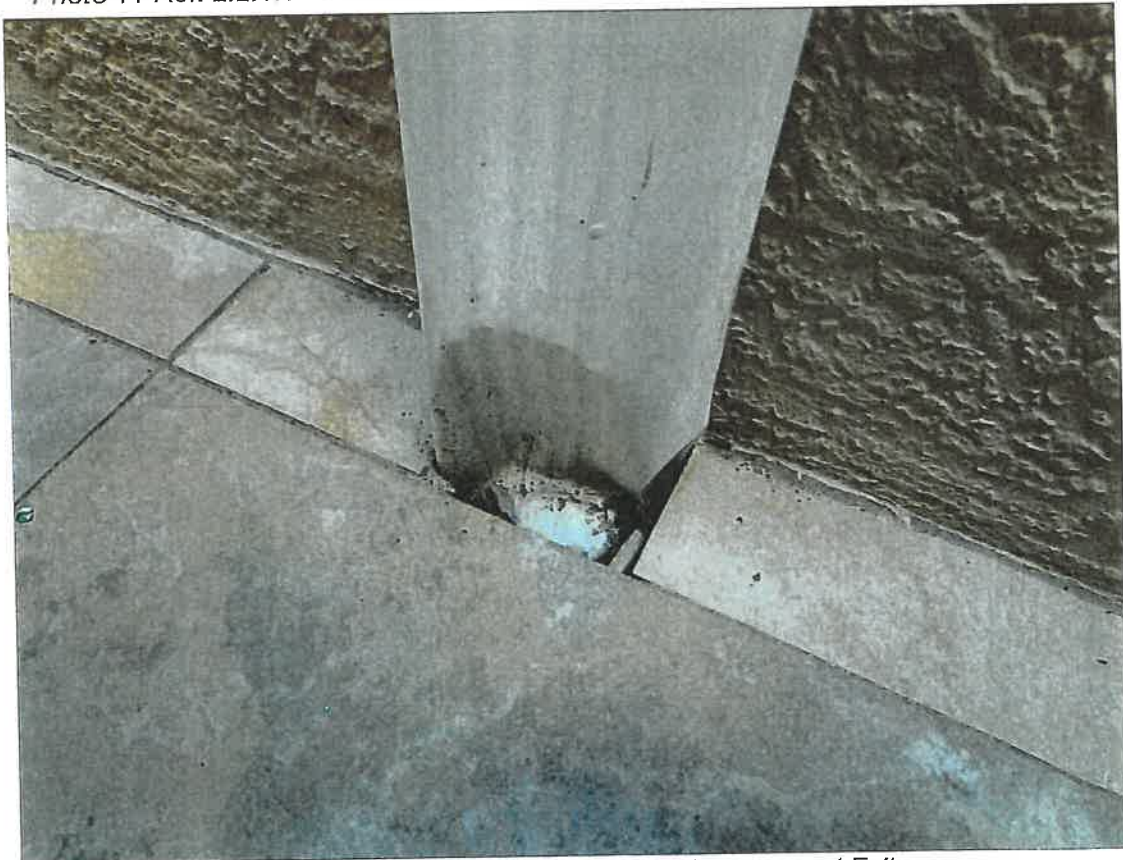
Photo 12 Ref: 2.2.2.1 – Crumpled Downspout Exit
