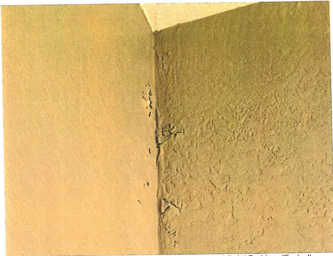
Photo 35 Ref: 2.2.7.2 – Stair Tower Moisture-Behind-Paint Problem (Typical)
