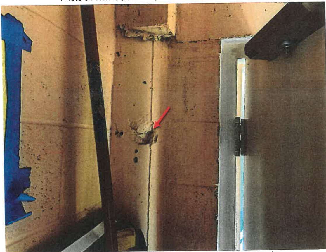
Photo 02 Ref: 2.1.1.1 – Spalled Column in Janitor Closet
