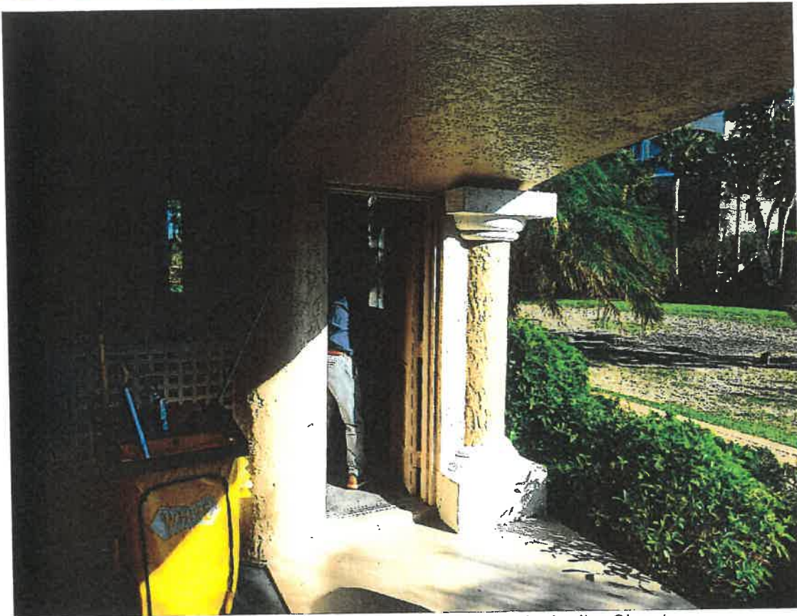
Photo 01 Ref: 2.1.1.1 – Spalled Column in Janitor Closet
