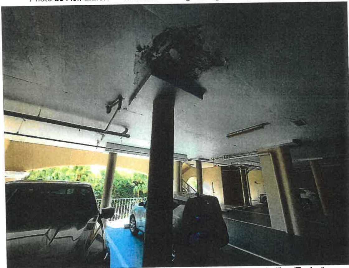
Photo 26 Ref: 2.2.6.1 – Moisture Coming Through Garage Ceiling (Typical)
