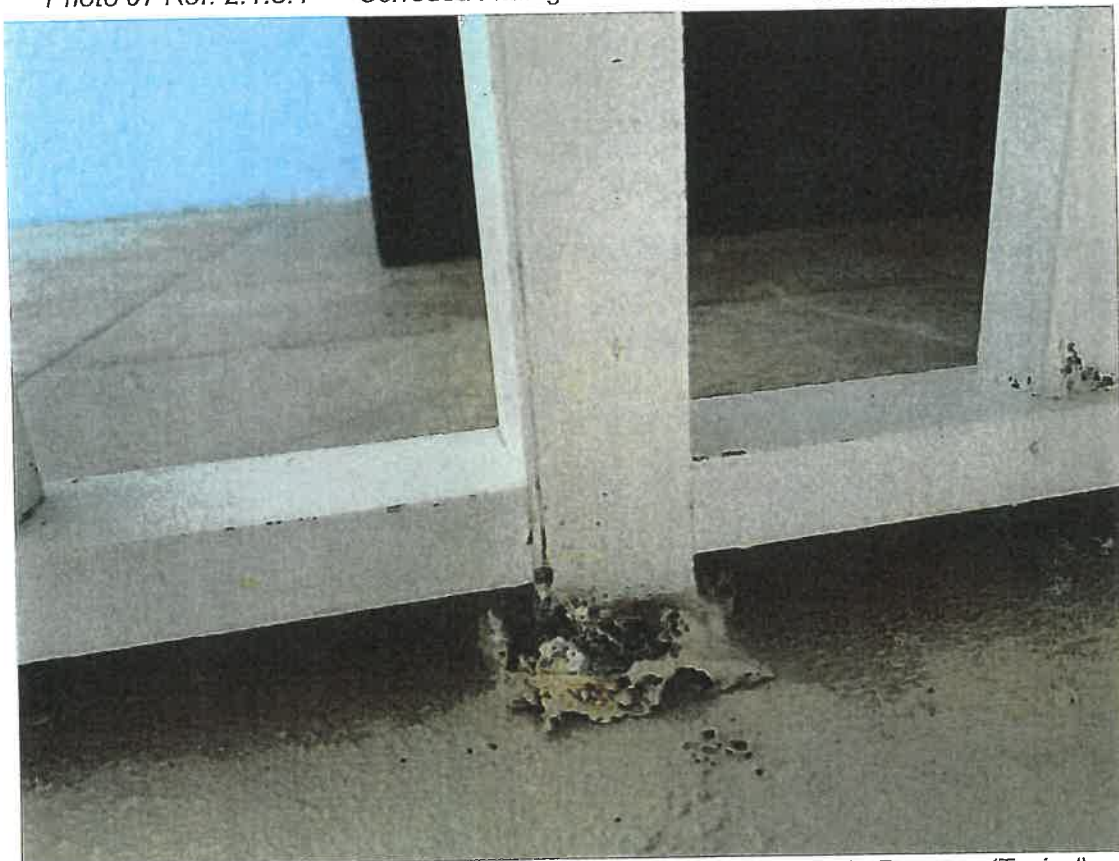
Photo 08 Ref: 2.1.3.1 – Corroded Railing Fasteners w/ Concrete Damage (Typical)
