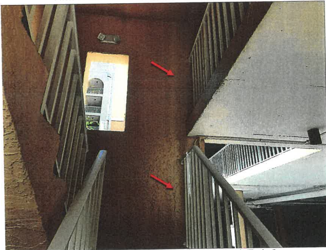
Photo 30 Ref: 2.2.7.1 – Stair Tower Settling Crack (Typical)
