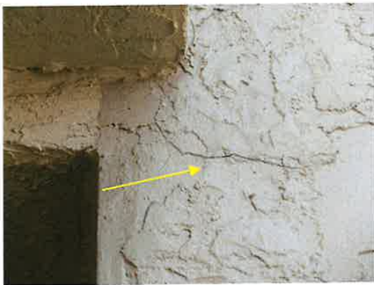
View of concrete distress along a wall.
