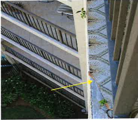
View of delaminated tile with vegetation growth along unit balcony deck edge.
