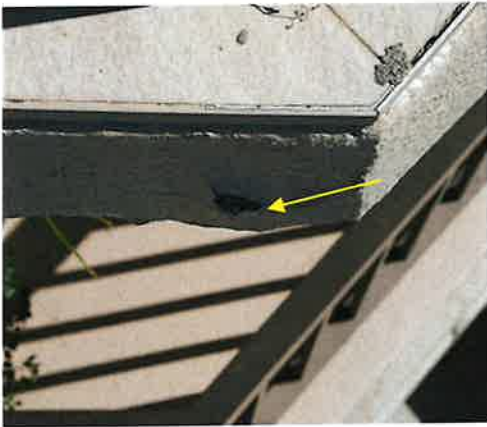
View of distressed concrete along unit balcony deck edge.
