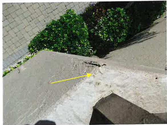
View of typical delaminated stucco.
