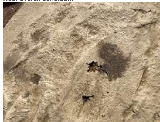
Peeling on the waterproofing.
