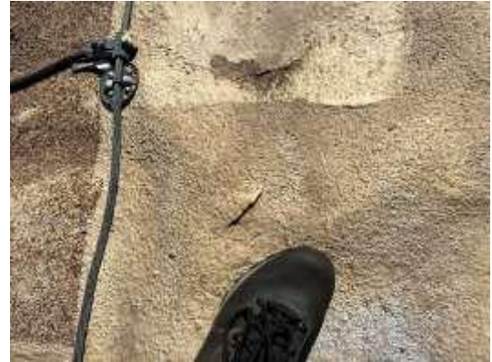
Cuts on the waterproofing.
