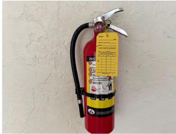
VIEW OF FIRE EXTINGUISHER
