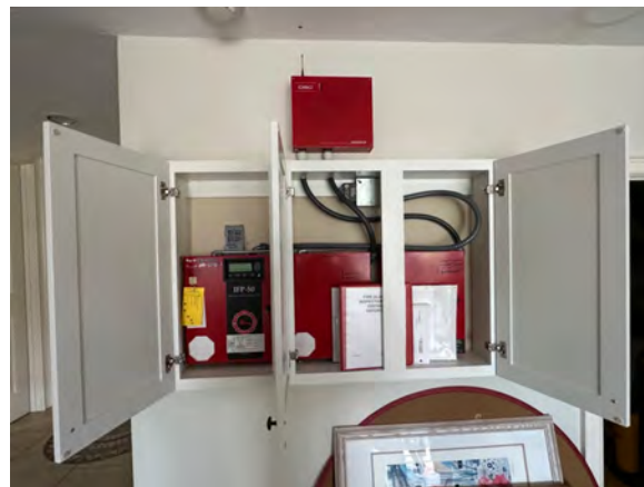
VIEW OF FIRE ALARM CONTROL PANEL
