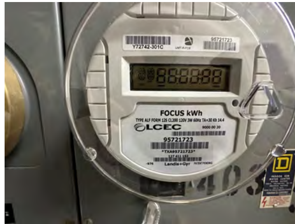
VIEW OF ELECTRICAL EQUIPMENT
