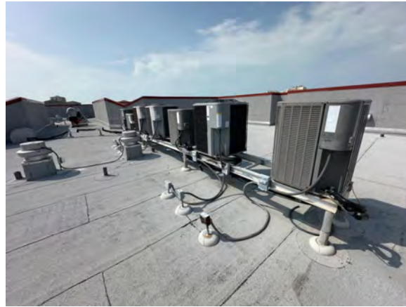
VIEW OF HVAC EQUIPMENT
