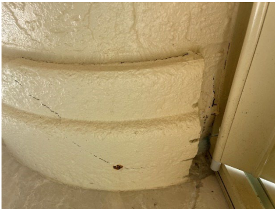
Cracked arch accent at column base. (Unit 1401)
