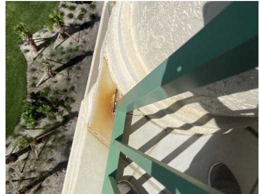
Stain on deck at post pocket. (Unit 701)
