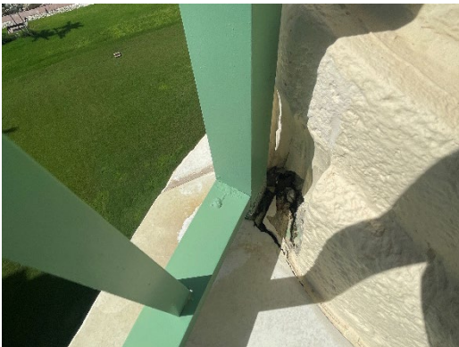
Staining between rail and column (Unit 701)
