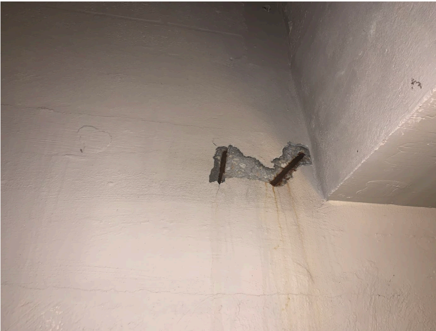
Column “spalling” at the staircase landing of the 18 th -floor. (Stair #1)
