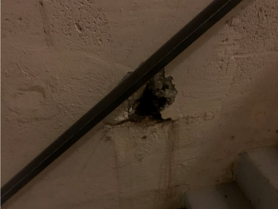
Column “spalling” at the staircase between the 18 th -floor and roof level.
