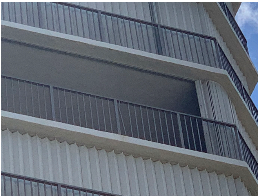
Damage picket at the unit #1101 balcony railing.
