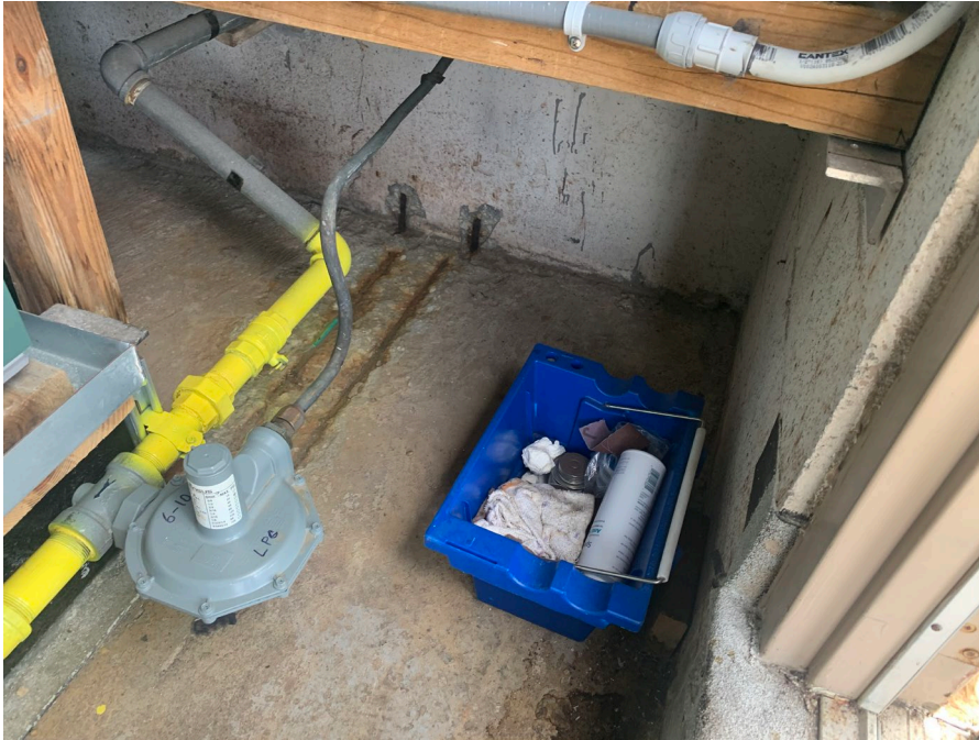
Floor “spalling” at the boiler room. (Roof)
