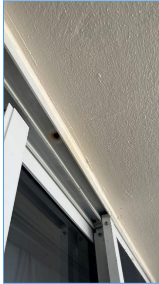
Figure 4: Typical corroded sliding glass door fastener (unit 202)
