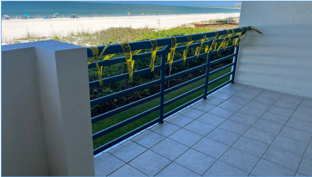
Figure 2: Balcony railing significantly deflecting when loaded at unit 103
