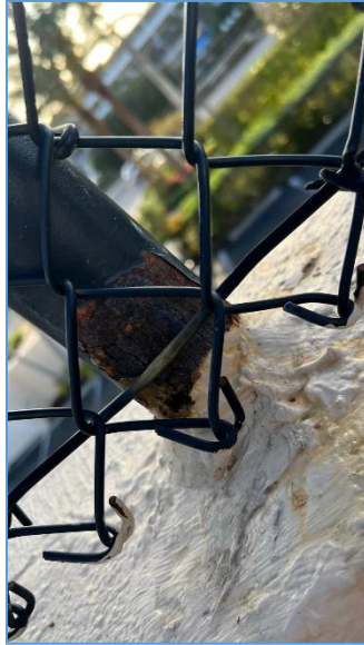
Figure 13: Tennis court chainlink post typical corrosion
