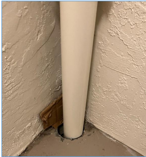
Figure 15: Pipe stand clamp missing (typical condition)
