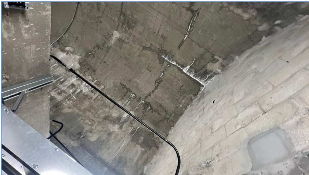
Figure 18: Rooftop elevator ceiling efflorescence to be removed and monitored
