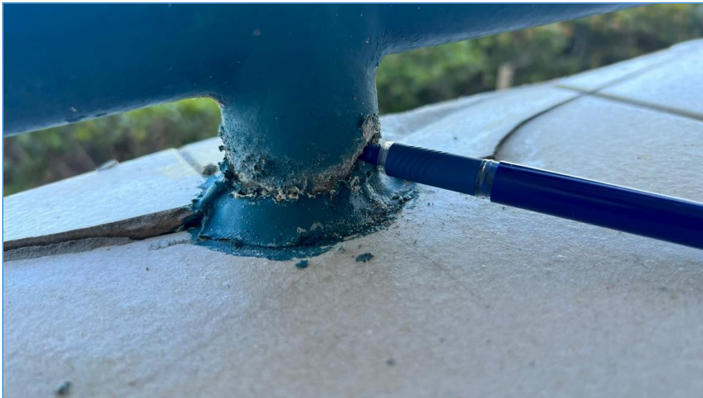
Figure 3: Balcony railing post corrosion at unit 104
