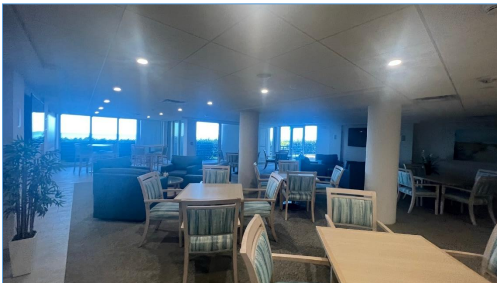
Figure 9: Card room interior finishes preventing visual examination of structural elements
