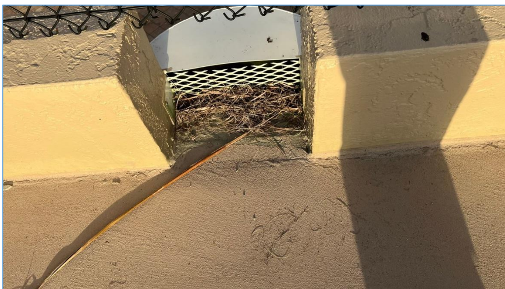
Figure 12: Tennis court scupper blocked debris
