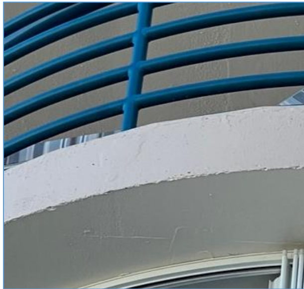
Figure 5: 203 concrete spall at slab edge coinciding with post pocket (typical)
