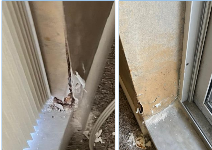
Figure 1: Cornerbead corrosion adjacent to original sliding glass doors at unit 306
