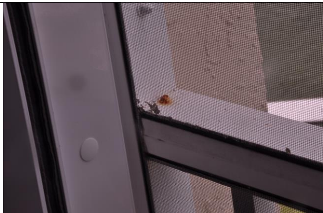
23. Unit 604, Building 4 – Rusty fasteners in Lanai area.
