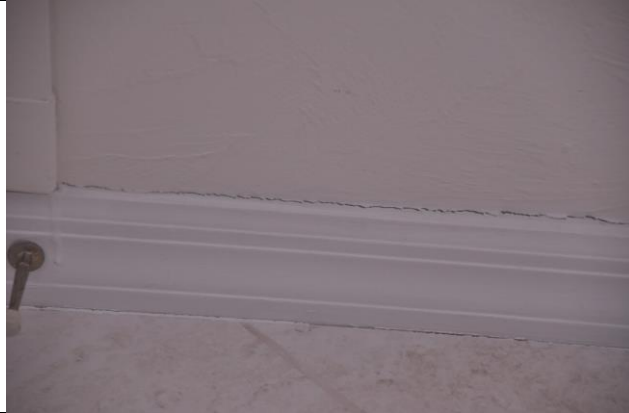
19. Unit 306, Building 4 – Cracks along baseboard.
