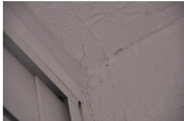
21. Unit 306, Building 4 – Cracks on Lanai ceiling.
