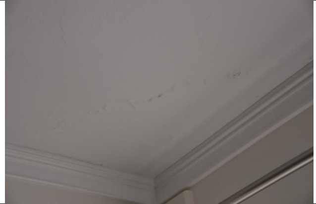
20. Unit 306, Building 4 – Cracks on ceiling.
