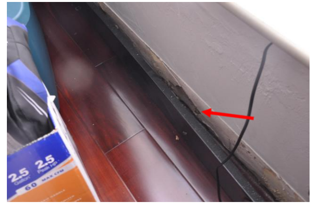
22. Unit 406, Building 4 – Moisture causes peeling on baseboards, elements disengaging from walls and ceiling.
