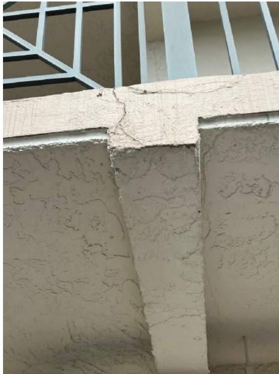
Figure 4: Hairline crack at concrete beam.
