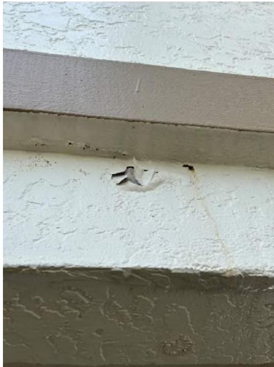
Figure 5: Hairline crack at slab edge and paint blister.
