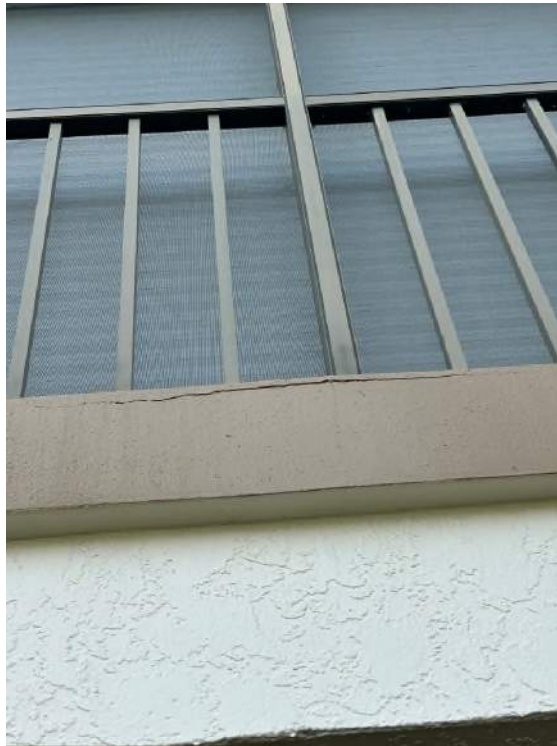
Figure 2: Hairline crack at slab edge.
