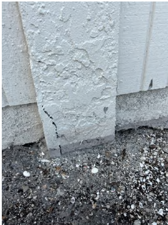
Figure 3: Hairline crack at column base.
