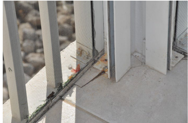
18. Unit 605 - Ceramic tile fracture – superficial damage - concentration of moisture & damage of steel angle
