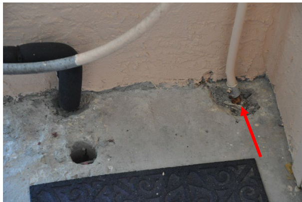
13. Water will concentrate and damage concrete. Prompt repair necessary. 7 th Floor Service Area
