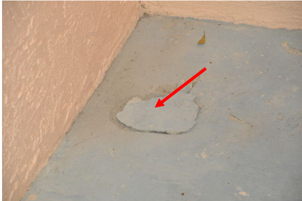
19. Concrete floor damage in service area 402
