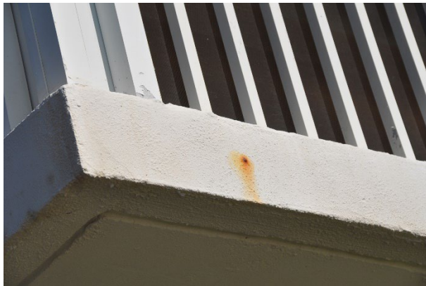
25. Corrosion of ferrous based element located very close to the concrete surface against ACI 318 codes. See next figure.
