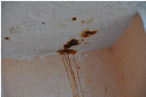
21. Corrosion effect in ceiling area of service space 302
