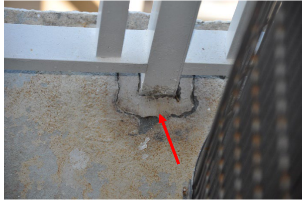
12. Minor maintenance issue that may lead to more important concerns if action does not take place promptly. Water will concentrate and percolate through to damage concrete reinforcement (Unit 702)
