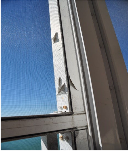
17. Improper use of materials and absence of maintenance – Unit 605. Structurally negligible.
