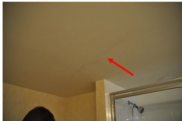
16. Watermark on ceiling in unit 605. Cause is only speculated but the damage cannot be precisely assessed by damage on surface.
