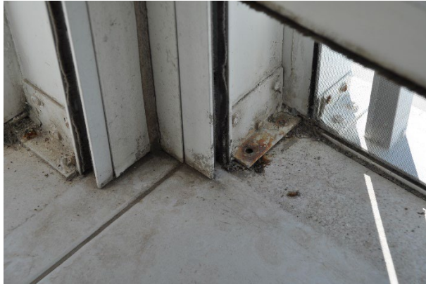
11. Typical maintenance issue of steel structural elements. (Unit 702)
