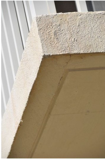
23. Maintenance will be required for such cracks. This can be injected with epoxy to prevent further expansion of the existing crack. See next figure.
