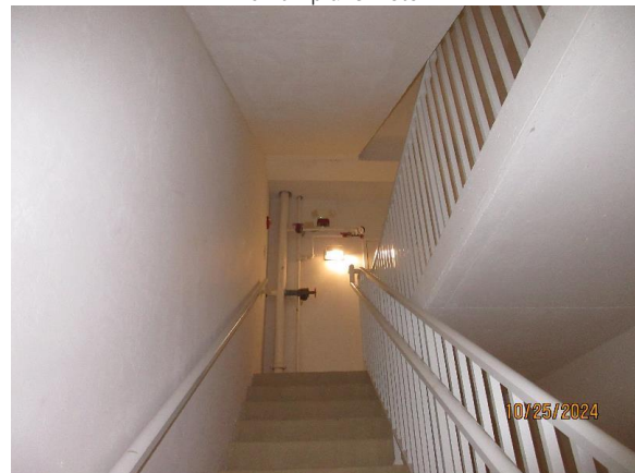
Fire Sprinkler Plumbing
