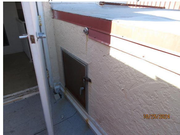
Corrosion Present at Ferrous Metal Fasteners
