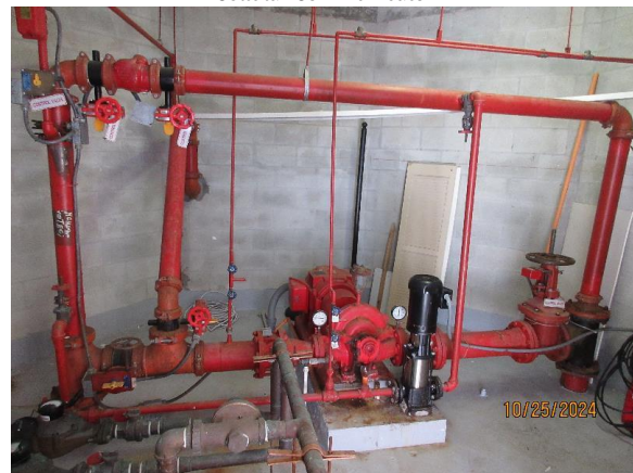
Fire Pump and Motor
