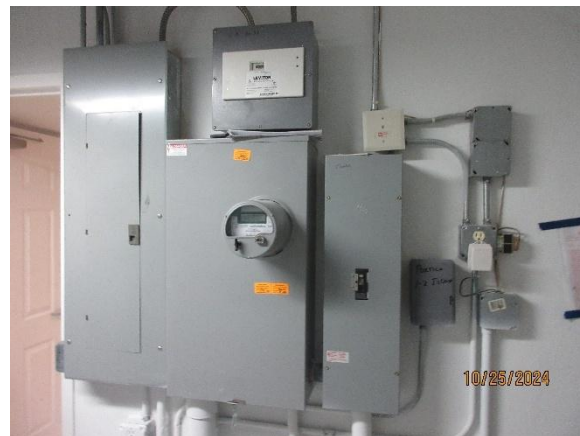
Typical House Meter and Panel
