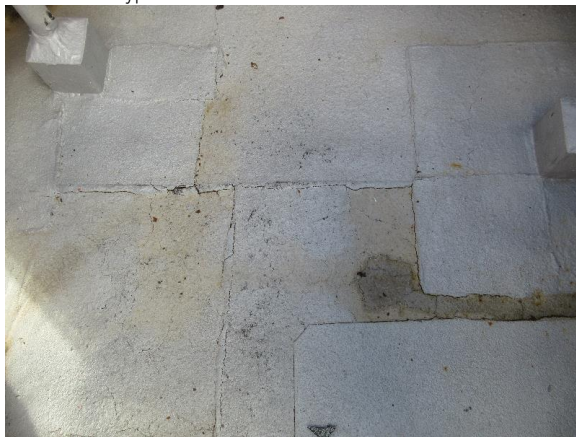
Cracking and UV Degradation at Seams
