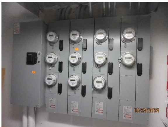
Typical Residential Electric Meter Bank
