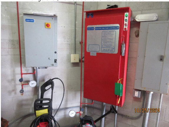
Fire Pump Controller
