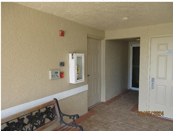
Extinguisher, Pull Station and Flasher/Sounder
