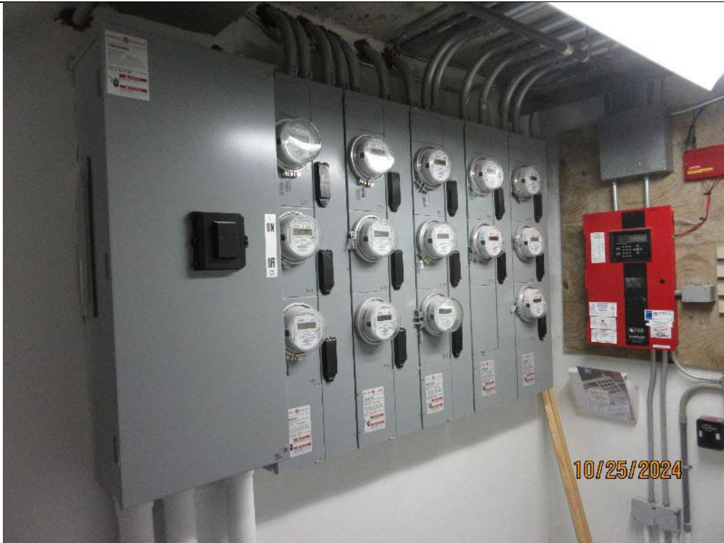
Photo 48. Typical Residential Electric Meter Bank
