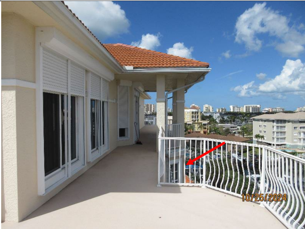
Photo 22. Penthouse Balcony Over Occupied Space
