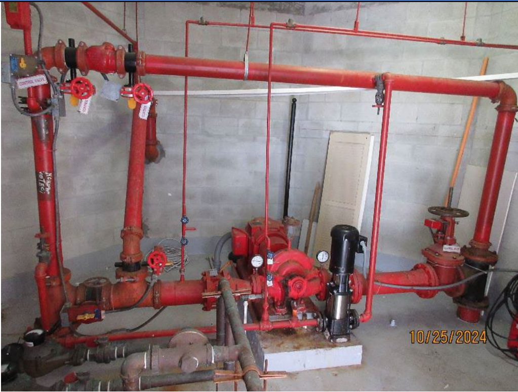
Photo 43. Typical Fire Pump and Motor
