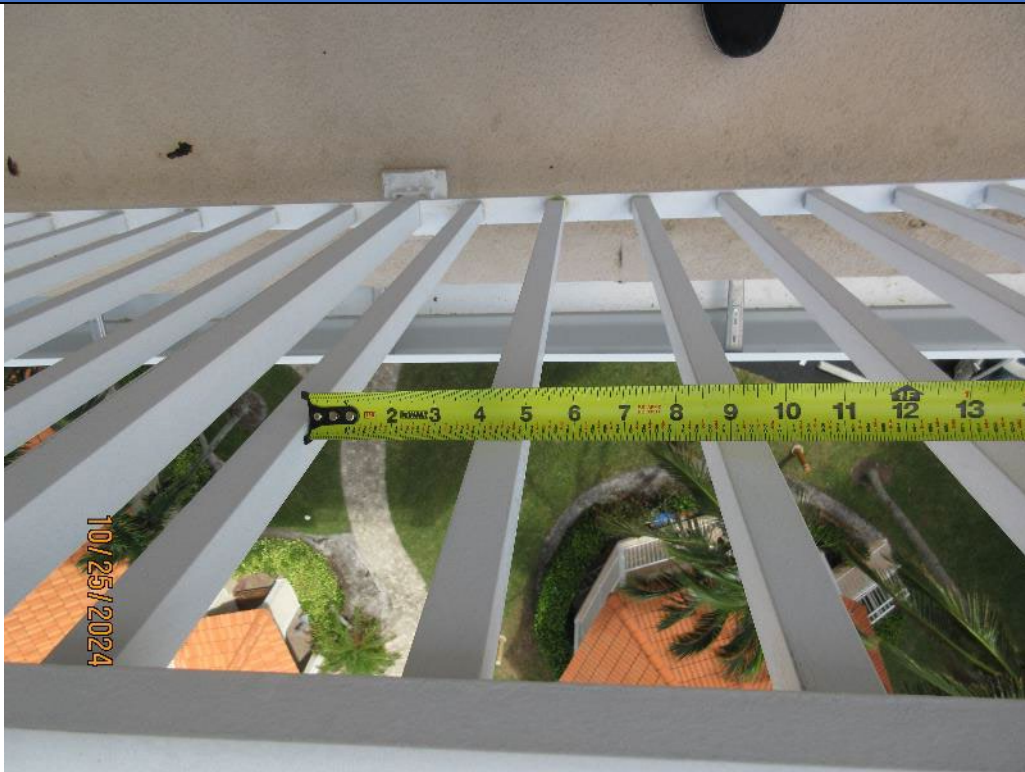
Photo 25. Typical Railing Picket Spacing Measured 4" or Less
