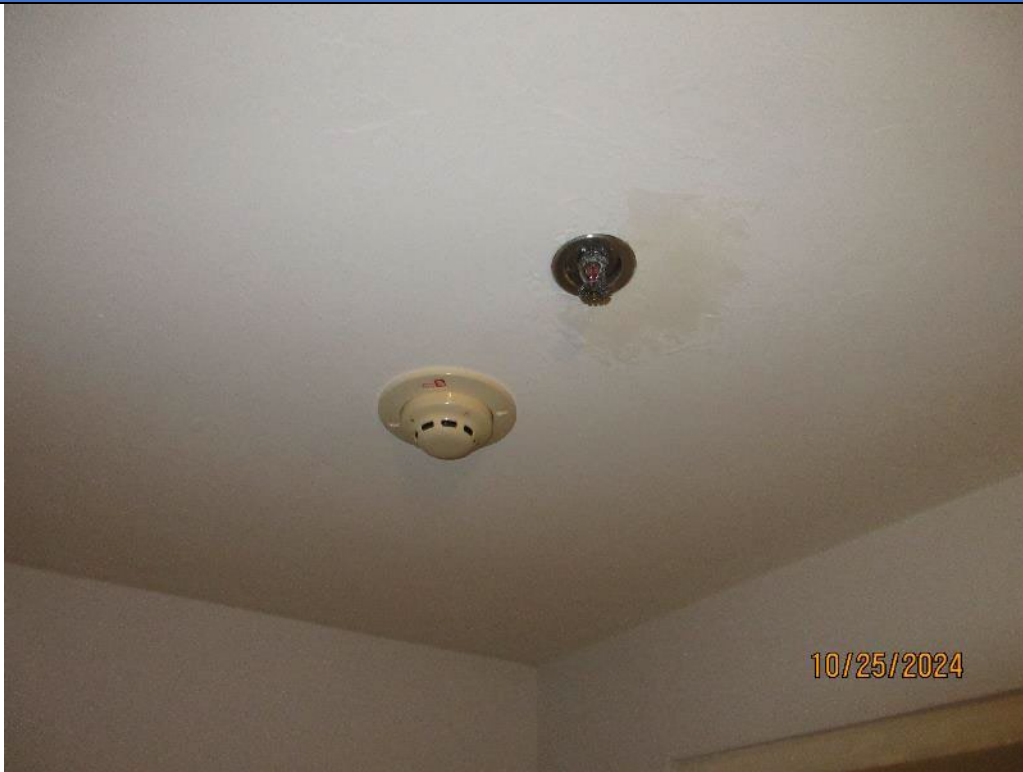
Photo 47. Fire Alarm Detection Device and Typical Sprinkler
