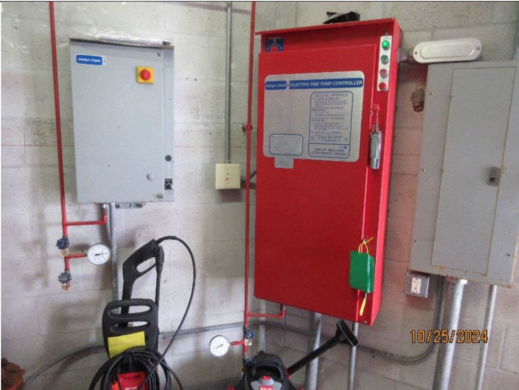
Photo 44. Fire Pump Controller
