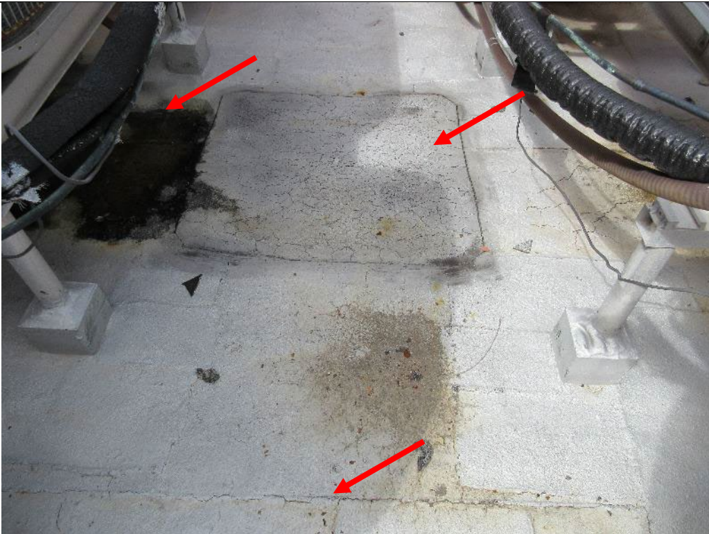
Photo 36. Modified Bituminous Roof Showing Signs Of Wear and Isolated Ponding
