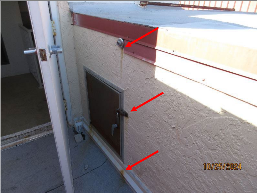
Photo 38. Corrosion at Ferrous Metal Fasteners
