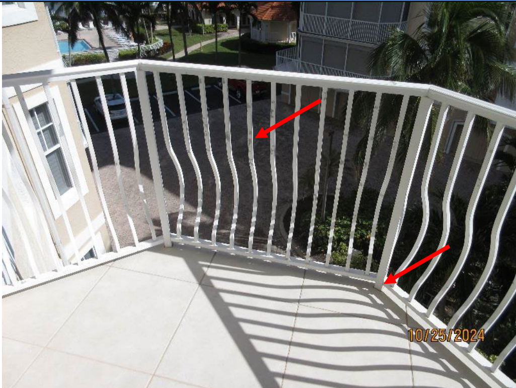
Photo 27. Railing Coating Exhibiting Signs of Wear and Typical Core Mounted Posts
