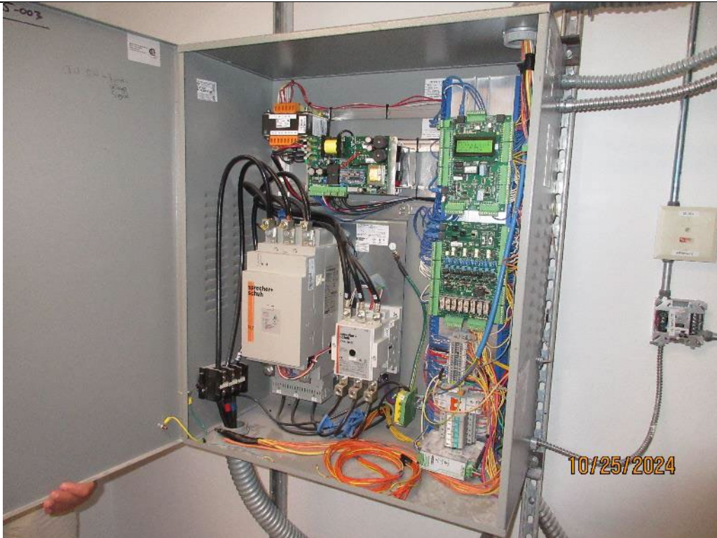
Photo 52. Typical Elevator Control Panel
