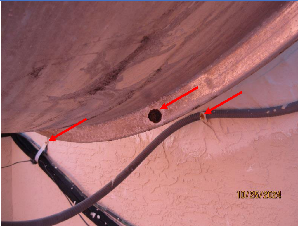
Photo 39. Corrosion at Ferrous Metal Fasteners
