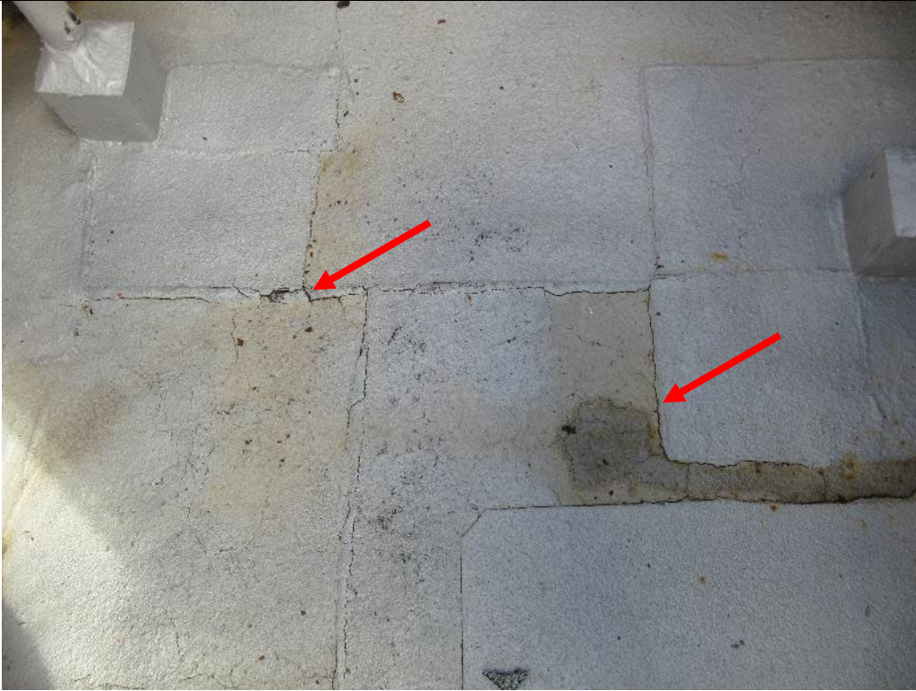
Photo 37. Modified Bituminous Roof Showing Signs Of Wear and Failed Prev Repairs
