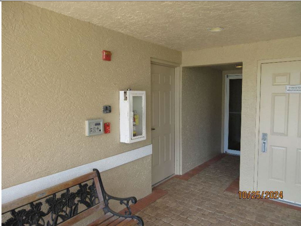
Photo 42. Typical Sounders, Flashers, Pull Station and Fire Extinguisher
