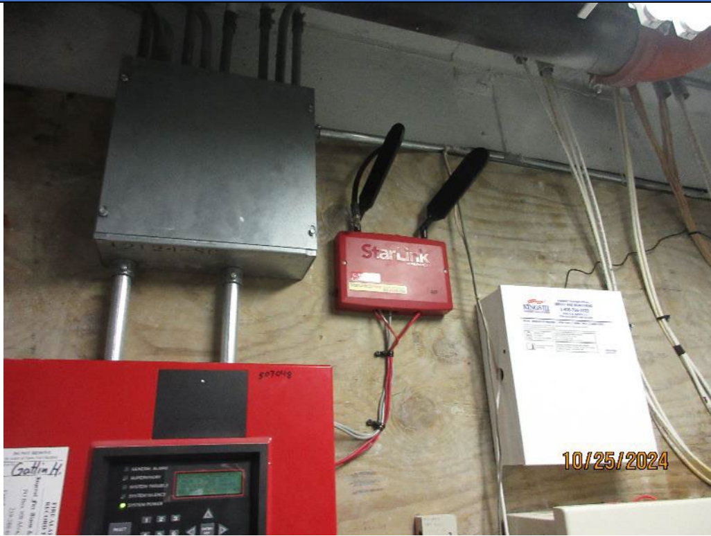
Photo 41. Cellular Commercial Fire Alarm and Emergency Communicators
