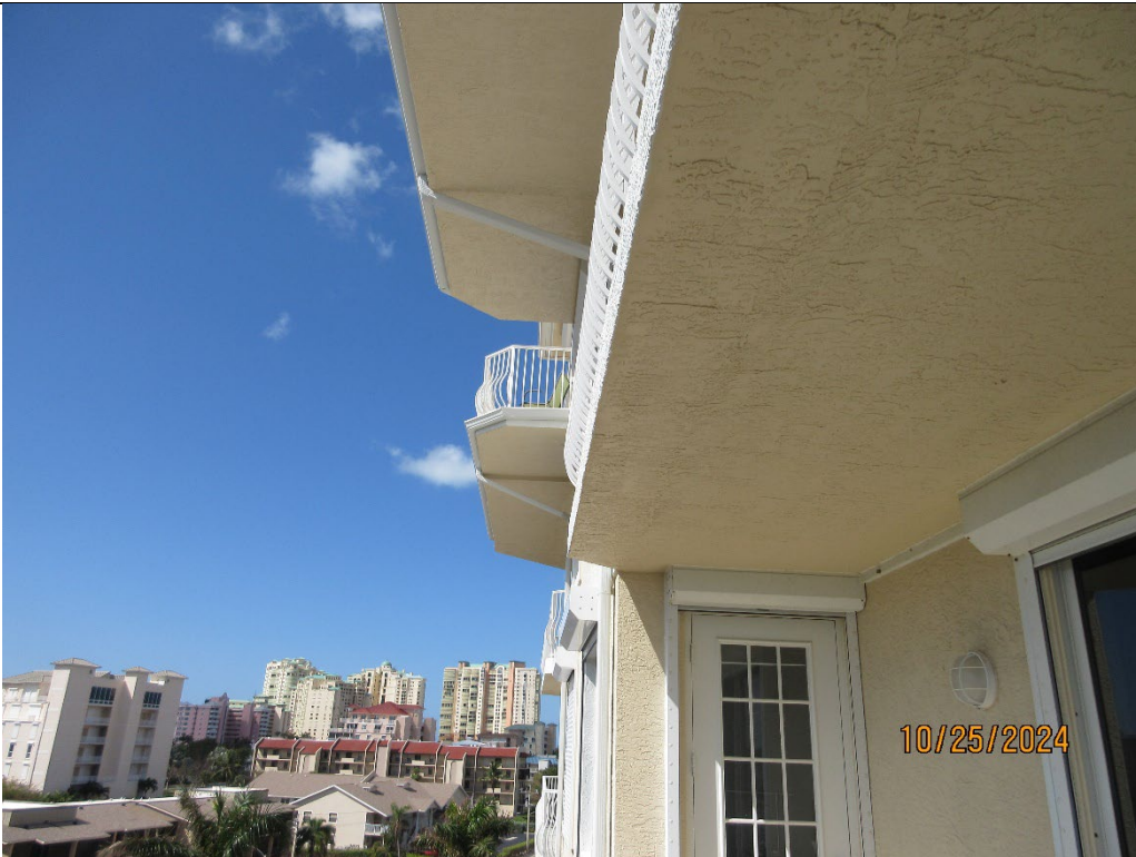
Photo 12. Typical Unit Balcony Ceiling Stucco with No Gutter
