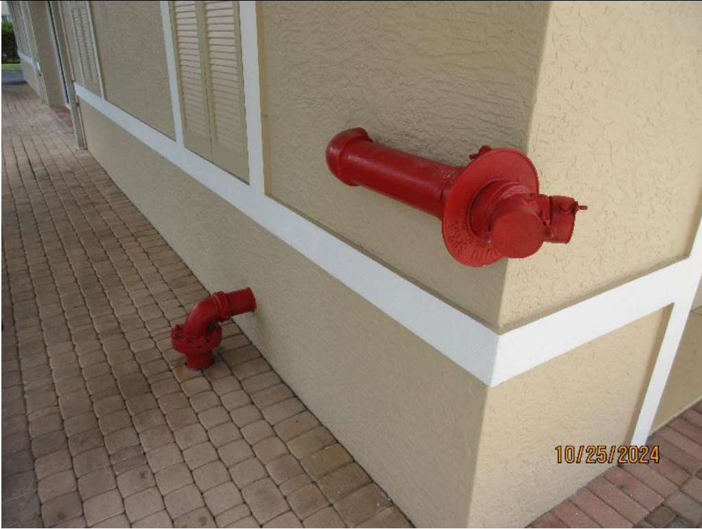
Photo 45. Fire Hose Stand Pipe
