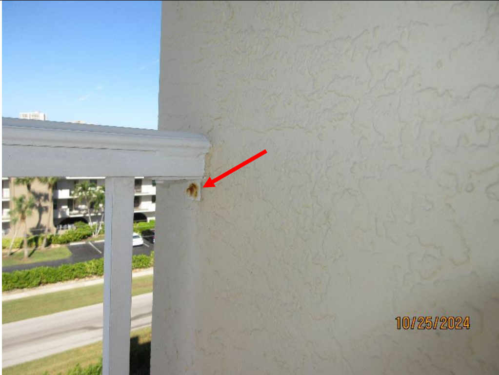
Photo 29. Corrosion at Select Railing Fasteners
