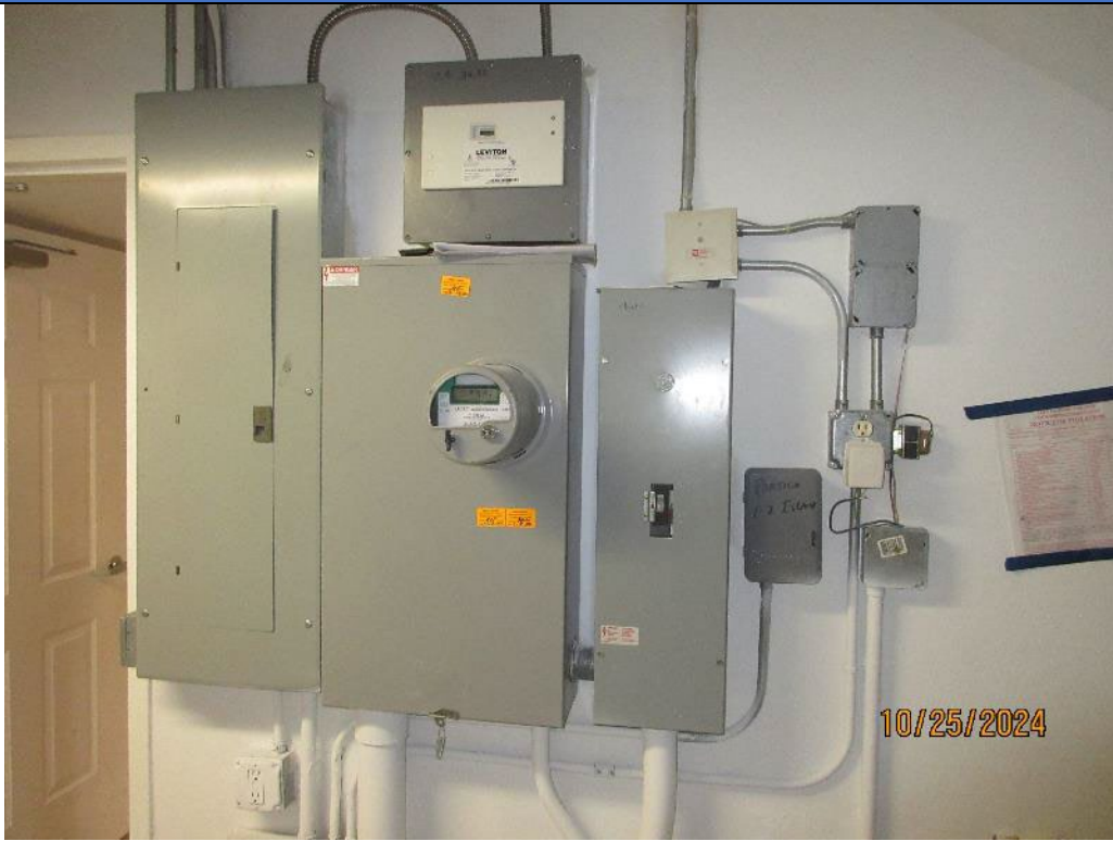
Photo 49. Typical House Power Meter and Panel
