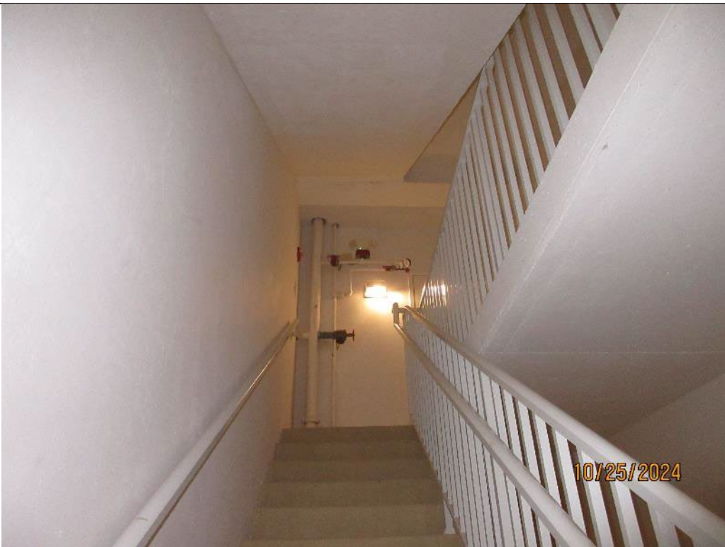
Photo 46. Sprinkler System Stair Tower Riser and Hose Connection
