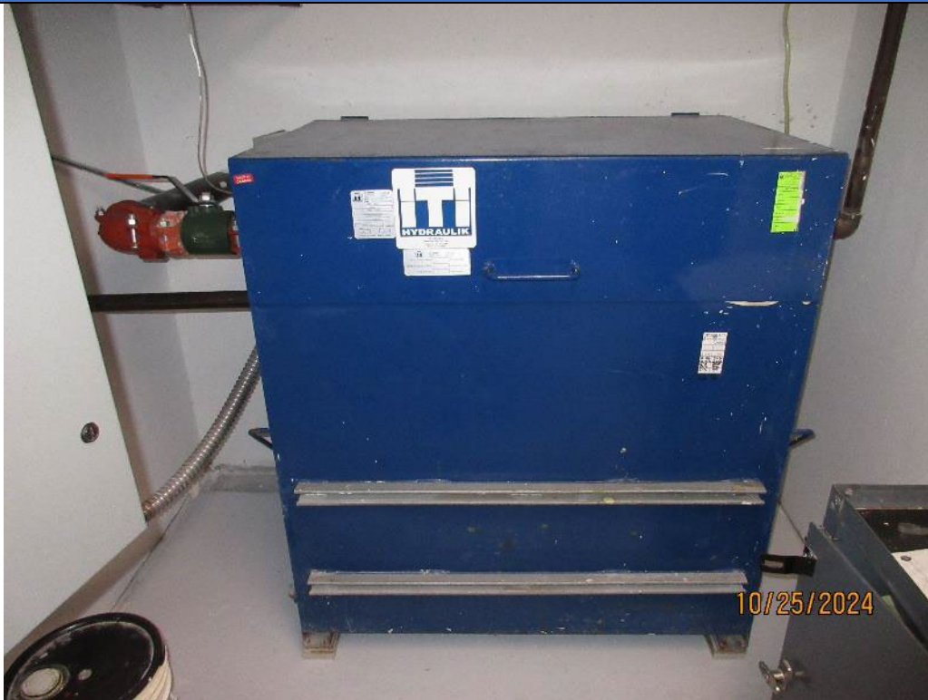
Photo 51. Typical Hydraulic Elevator Controller
