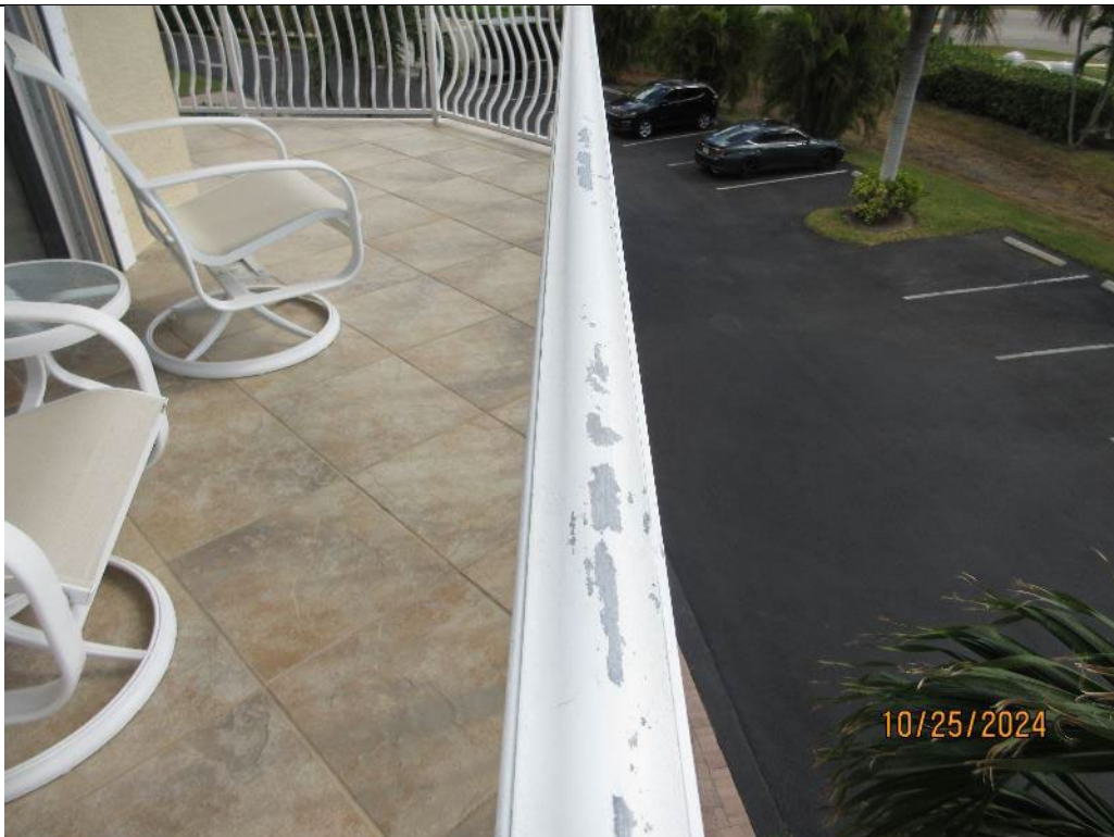
Photo 26. Railing Coating Exhibiting Signs of Wear
