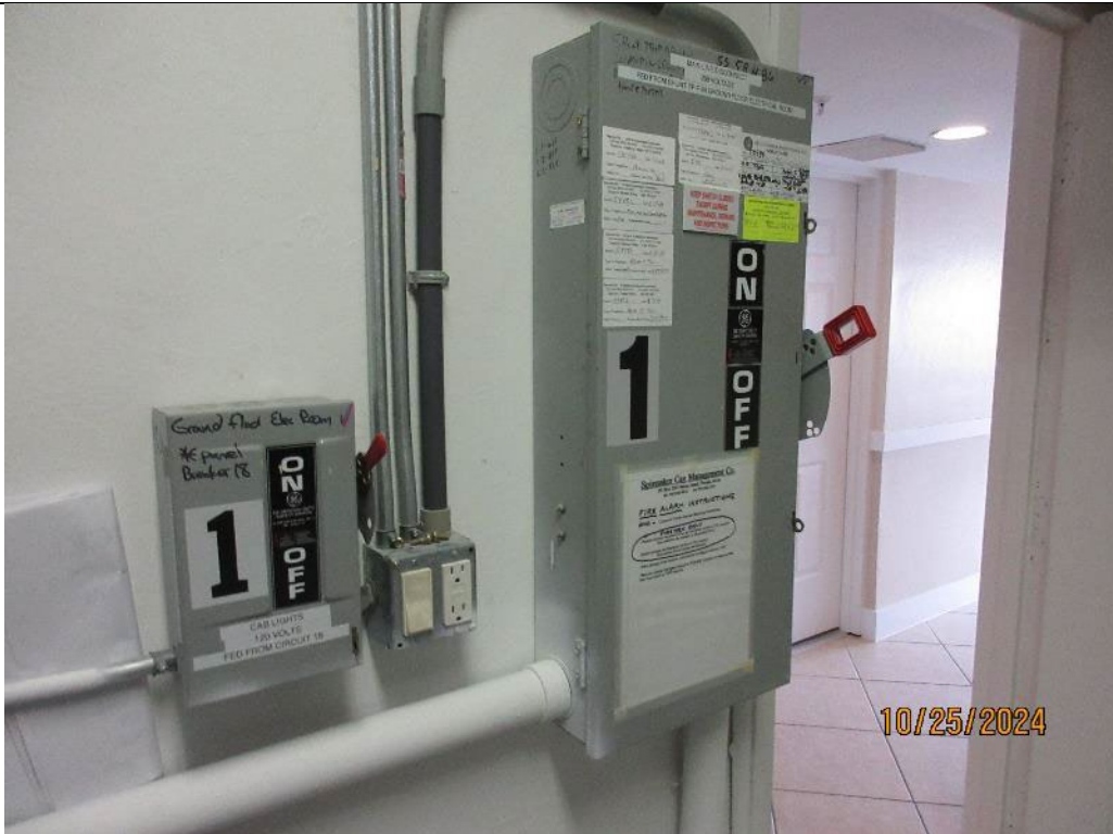
Photo 50. Typical Emergency Shut Off
