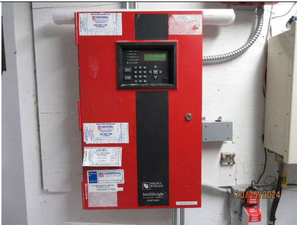
Photo 40. Typical Building Addressable Fire Alarm Control Panel
