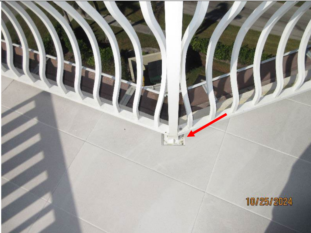
Photo 28. Base Plate Mounted Railing Post
