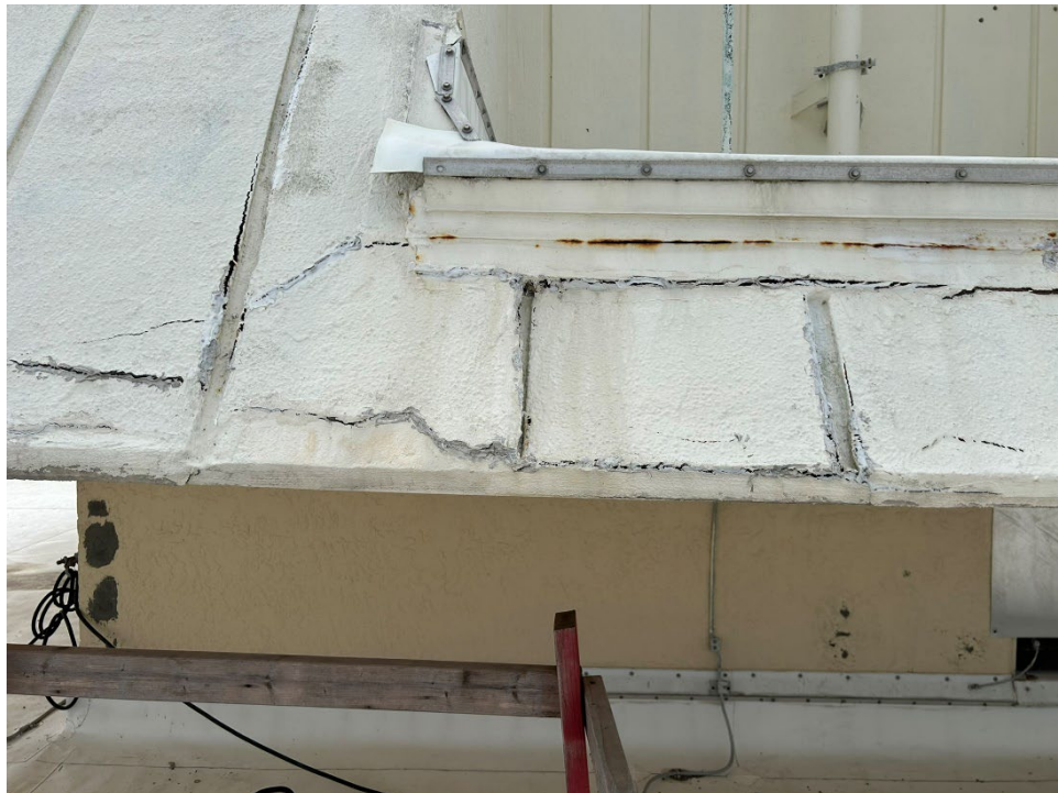
6. View of the cladding and failing finishes on the roof.
