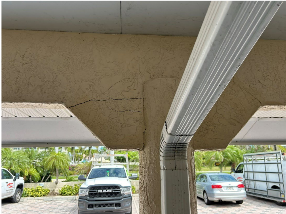
14. The observed cracks at the shear caps are indicative of a shear failure; therefore, we recommend the stucco be removed to determine the extent of the structural damage.
