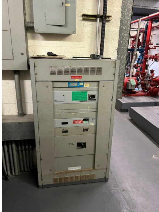
19. An Example of the electrical components at the common area.
