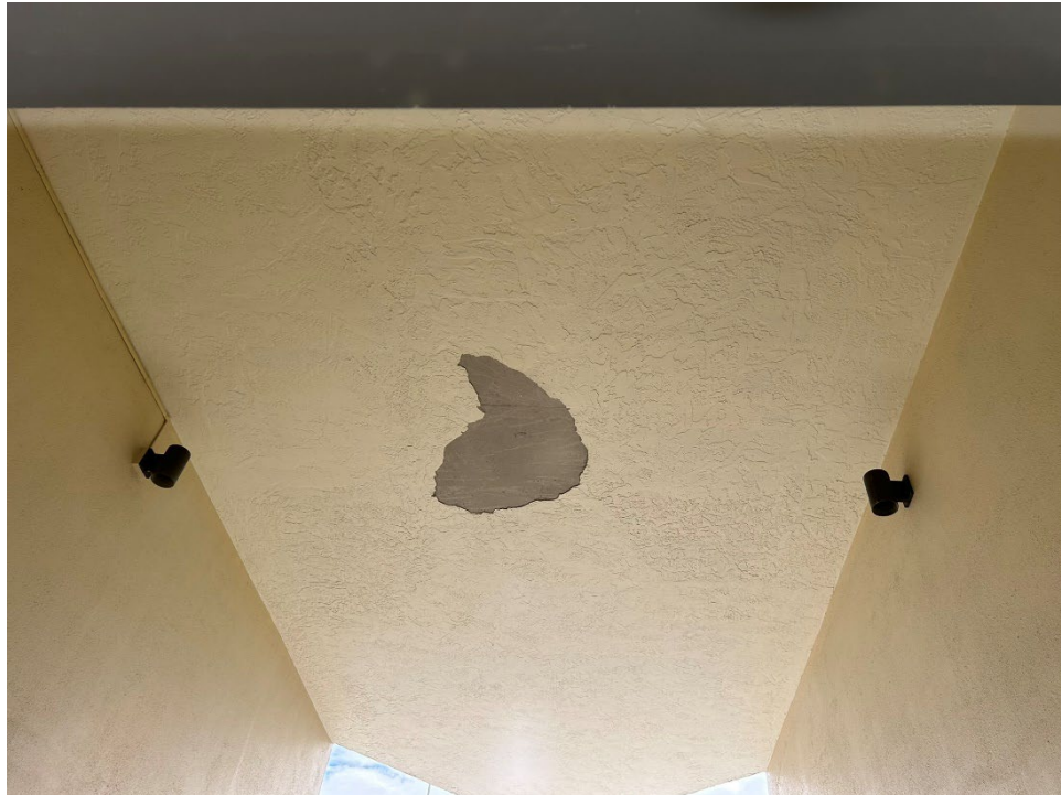
8. View of the observed delamination on the stucco.
