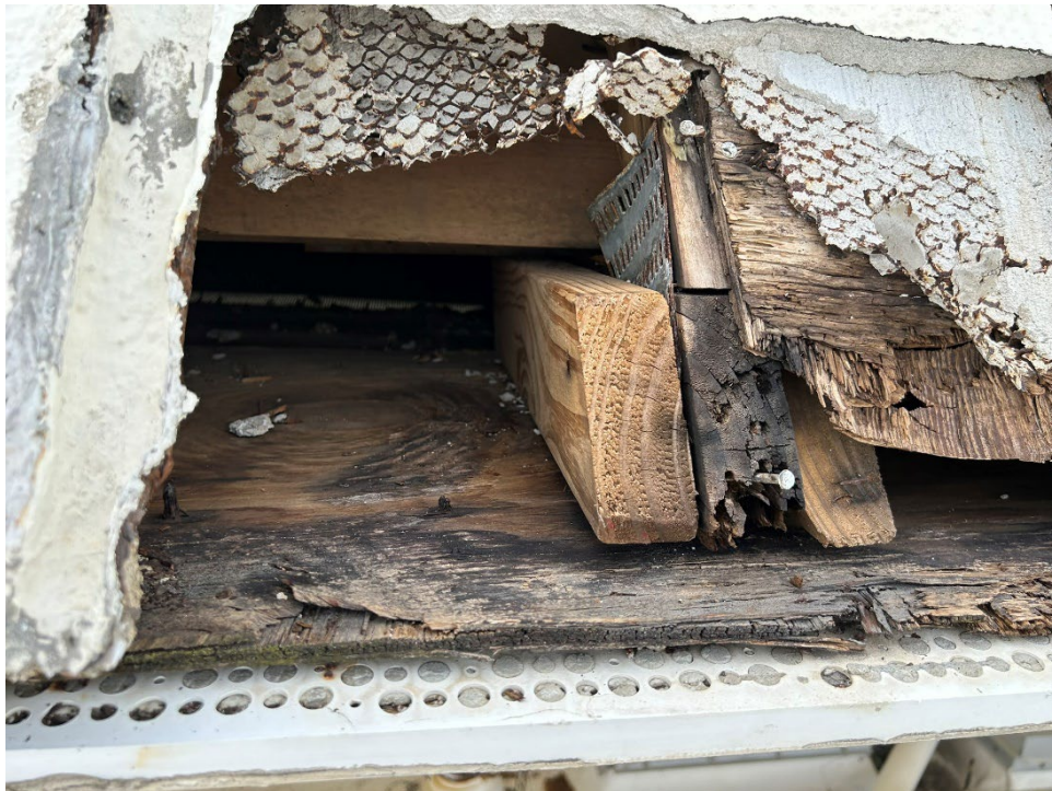
4. View of the observed water damage impacting the wood framing and sheathing of the middle roof section.
