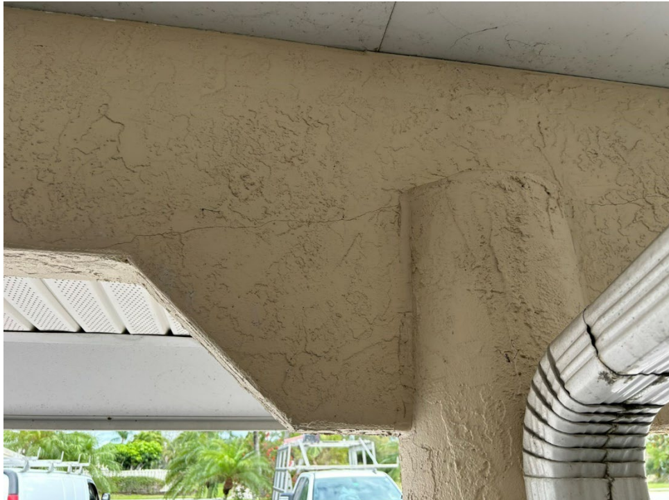
16. View of the additional shear failure cracks at the shear caps.
