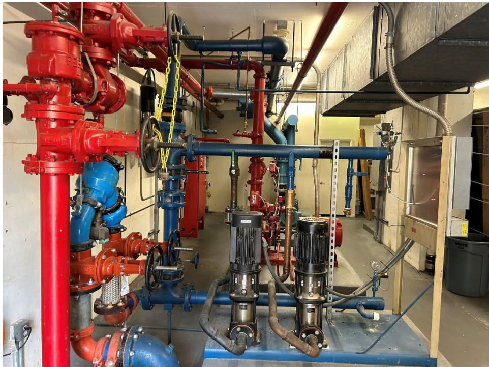
18. View of the fire pumps.
