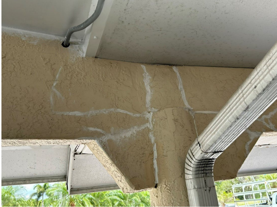
13. View of the observed cracks that have been repaired.
