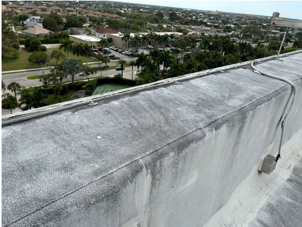
5. View of the failing joint sealant at the parapet walls.
