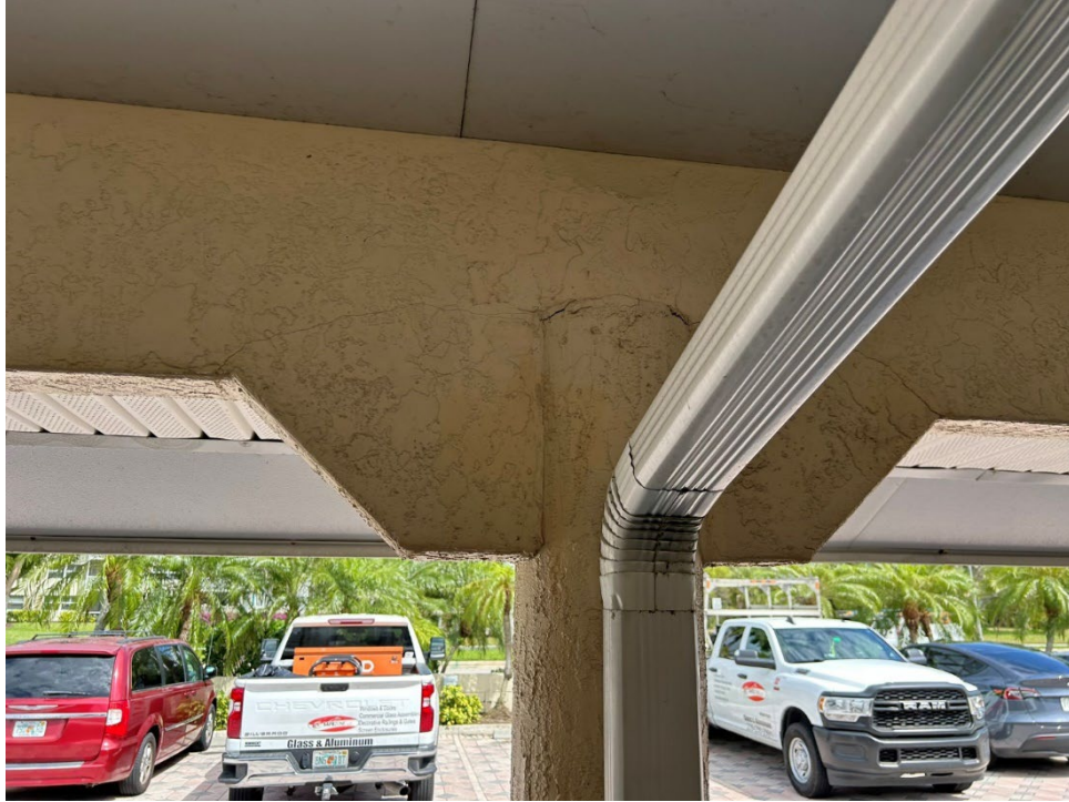
15. View of the additional shear failure cracks at the shear caps.
