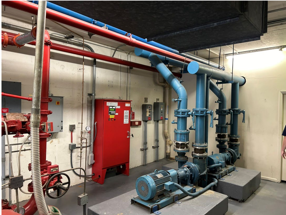
17. View of the domestic water pumps.
