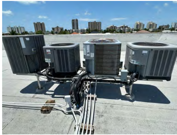
VIEW OF HVAC EQUIPMENT
