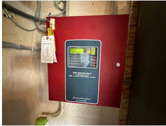
VIEW OF FIRE ALARM PANEL
