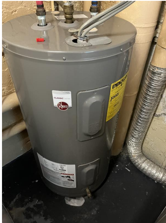
View of typical potable system components at subject site.
