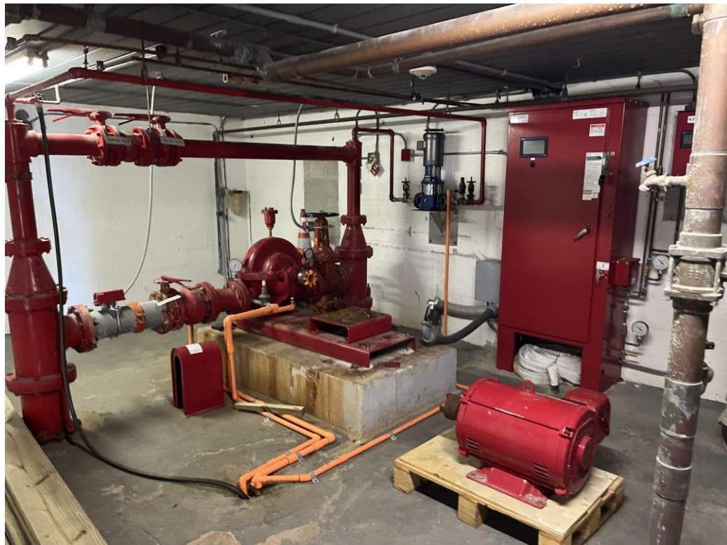
View of typical fire pump and related fire system equipment at subject site.
