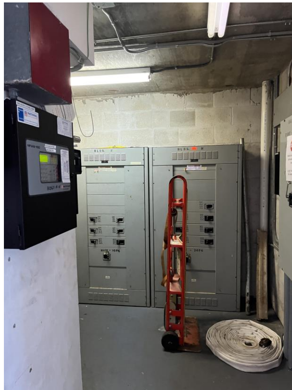
View of typical electrical equipment at subject site.
