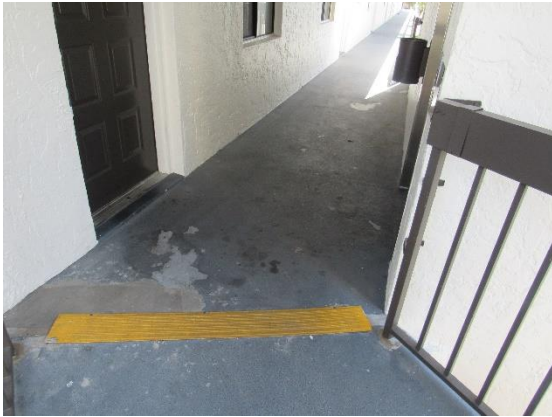
View of coating failure on breezeway.
