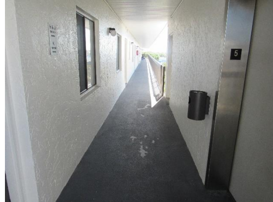
View of coating failure on breezeway.
